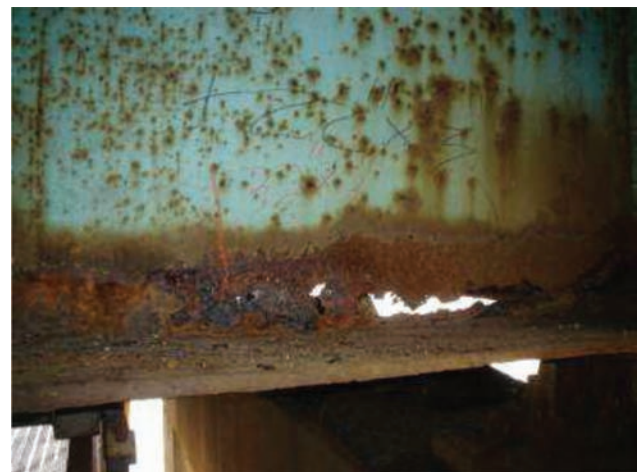
Figure F6.1 Loss of section on steel girder due to corrosion (Zaffetti, 2010).
