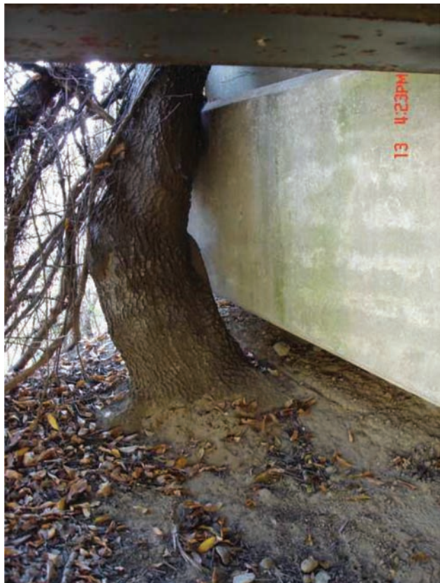
Figure G13.1 Trees around structure elements are a significant hazard (GDOT, 2012).
