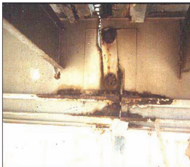
Figure F10.2 Typical pack-rust formation at pin and hanger connection (WisDOT, 2011).
