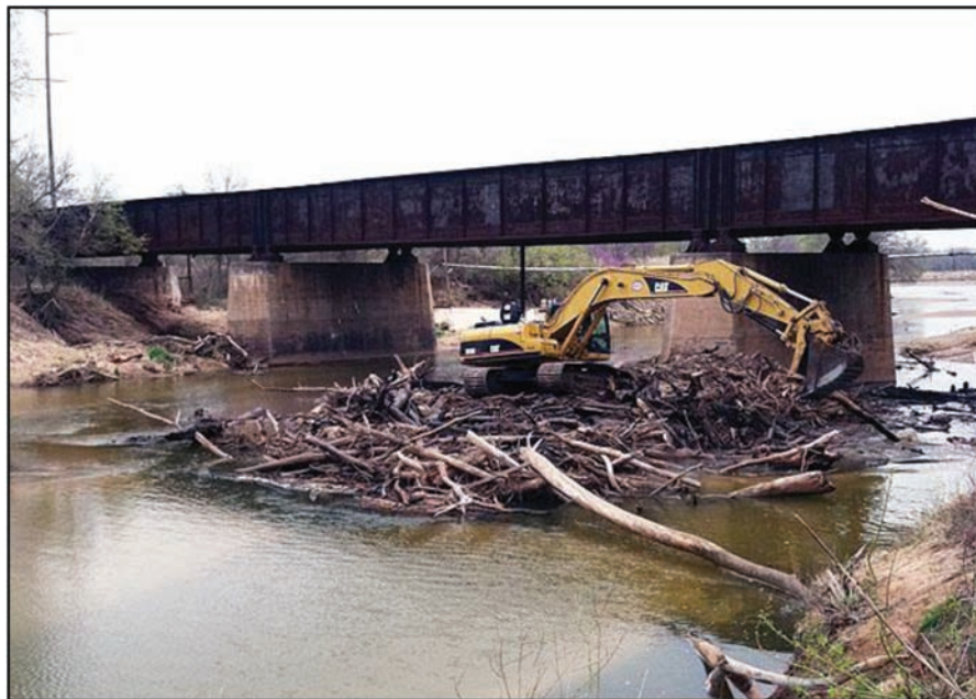
Figure F9.4 Excavator removes debris that has built up around a bridge pier (Hulcher Services, 2014).
