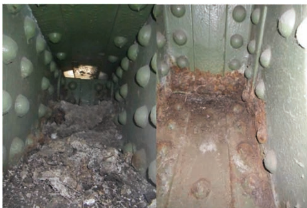
Figure F6.3 Interior of lower chord from truss. Before (left) and after (right) cleaning and washing (Berman et al., 2013).
