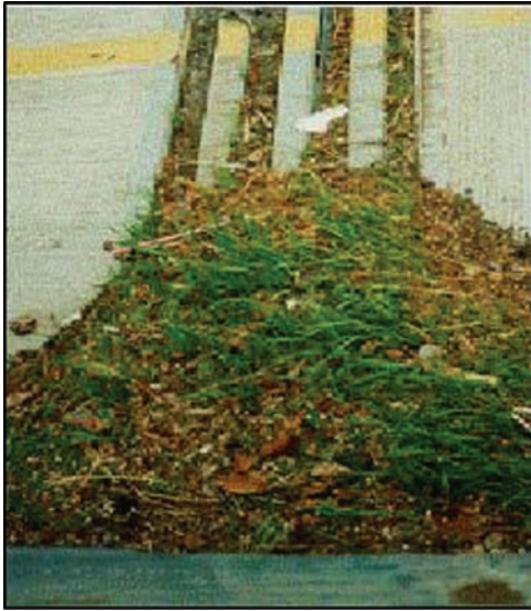
Figure F3.1 Accumulation of debris in a bridge expansion joint (Kaczinski, 2010).
