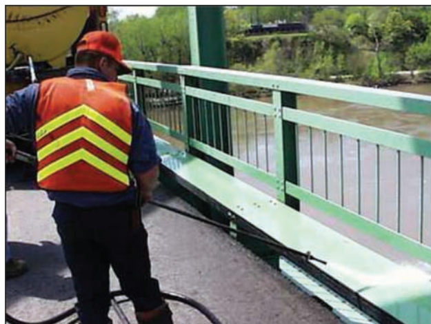
Figure G2.2 Flushing helps to remove dirt and debris from curb outlets and pipe drains (MoDOT, n.d.).
