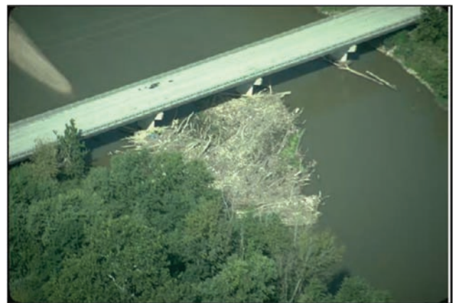
Figure F9.1 Blockage of a 27-meter span over White River in Paragon, Indiana, September 25, 1992 (Diehl, 1997).
