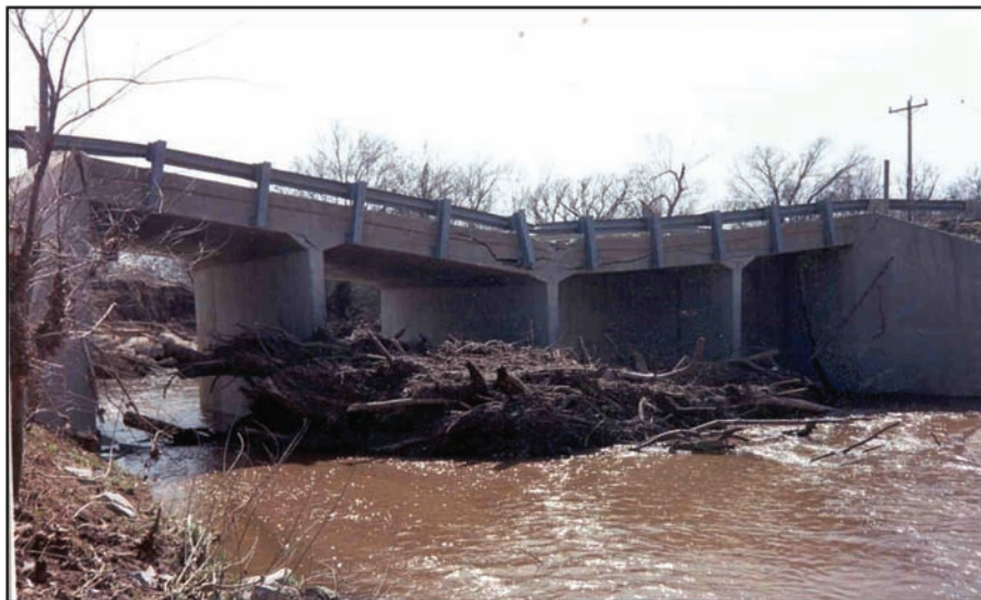
Figure F9.3 Failure of a bridge located in Oklahoma due to debris accumulation (Bradley et al., 2005).
