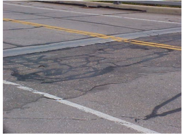
Figure F5.4 Damaged approach slab showing surface cracks (Abu-Hejleh et al., 2006).
