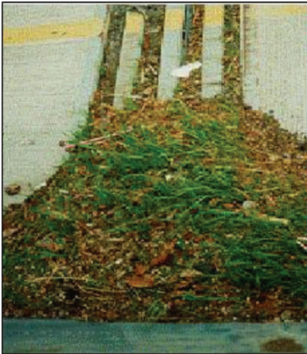
Figure G6.1 Accumulation of debris in a bridge expansion joint (Kaczinski, 2010).
