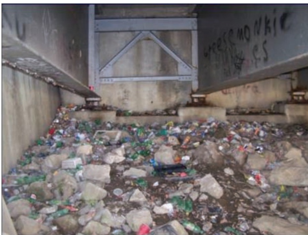
Figure G11.1 Debris, dirt, and waste can be found surrounding superstructure elements (Steele, 2013).
