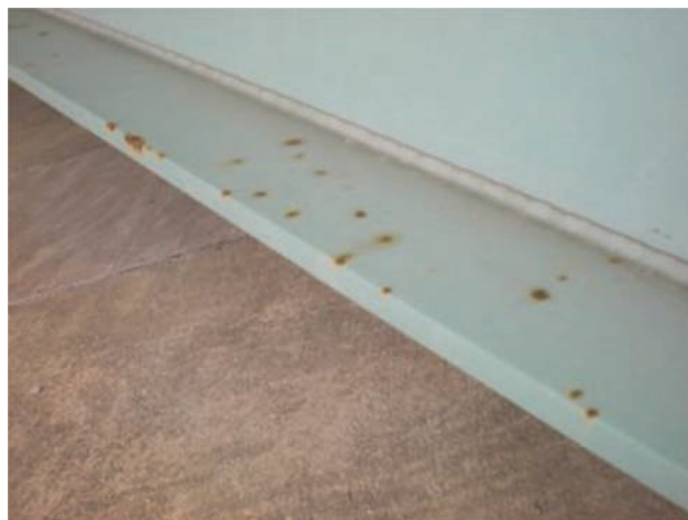
Figure G12.1 Steel girder candidate for spot painting (MoDOT, 2010).
