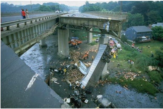
Figure F10.3 A suspended span collapsed at the Mianus River Bridge in Greenwich, Connecticut due to pin and hanger failure (Morgan, 2015).
