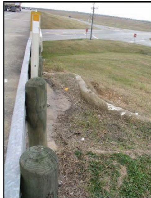
Figure F5.5 Drainage system obstructed by accumulation of weeds and debris (Jayawickrama et al., 2005).
