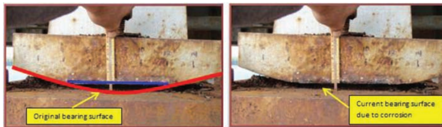
Figure F4.1 Steel bearing corroded, which has reduced its ability for displacement and rotations (Balassone, 2010).
