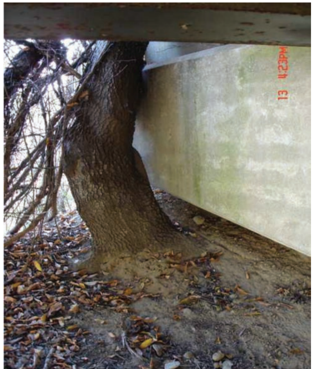
Figure F8.1 Interference of tree with bridge structure (GDOT, 2012).
