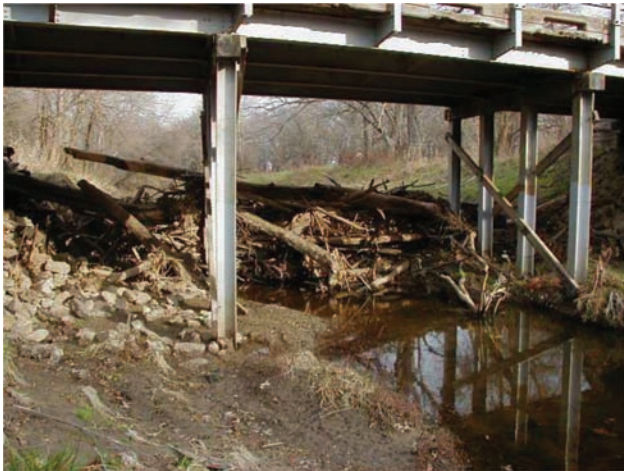
Figure G14.1 Logjam accumulated next to substructure's elements, which is a hazard to the whole structure (MoDOT, n.d.).
