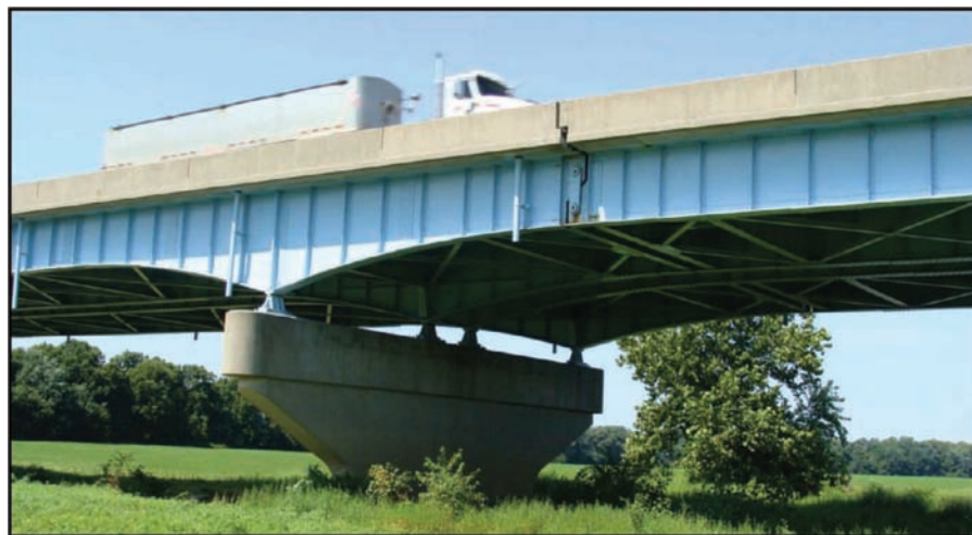
Figure F10.1 Pin and hanger connection at the US-41 White River Bridge, in Hazelton, Indiana (Sherman, Mueller, Connor, & Bowman, 2011).
