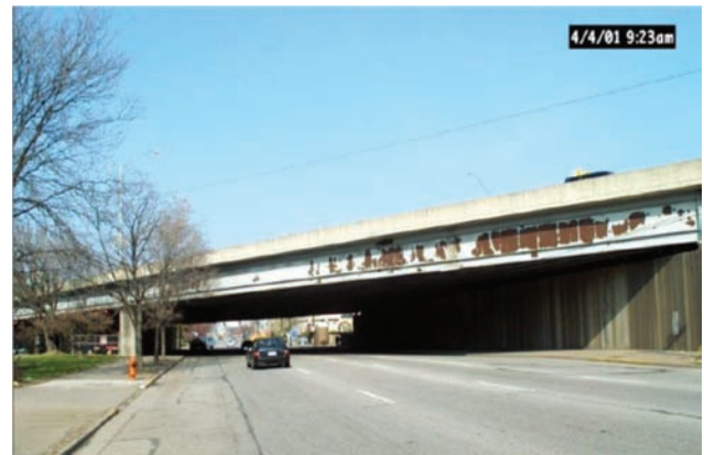
Figure F7.1 Steel girder coating showing damages (Meade, 2013).
