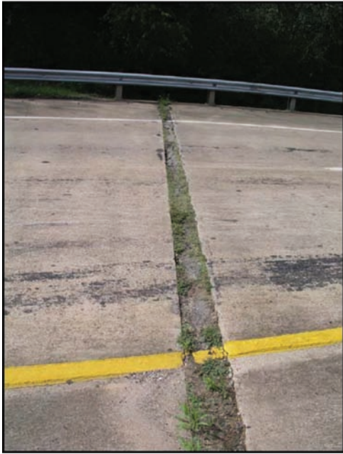
Figure F5.3 Poorly maintained wide joint between bridge deck and approach slab (Jayawickrama et al., 2005).
