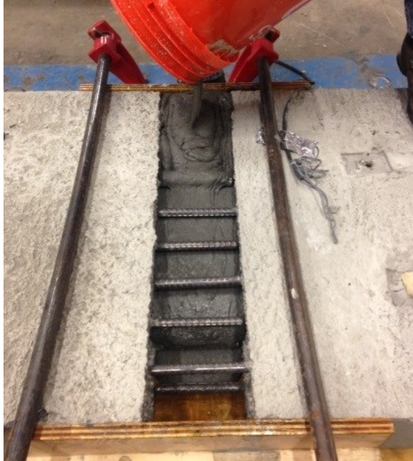
Figure 25. Photo. Placement of UHPC in the connection region of a deck-level connection specimen.
