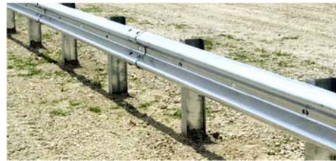
Fig. 1.1: A strong-post W-beam guardrail.
