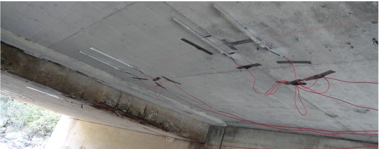
Figure 16: Smyrna No. 2250 underside general condition with joint detail
