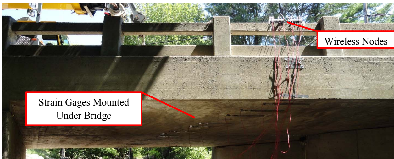
Figure 1: Typical strain sensors mounted under bridge connected to wireless nodes
