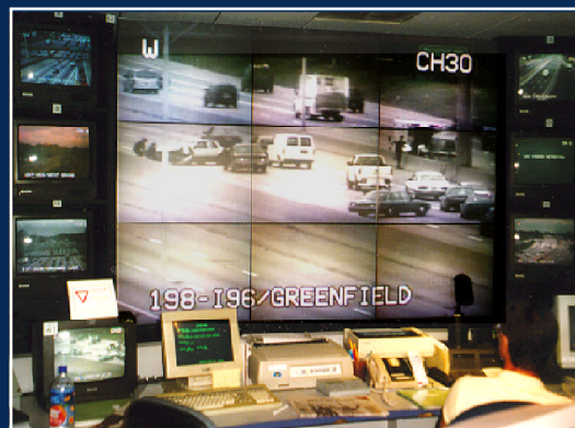
MICHIGAN INTELLIGENT TRANSPORTATION SYSTEMS CONTROL CENTER
