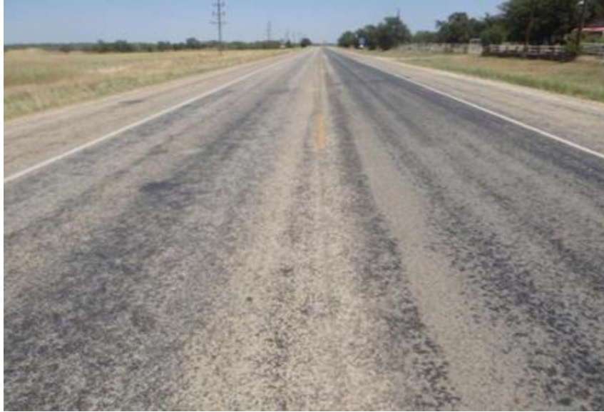
Figure 28. US 183 Bleeding Surface Treatment prior to PFC Surfacing.
