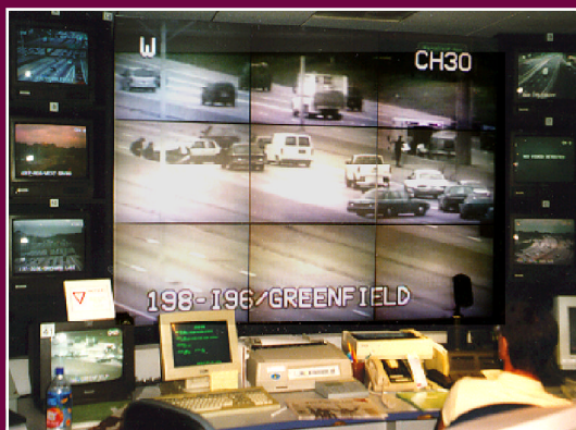
MICHIGAN INTELLIGENT TRANSPORTATION SYSTEMS CONTROL CENTER
