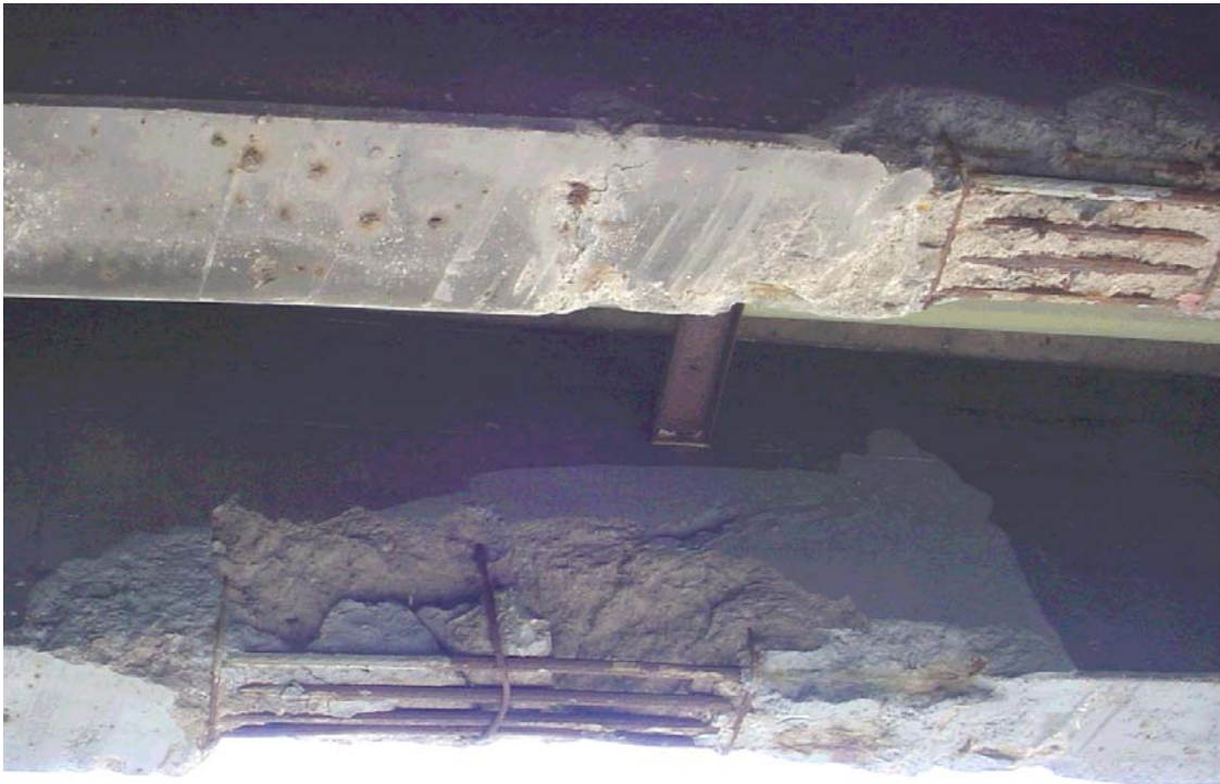
Figure 1 Impact damages in the concrete bridge girders by over-height trucks
