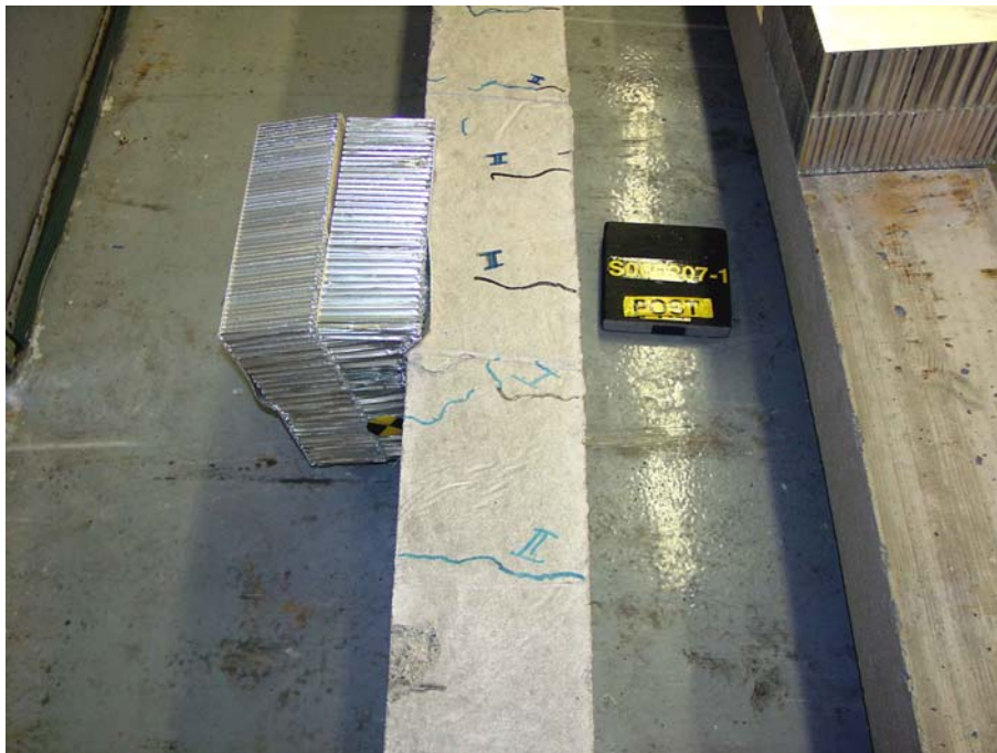
(b) Marked crack and/or damage
