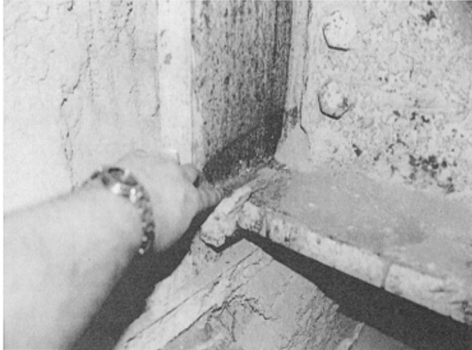
Figure 1. Beam-column connection damage (Kiremedjian, 1999)
