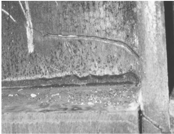
Figure 3. Cracks through column flange and extending into web (Hall, 1995)
