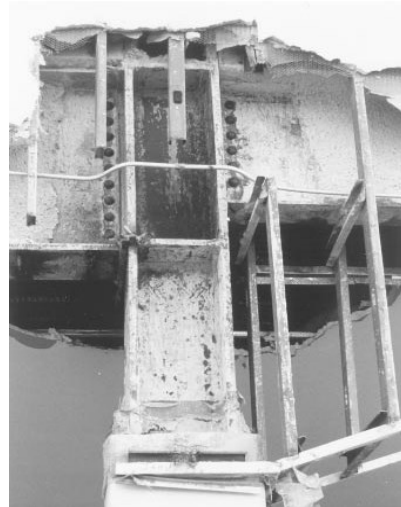
Figure 2. Plastic hinging at top of column (Hall, 1995)
