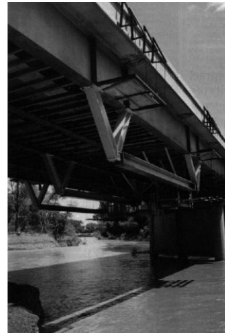
Figure 6. ISB vibration absorber on I-35 bridge (Patten et al. , 1999)
