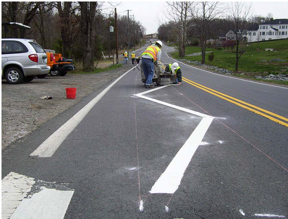
Figure D-2. Marking Painting on Northbound Approach of Belmont Ridge Road
