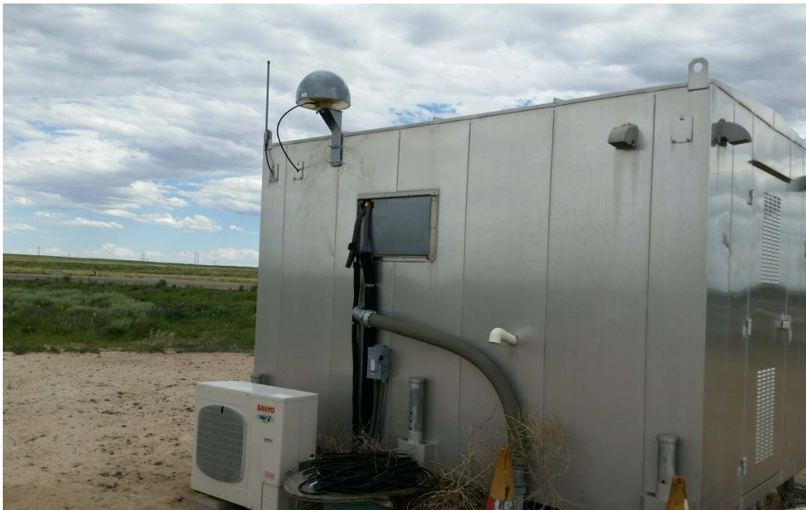
Figure 3. Integrity Monitoring GPS Station (Post 85 Bungalow)
