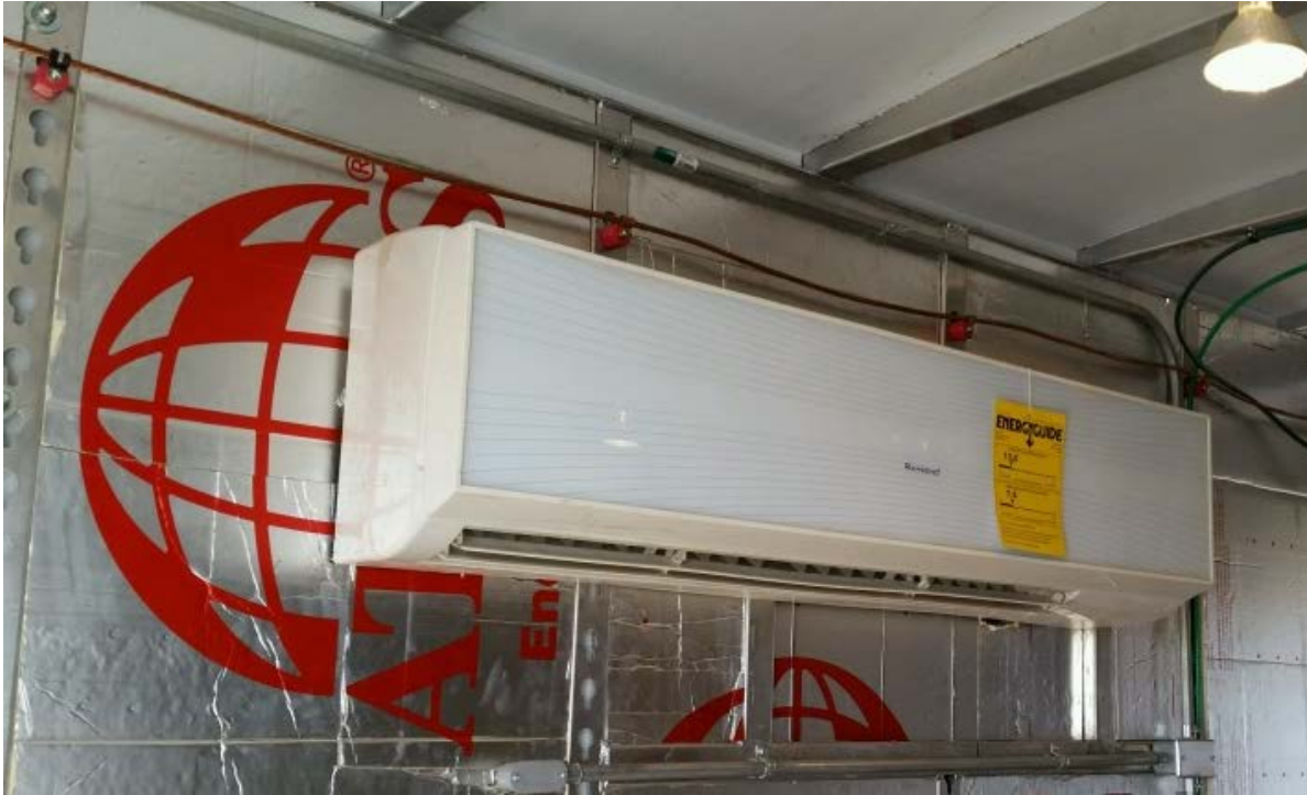
Figure 8. HVAC Unit and Insulation installed in the Equipment House
