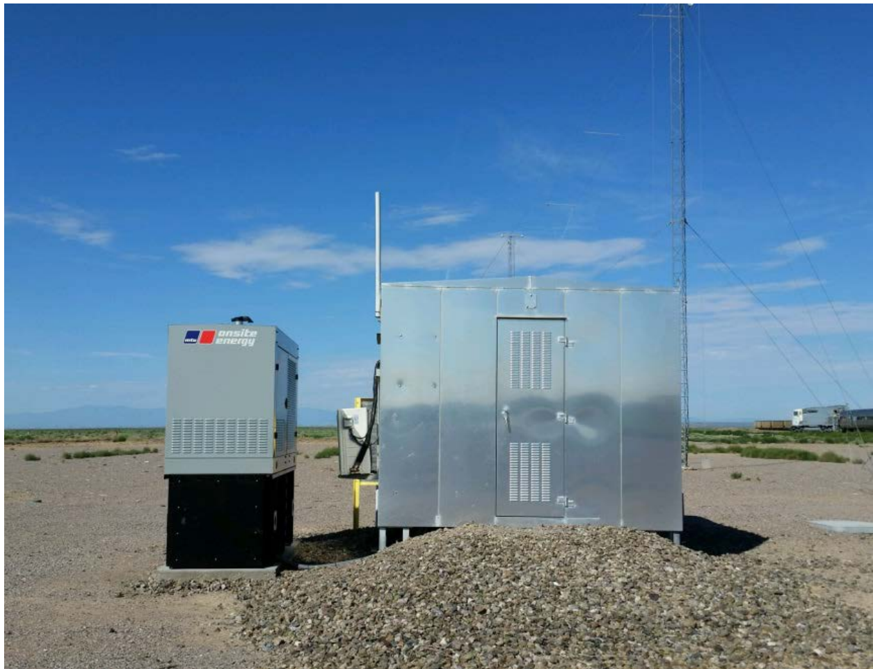
Figure 9. Site Backup Power Generator
