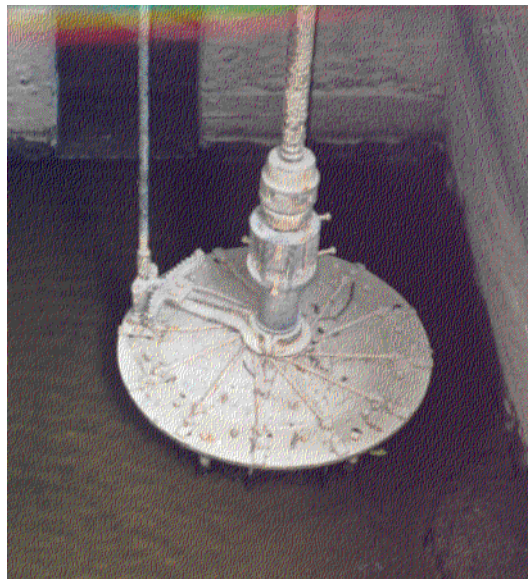
Figure 83. A pre-1913 Leffel turbine with wicket gate design, showing link rods to gates and gate control rod going upward into mill, also drive shaft and upper bearing case.
