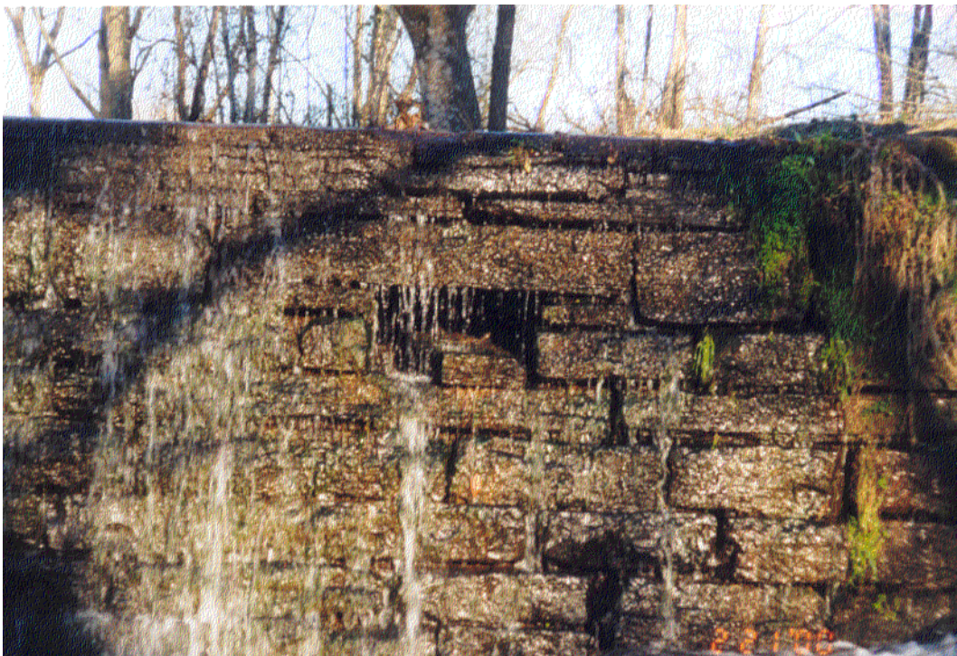
Figure 26. Masonry dam showing high drain hole in the center of the photograph.
