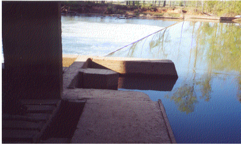
Figure 27. Flood gates (closed) at Ketner's Mill dam in Marion County, Tennessee.
