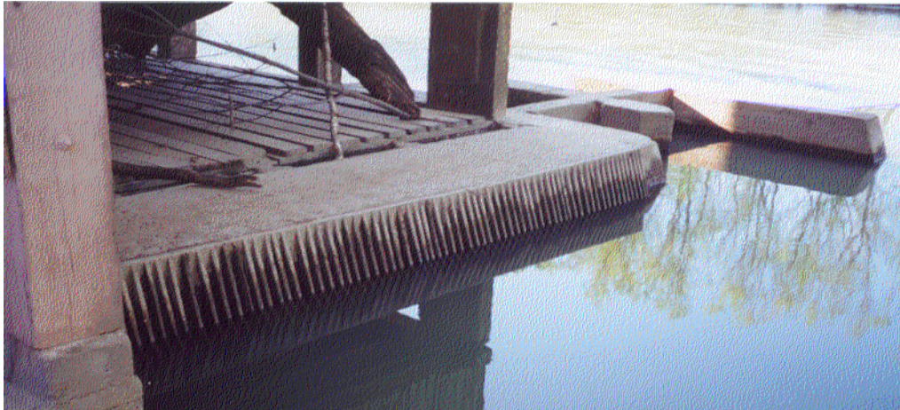
Figure 85. The turbine trash rack at Ketner's Mill in Marion County, Tennessee.
