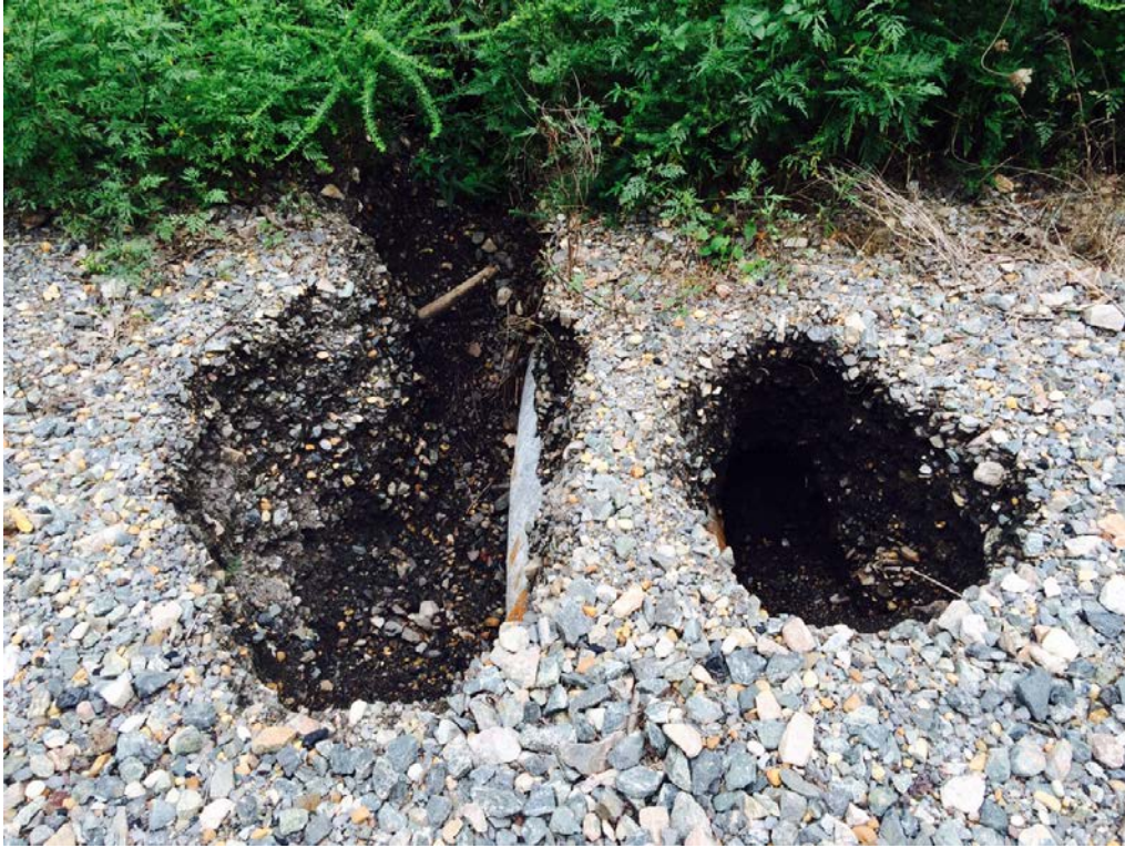
Figure 20. Example of poor drainage condition leading to ballast washout
