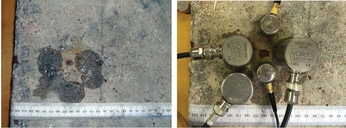
Figure 4: Photographs of a concrete block tested in the laboratory. Fine cracks originate from the reinforcing steel bar, owing to the development of corrosive layers around the steel bar. Also, the infusion of iron oxide around the porous structure of the concrete is seen in the photograph, which influences the resistivity of the concrete. Traces of silicone grease used in coupling AE probes are seen around the steel bar.
