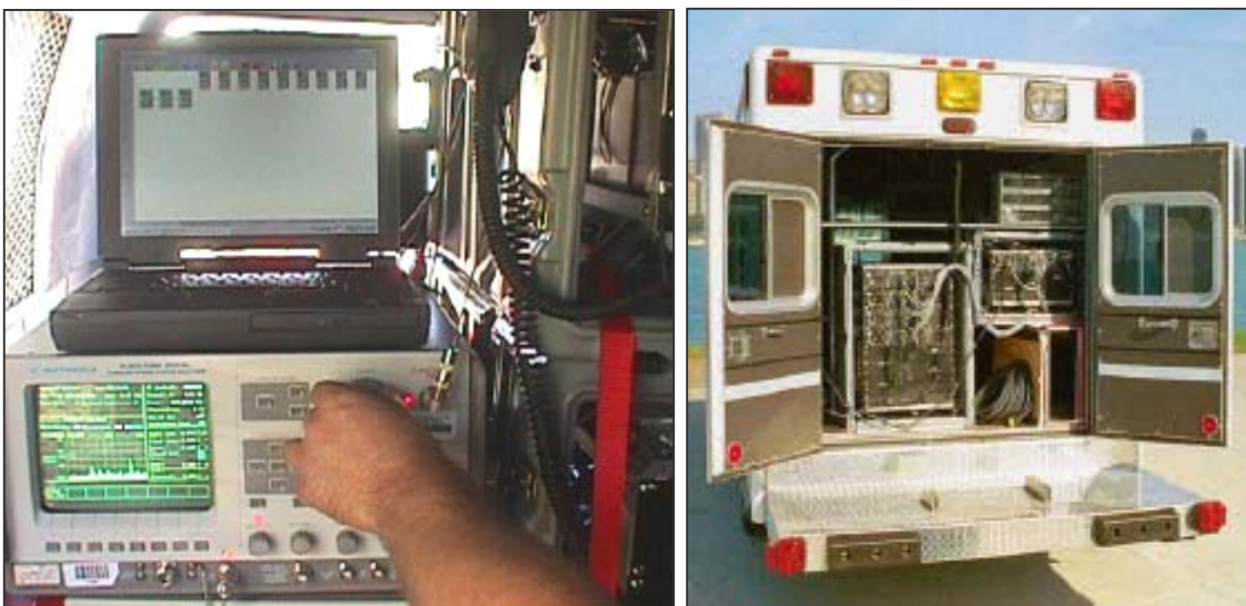
Figure 12 – Typical ACU-1000 System Configuration for Mobile Operations
