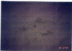
Photo #5 Very light block cracking in the westbound tined sections
