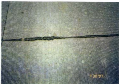
Photo #4 Overfilled joints in the eastbound lanes of the diamond ground sections
