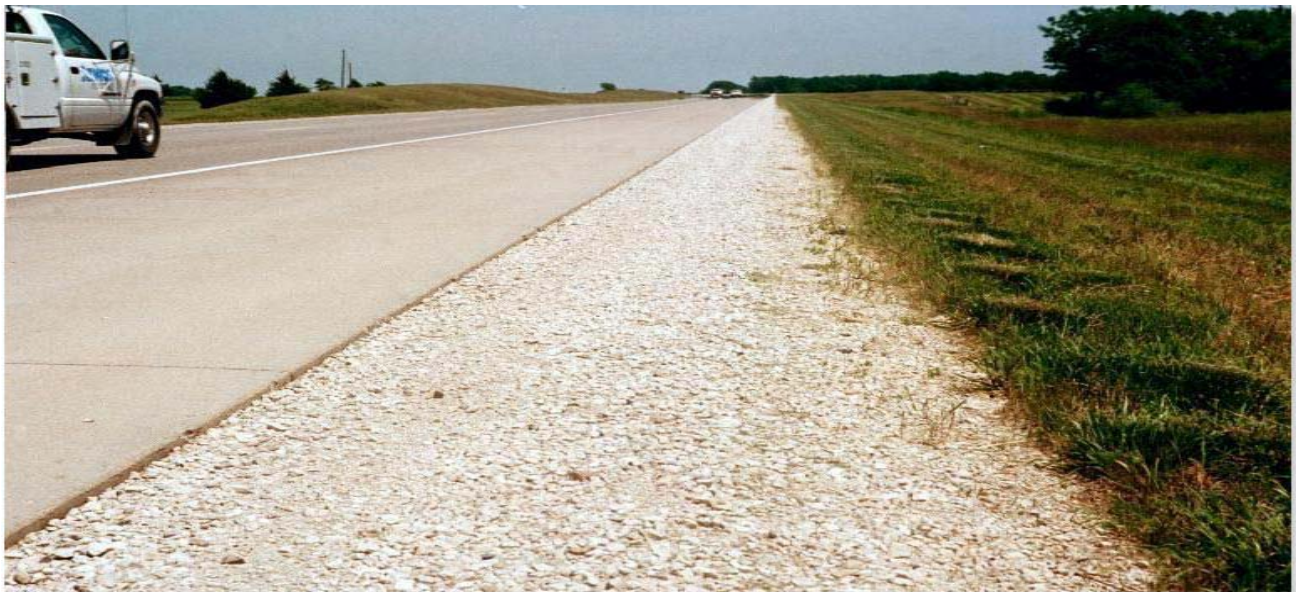
FIGURE 3: Expected aggregate appearance of a daylighted drainable base. This is the right shoulder on US-50 at Station 242+00
