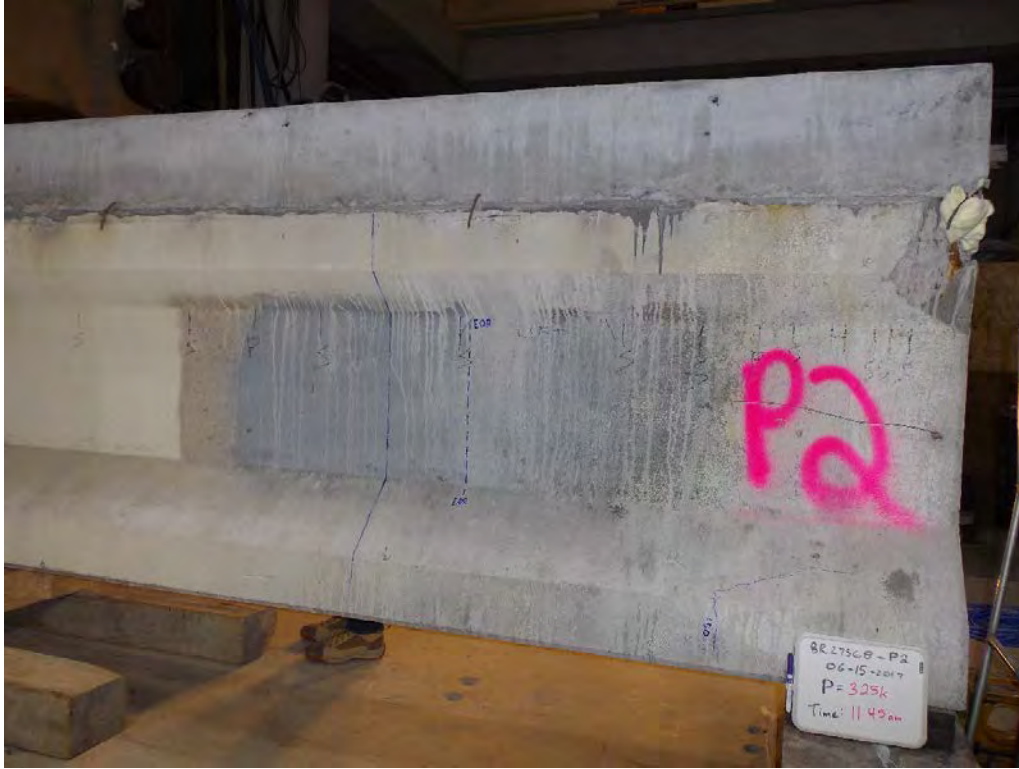
Figure B.20 Girder P2 Northside Section 1-Section 2 P=325 kips
