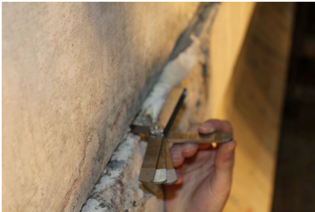
Figure 4.49 Separation between the deck and top flange of Girder P26.
