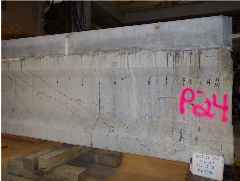
Figure B.79 Girder P24 Northside Section 1-Section 2 P=375 kips
