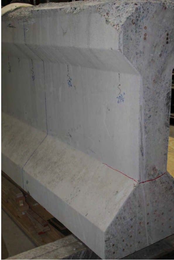
Figure 2.3 Typical cut-end horizontal crack in Girders P2, P4, and P26 (marked in red)
