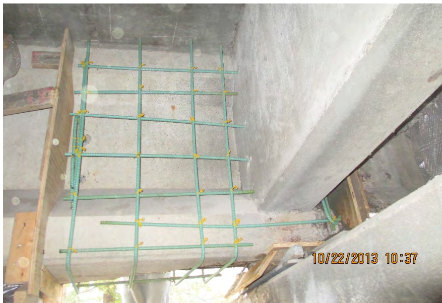
Figure A.20: Inside face view of P26 beam end just prior to shotcreting.
