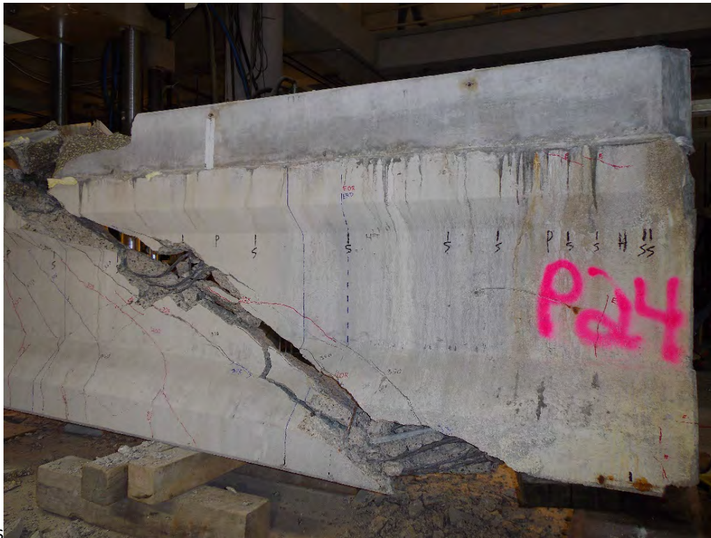
Figure B.82 Girder P24 Northside Section 1-Section 2 Failure
