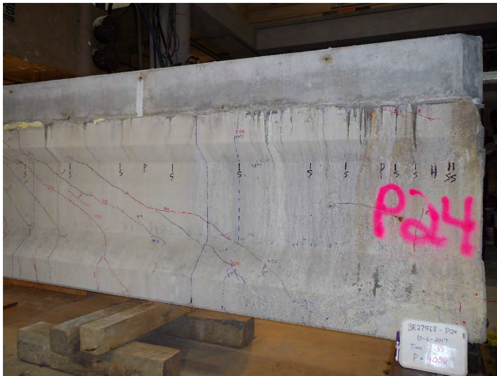
Figure B.80 Girder P24 Northside Section 1-Section 2 P=400 kips
