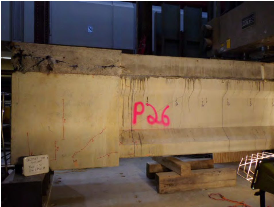
Figure 4.5 Girder P26 web shear cracking P=325k
