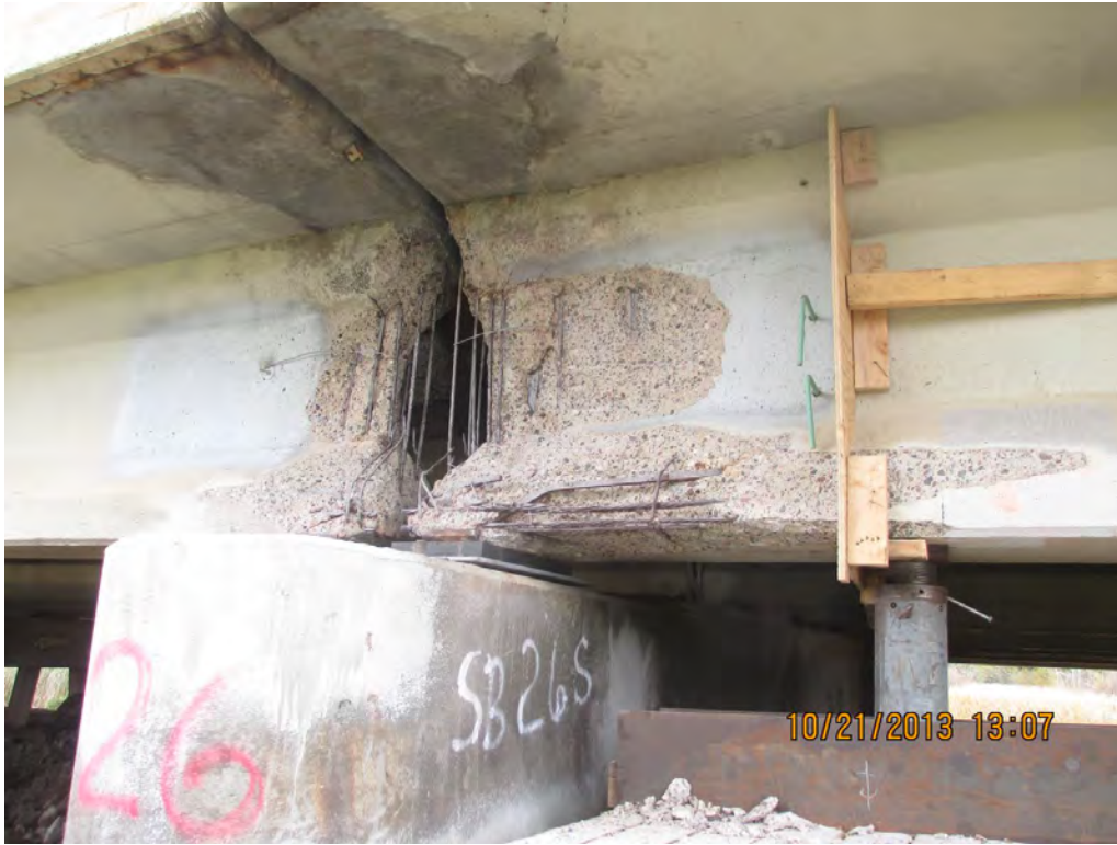
Figure 1.3 Severely corroded girder at Pier 26
