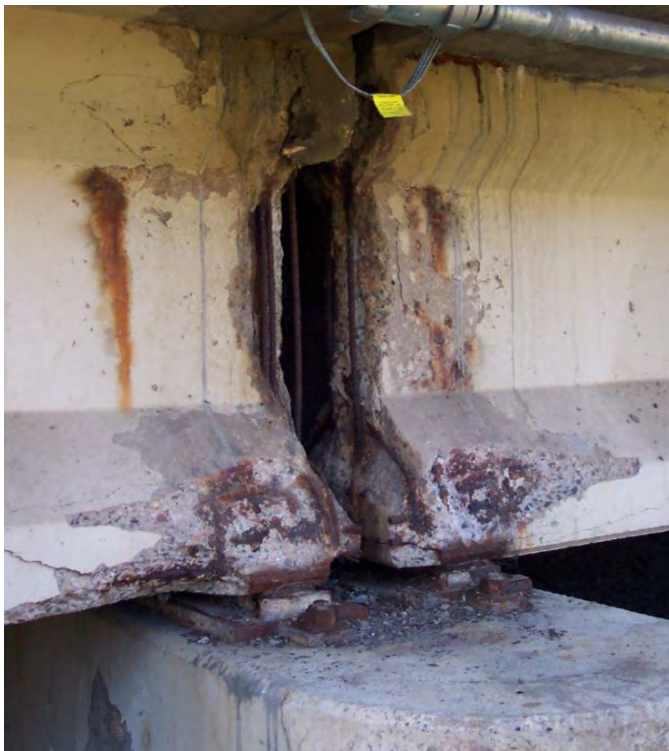
Figure A.7: Photo from October 2010 of Pier 4 beam end prior to final scoping
