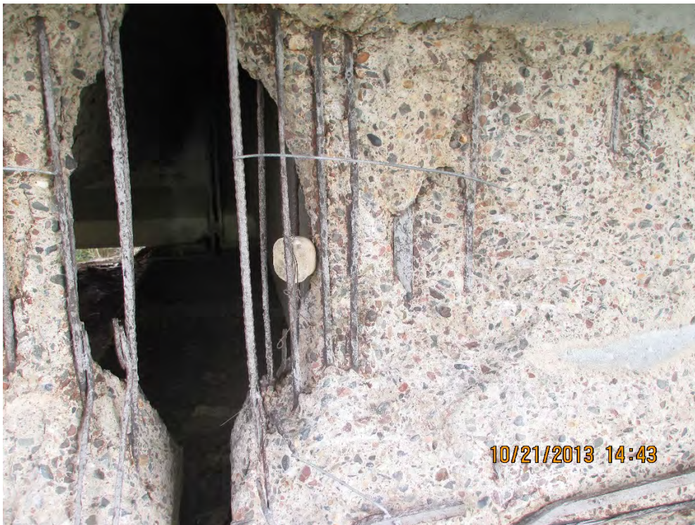
Figure A.18: Prepared beam end at Pie 26 prior to installation of mild rebar.
