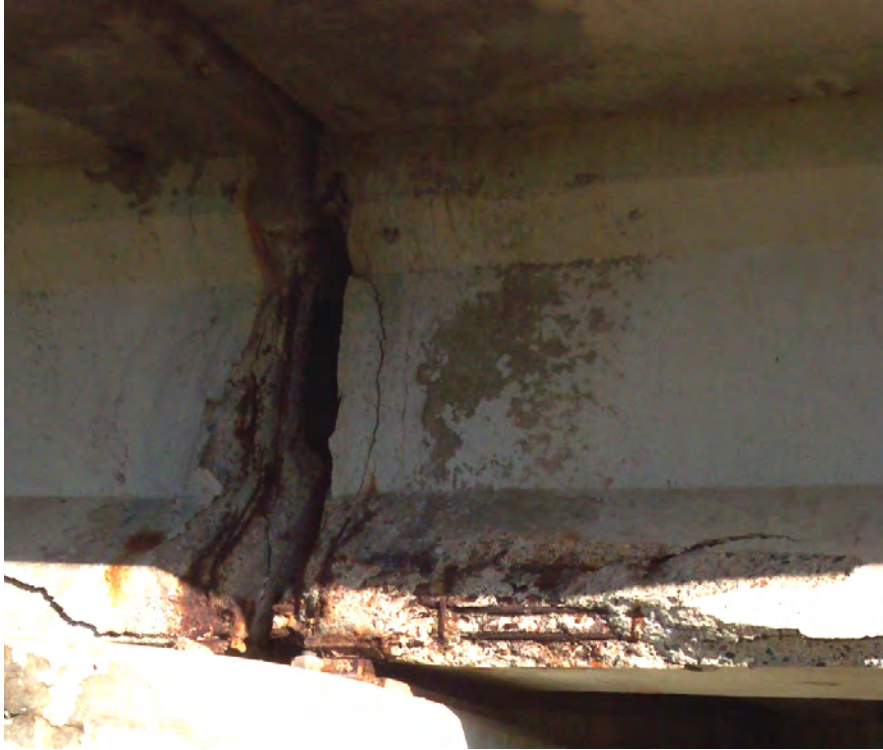
Figure A.8: Photo from October 2010 of Pier 26 beam end prior to final scoping
