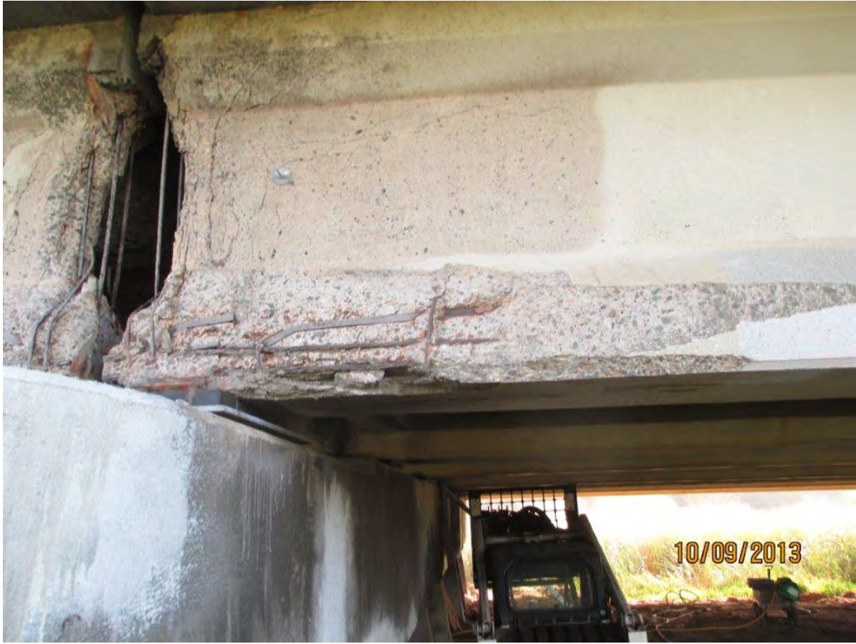
Figure A.12: Sandblasted beam end at Pier 26 prior to issuing box-style repair design details.
