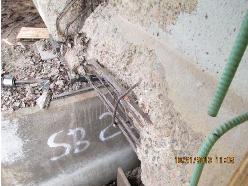
Figure 1.5 Exposed strand in girder at Pier 26
