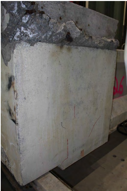
Figure 2.10 As-received cracking on Girder P26 on exterior side
