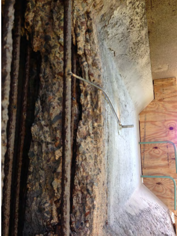
Figure A.17: Separation of concrete web concrete upon slow jacking from temporary support location. Separation was likely due to rebalancing of internal prestress forces. After the separation was reported the jacking pressure was immediately reduced to 50% dead load take-up from 100% dead load. The repair proceeded under 50% dead load take-up.
