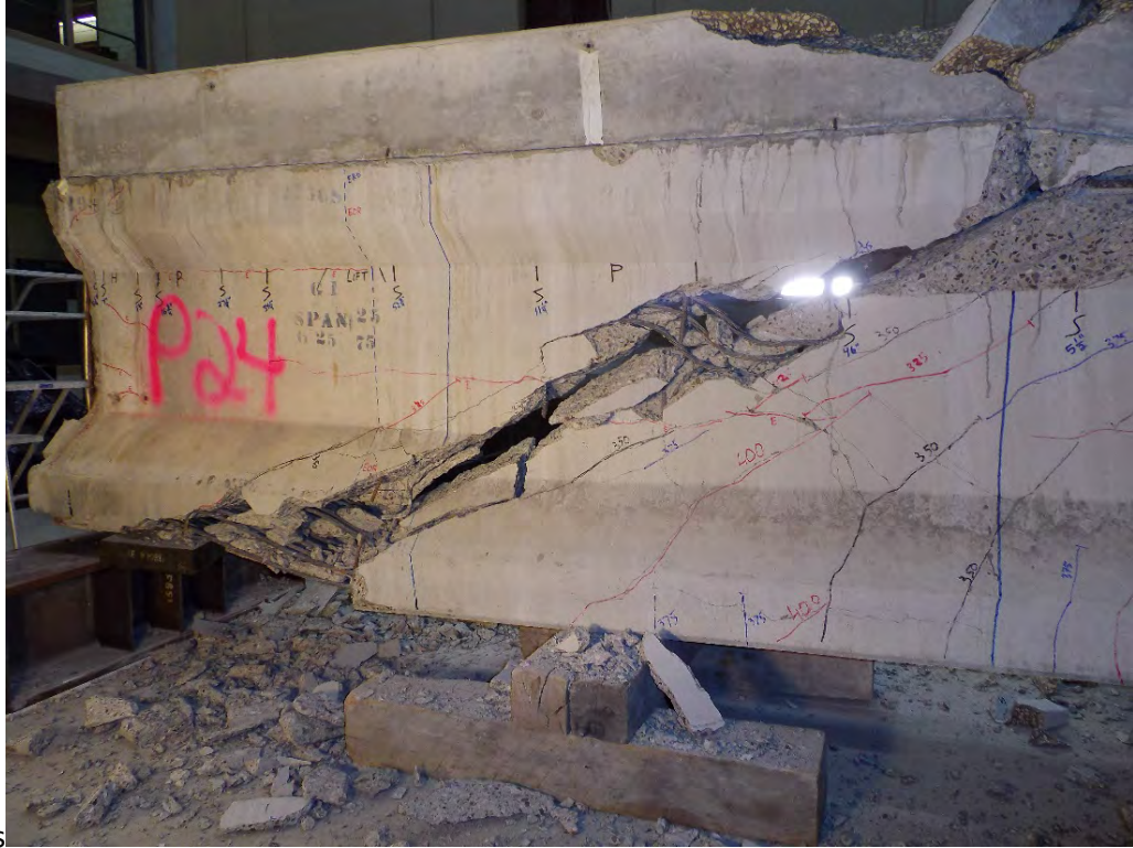
Figure B.73 Girder P24 Southside Section 1-Section 2 Failure
