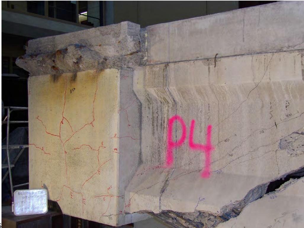
Figure B.56 Girder P4 Repair Section 1 Failure
