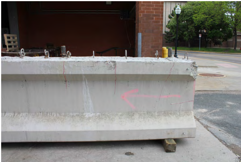
Figure 2.4 Girder P24 cut-end cracking
