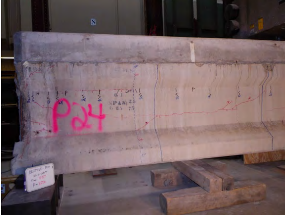
Figure 4.4 Girder P24 web shear cracking P=325k
