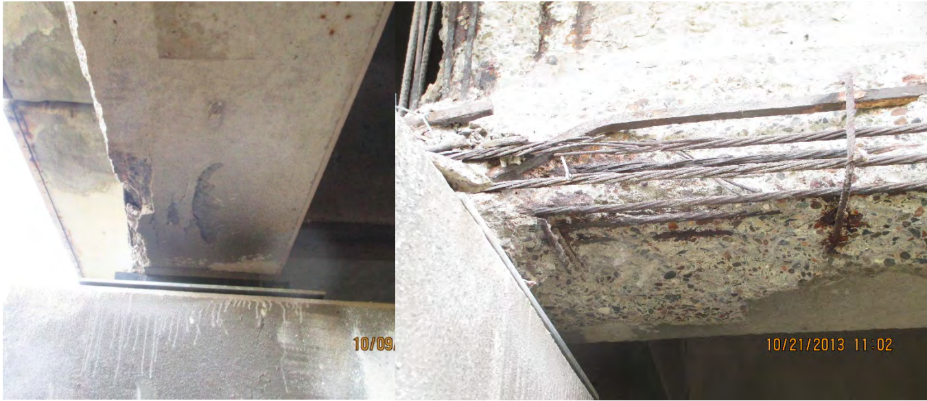
Figure A.13: Underside of Pier 26 beam prior to preparation.
