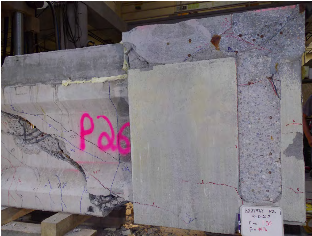
Figure B.107 Girder P26 Northside Section 1-Section 2 Failure
