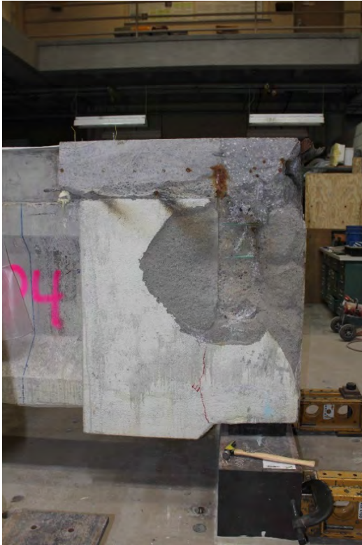
Figure 2.6 Damage to the repair on the diaphragm side of Girder P4
