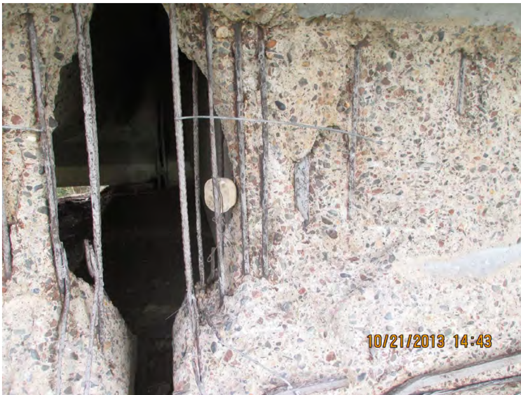
Figure 1.4 Damaged concrete and transverse reinforcement in girder at Pier 26
