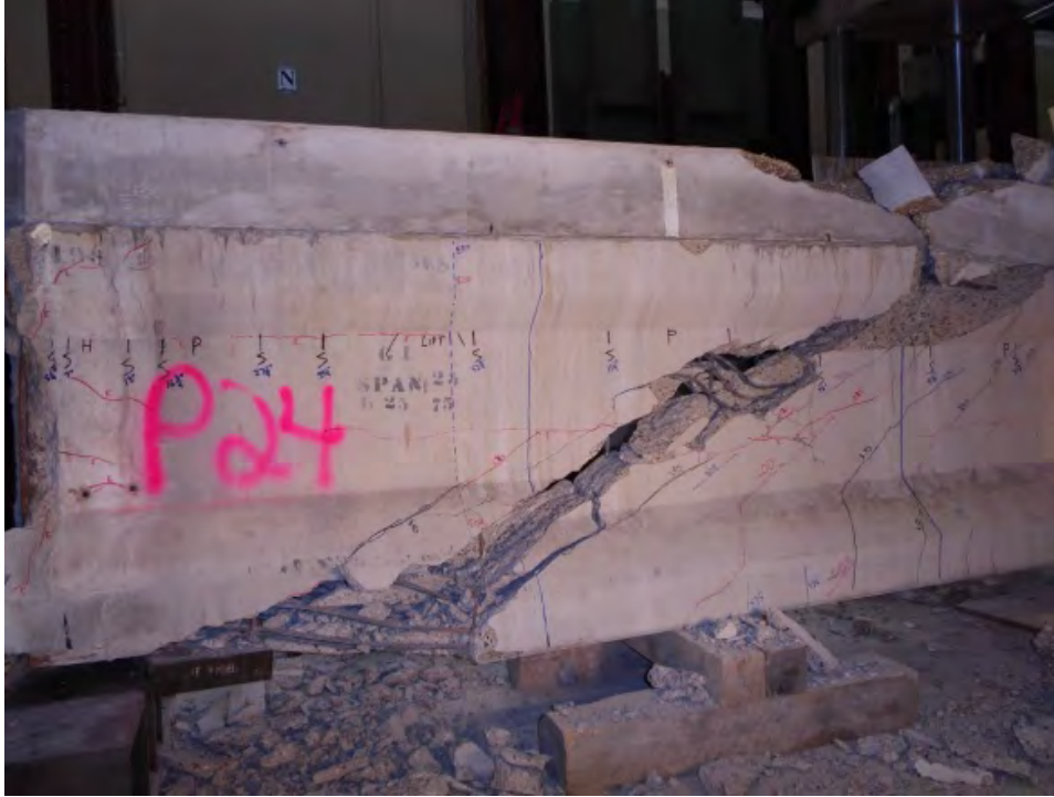
Figure 4.12 Girder P24 after failure
