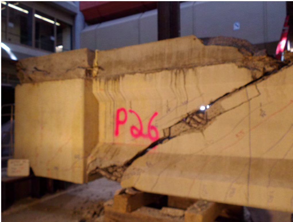
Figure B.115 Girder P26 Repair Section 1 – Section 2 Failure
