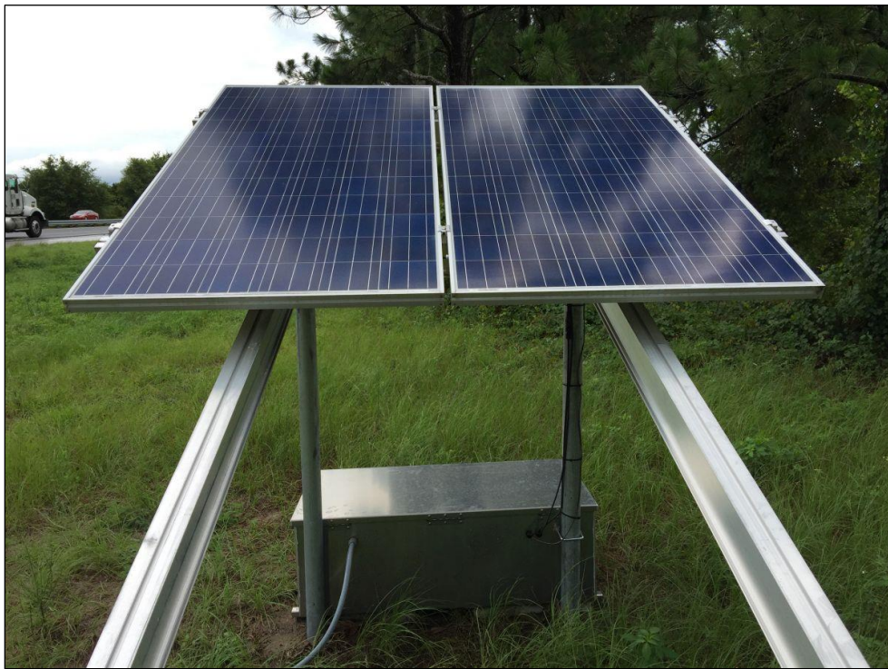
Figure B-0-12: Solar Power Unit – Location 3
