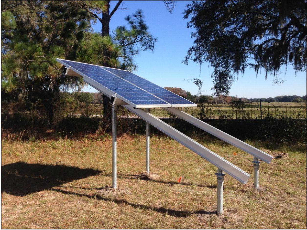
Figure 3-9: Solar Power System – Location 3
