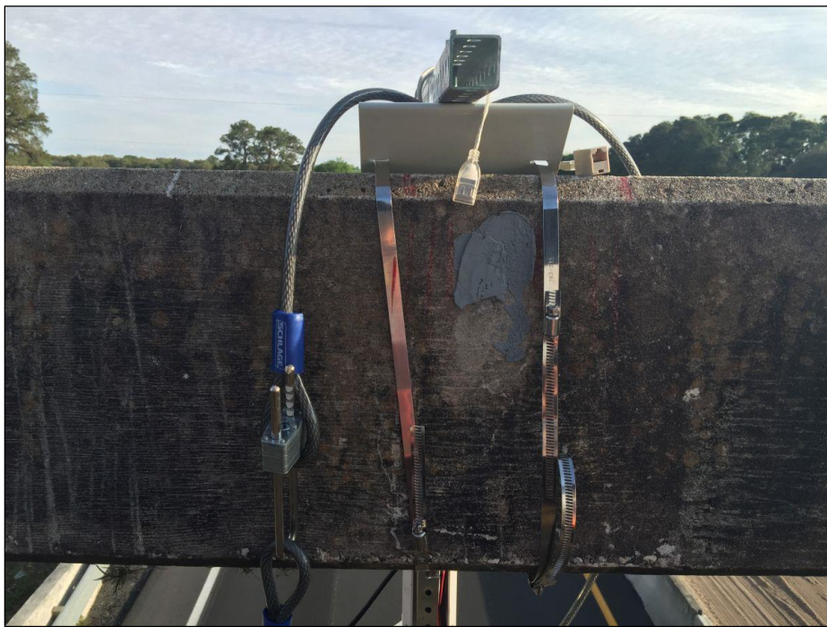
Figure B-0-8: Bracket Strapped to Overpass
