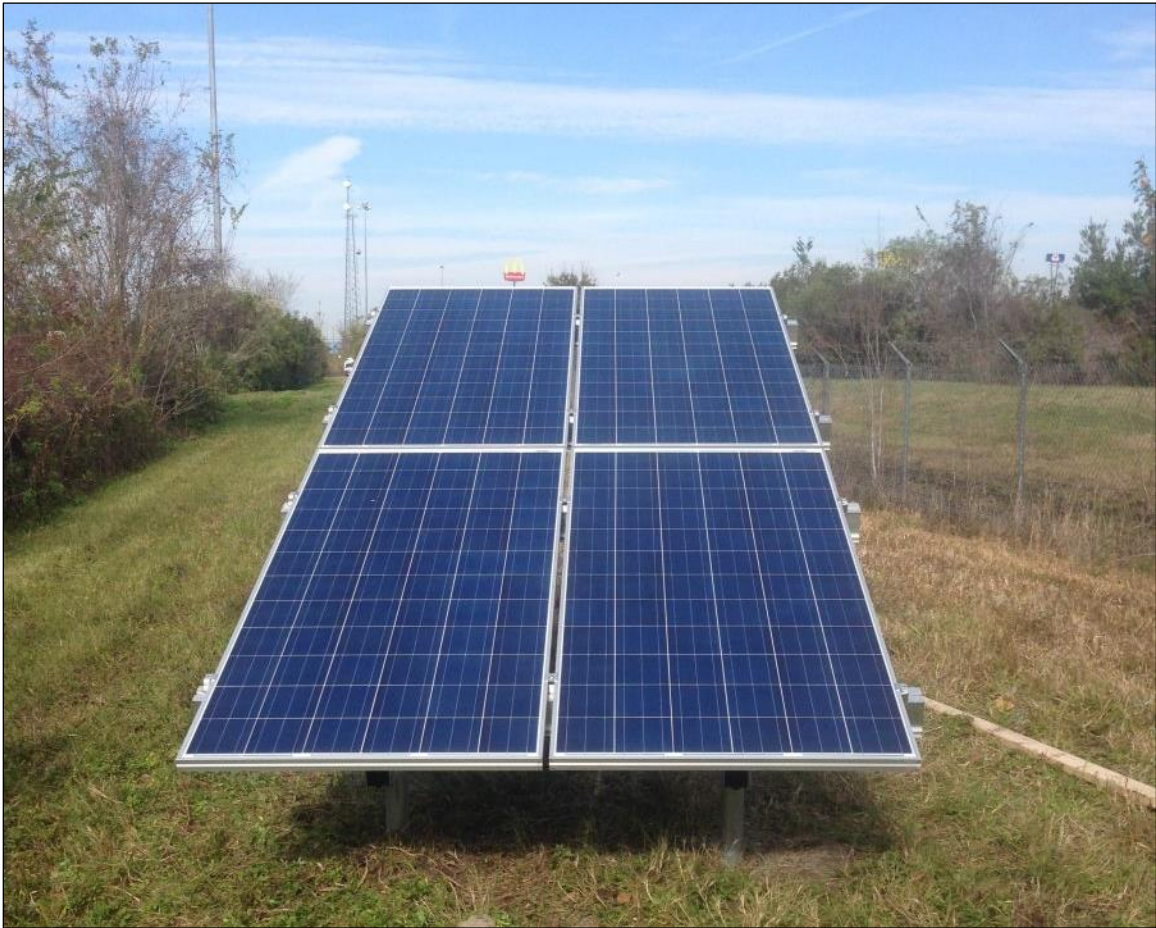
Figure 3-8: Solar Power System – Location 2
