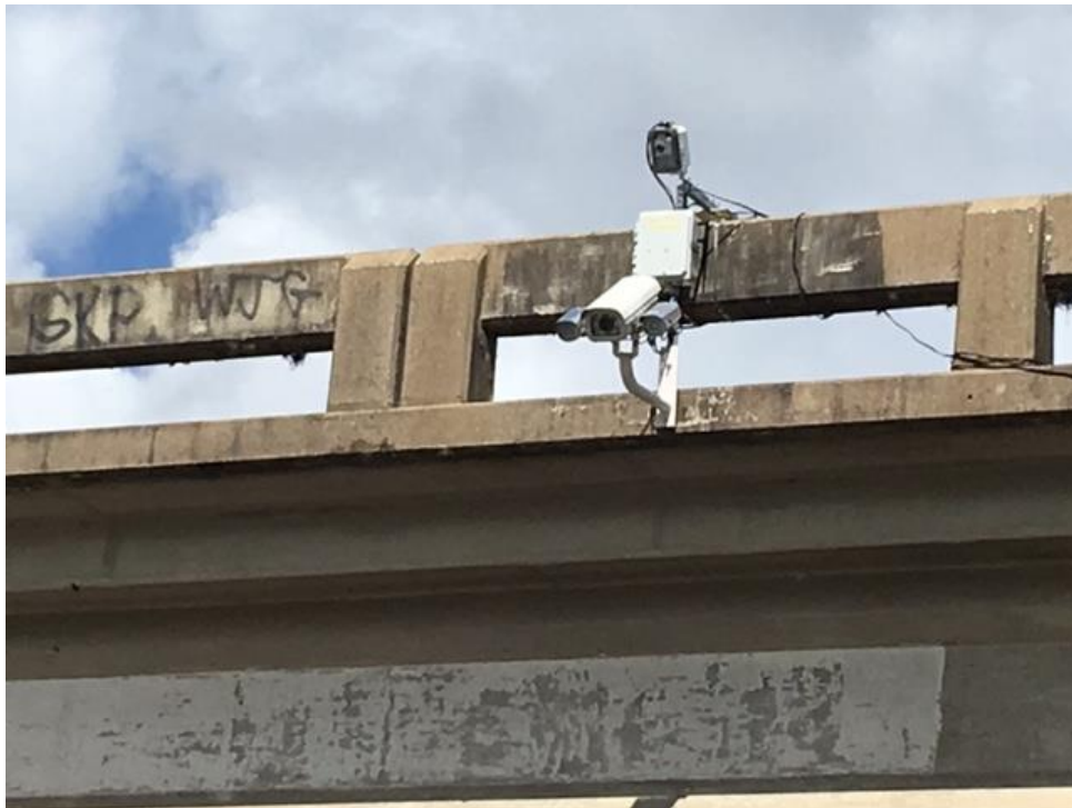
Figure 4-8: Bracket Close-up Showing Sensor, Camera, and Processor
