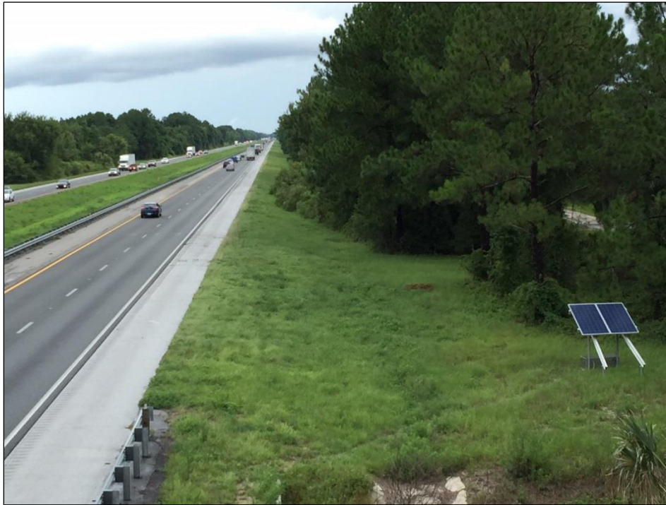
Figure B-0-11: Solar Power Unit – Location 3
