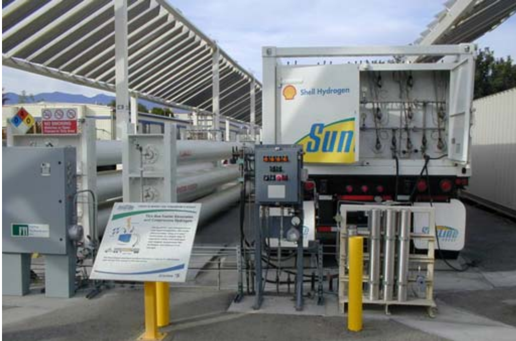
Figure 13. Hydrogen storage at SunLine
