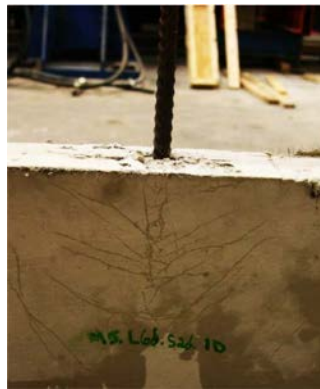
Figure 7.5. Diagonal crack pattern observed by Graybeal.
