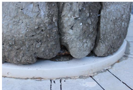
Figure 3.4 – Bottom of Pile Specimen #1 showing exposed reinforcement
