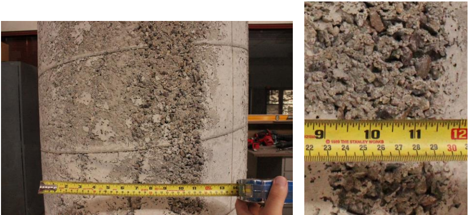
Figure 3.15 – Exposed aggregate in Pile Specimen #8
