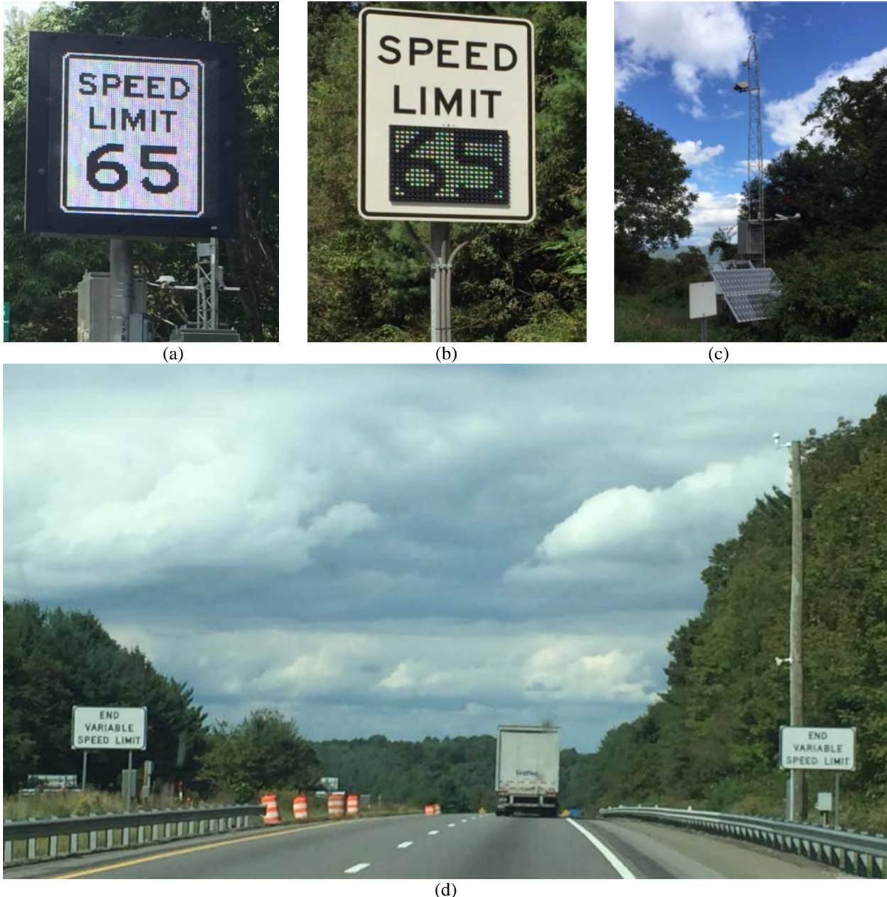
Figure 3. VSL System Devices: (a) full matrix DMS VSL display; (b) speed limit signs with dynamic VSL cutout; (c) RWIS station; and (d) traffic sensor, CCTV, and signing at the northern end of the corridor. VSL = variable speed limit; DMS = dynamic message sign; RWIS = road weather information system; CCTV = closed circuit television.
