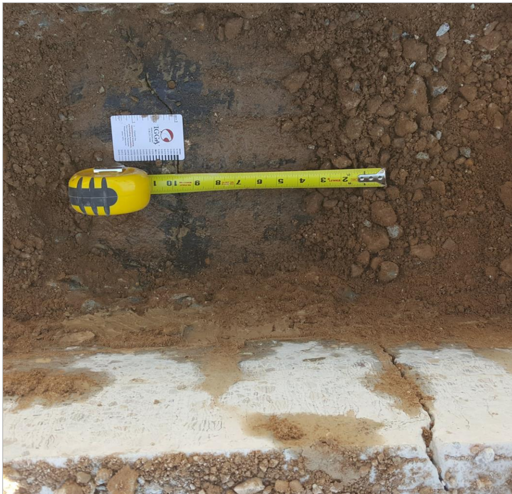
Figure 16: Soil cement base crack
