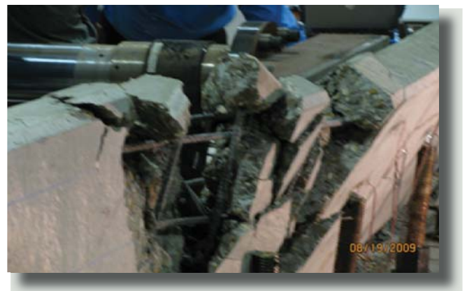
Figure 2 Barrier after failure
