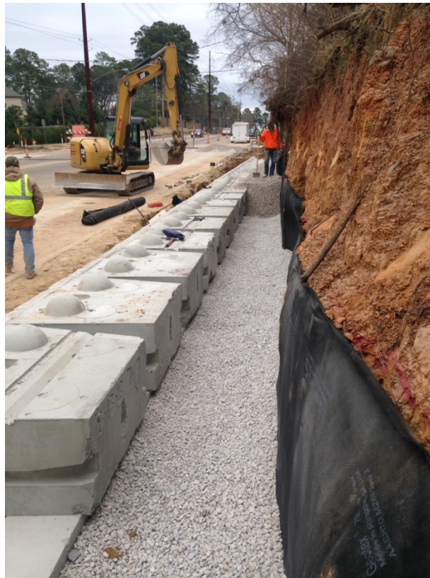
Figure 6. Photo. Unreinforced concrete leveling pad (not shown) with first course of block installed with the stone backfill material shown.
