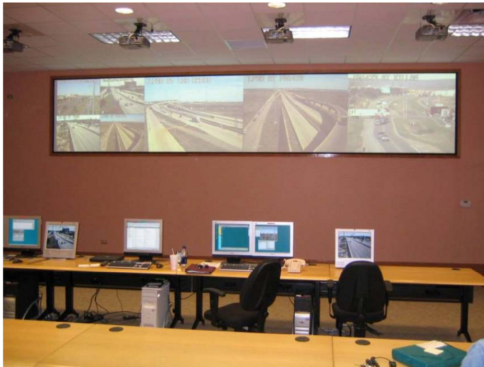
Figure 2-21: Laredo's TMC – STRATIS.
