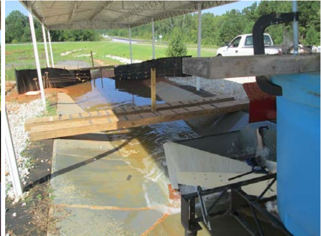
(b) silt fence ditch check w/ weir impoundment
