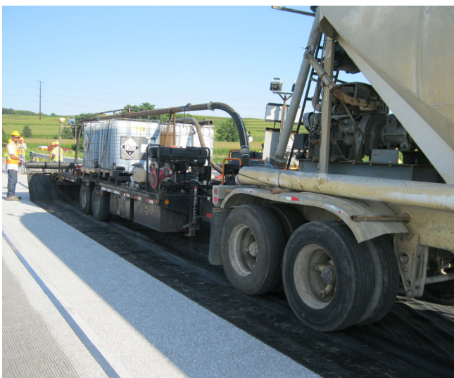
Semi-truck and trailer carrying hopper of flint chips, vats of epoxy polymer, and a blower on the Keg Creek Bridge
