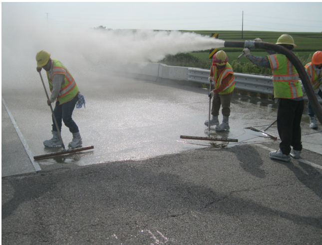
Spreading polymer and blowing flint chips on the Keg Creek Bridge deck
