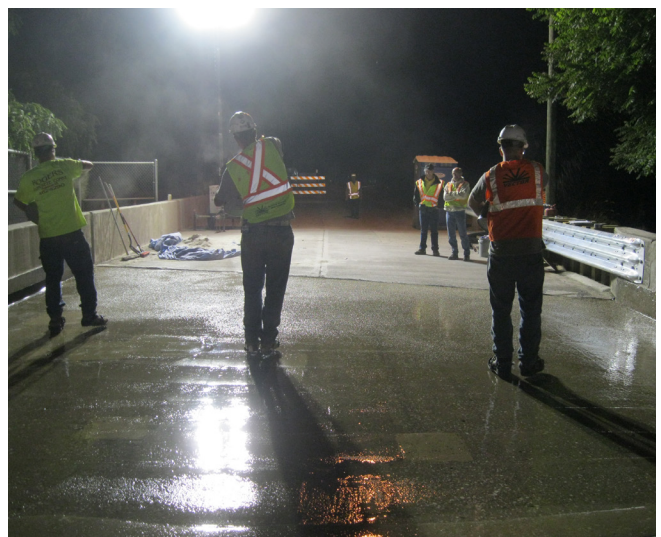
Hand-broadcasting flint chips on the first polymer layer of the Johnson County bridge deck
