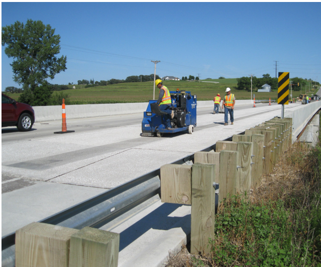
Shot blasting (and vacuuming) the Keg Creek Bridge deck to achieve deck surface relief as part of initial preparation
