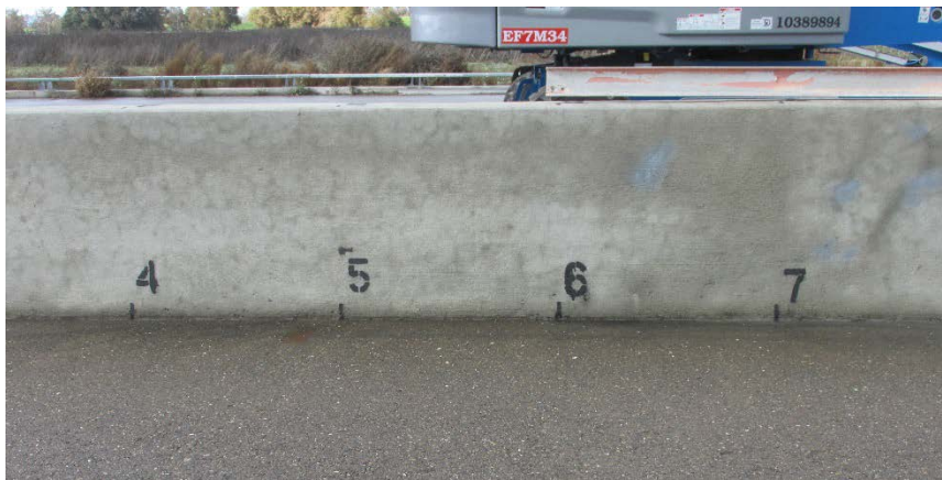
Figure 5-2 Type 60 Barrier Point of Impact (I-beam on barrier was removed prior to test)
