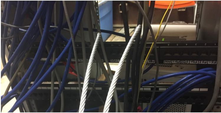
Figure K5. Patch Panels for Ethernet Connection.
