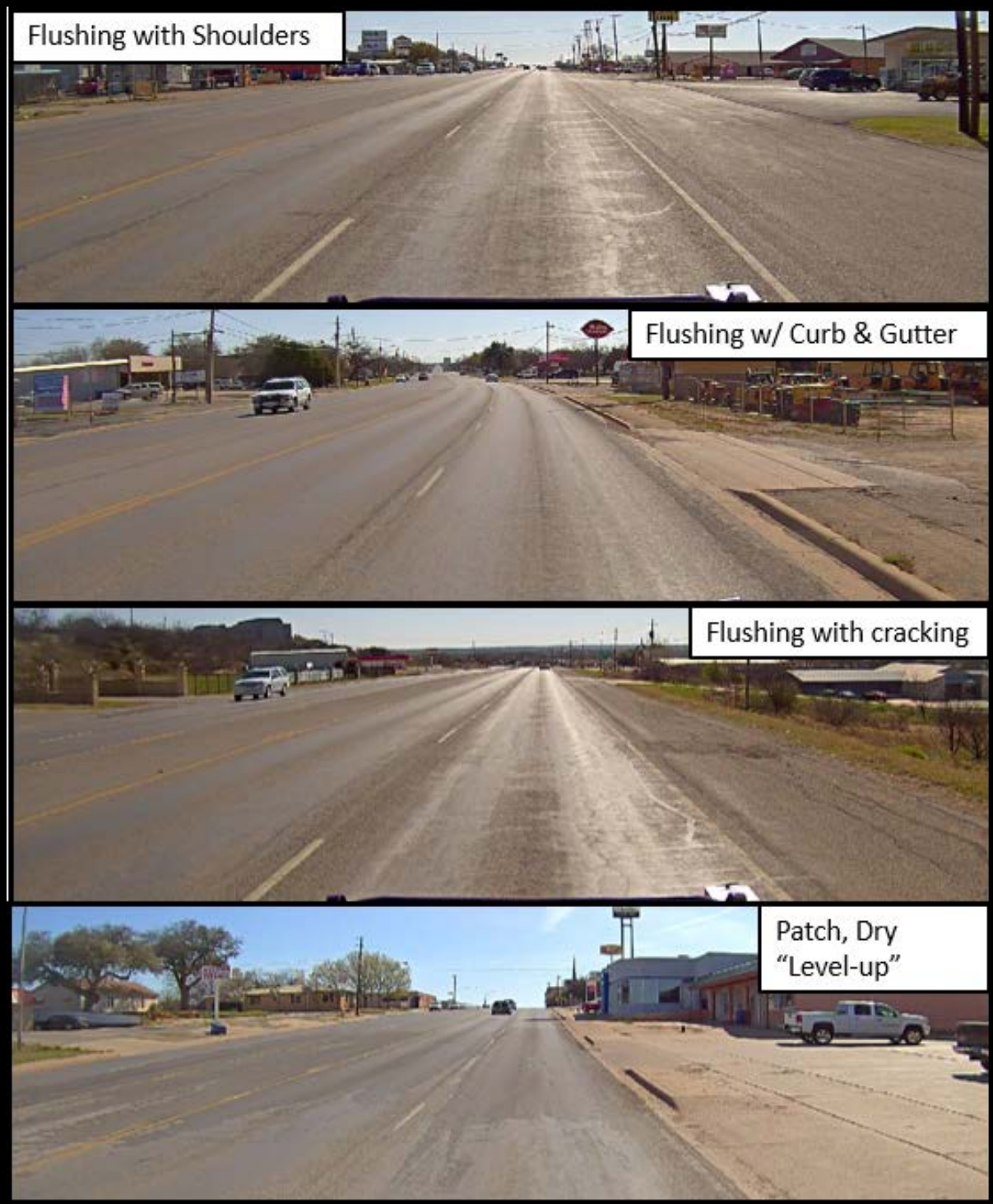
Figure 27. US 180 Surface Conditions.
