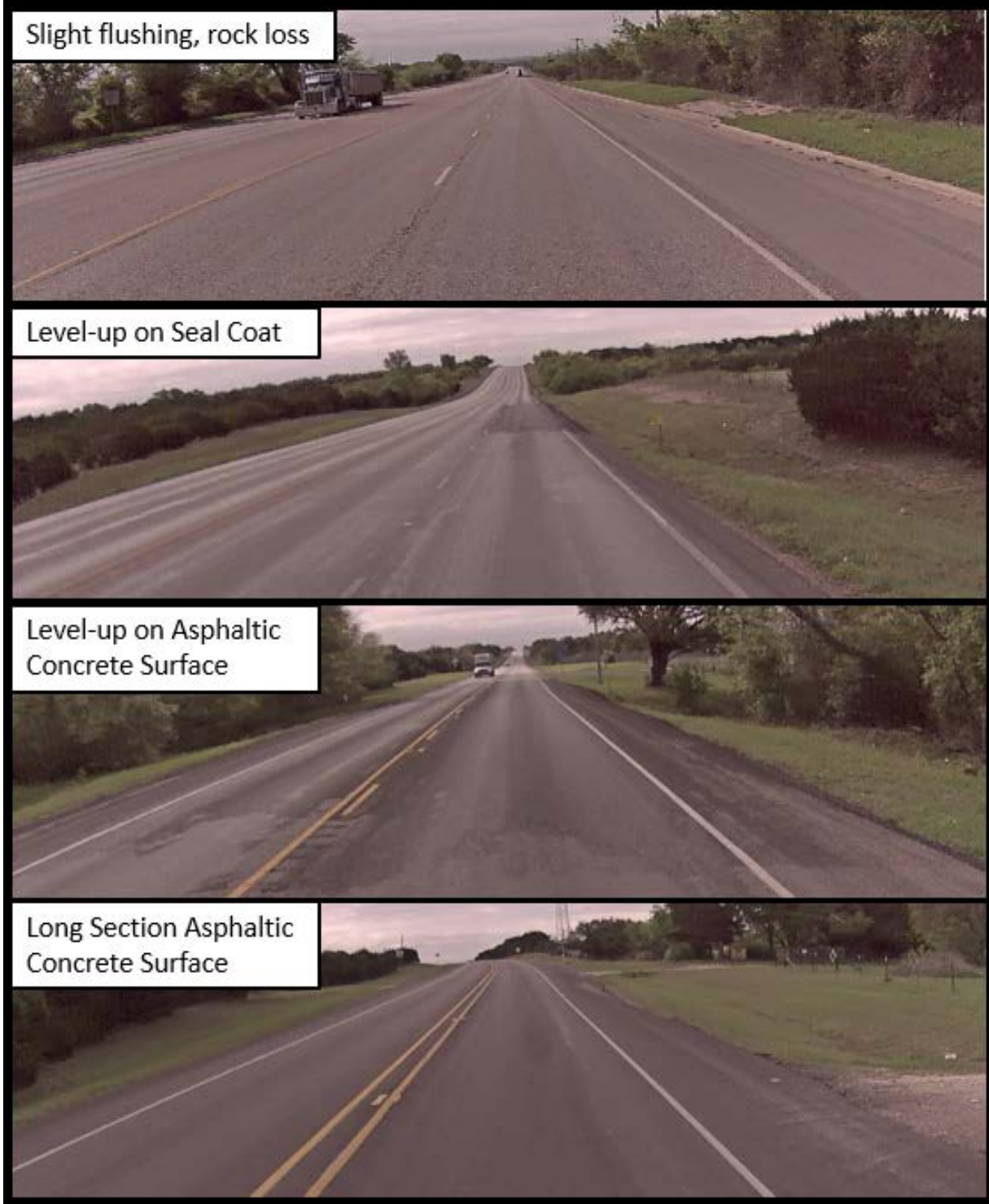
Figure 35. SH 36, Waco District, Surface Conditions.
