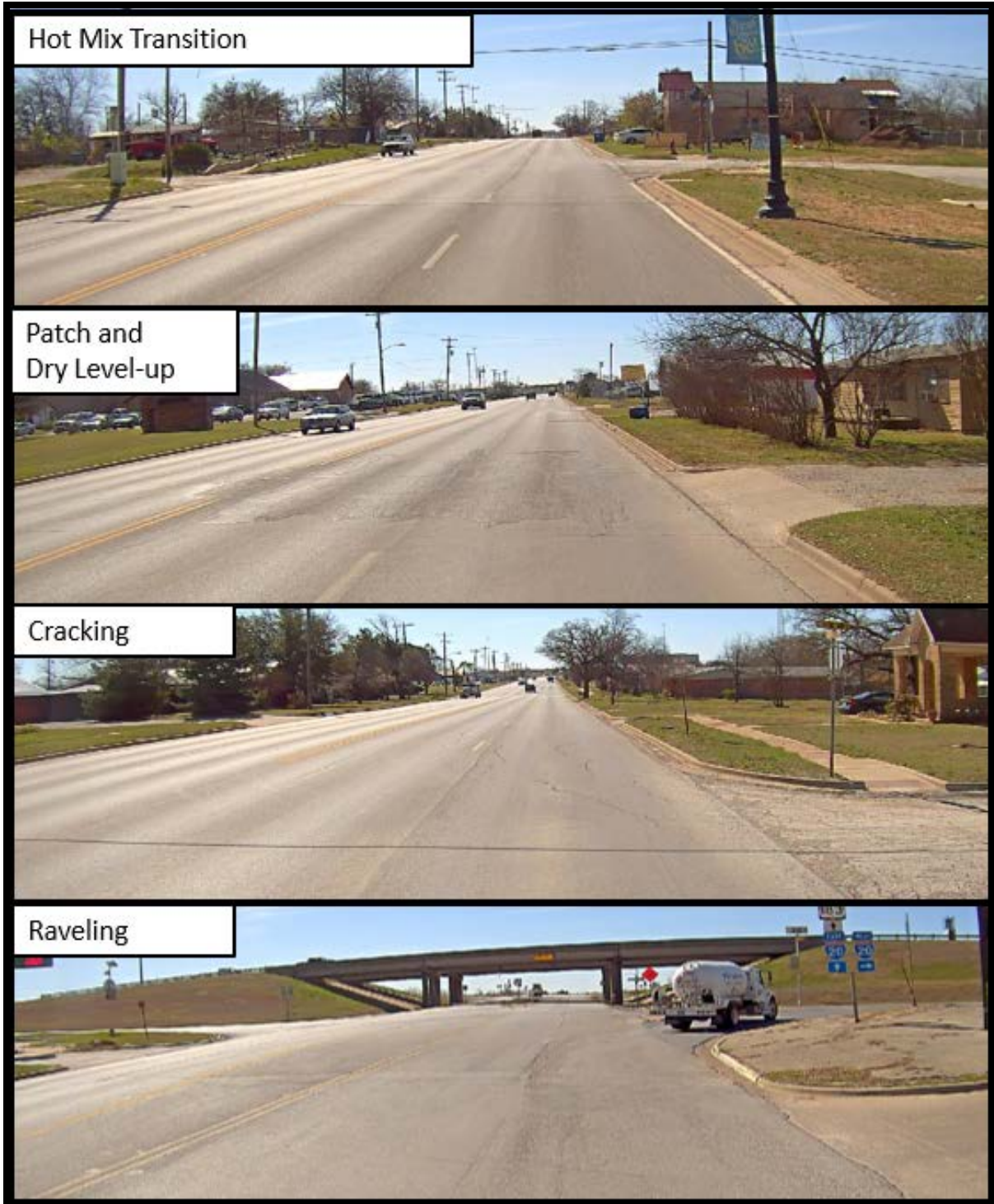
Figure 28. US 183 Surface Conditions.
