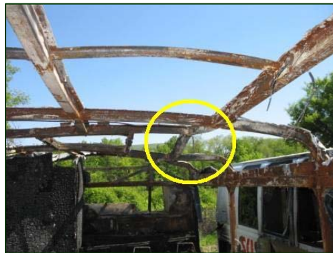
Figure 13. Fire related deformation of the left side roof structure.
