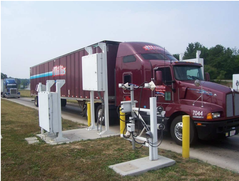
Figure 1-2. London, Kentucky, ISSES deployment. System control cabinet at left; elevated radiation detection panels close to truck lane on either side; visible lighting and identification camera apparatus in foreground.
