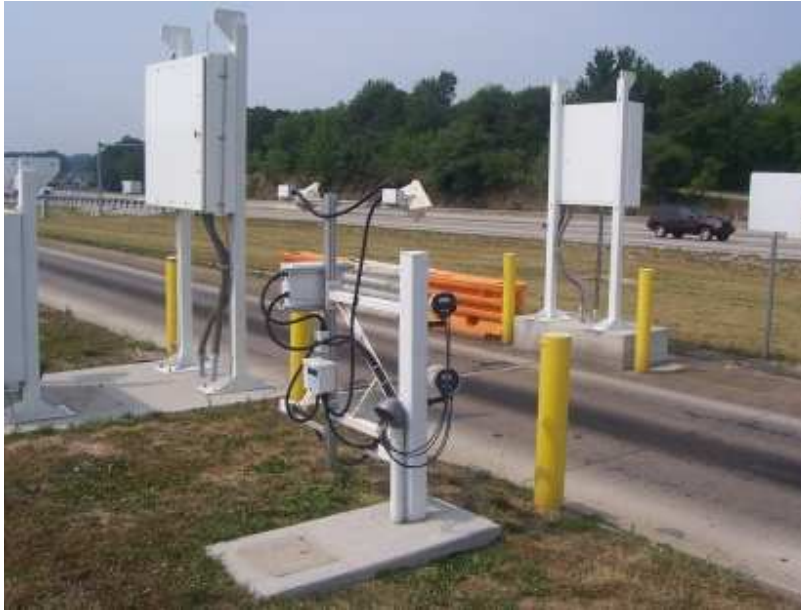
Figure 5-7. Rear view of USDOT number reader camera (at center foreground, on narrow post below two light fixtures). Two ALPR cameras are on larger post at right of USDOT camera.
