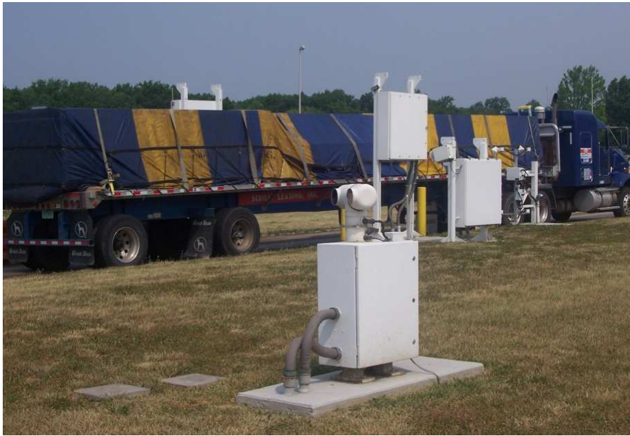
Figure 1-1. London, Kentucky, northbound I-75 weigh station (Laurel County). ISSES thermal inspection cameras in foreground and portal monitor/automated vehicle identification system in background.
