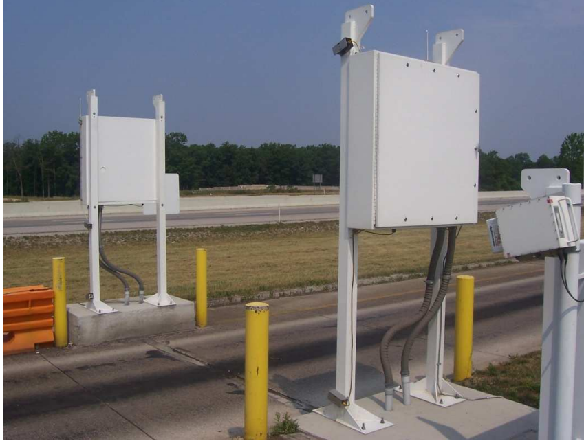
Figure 5-2. Laser scanner for triggering and classification (far right) and raised radiation portal monitors (left and center-right).
