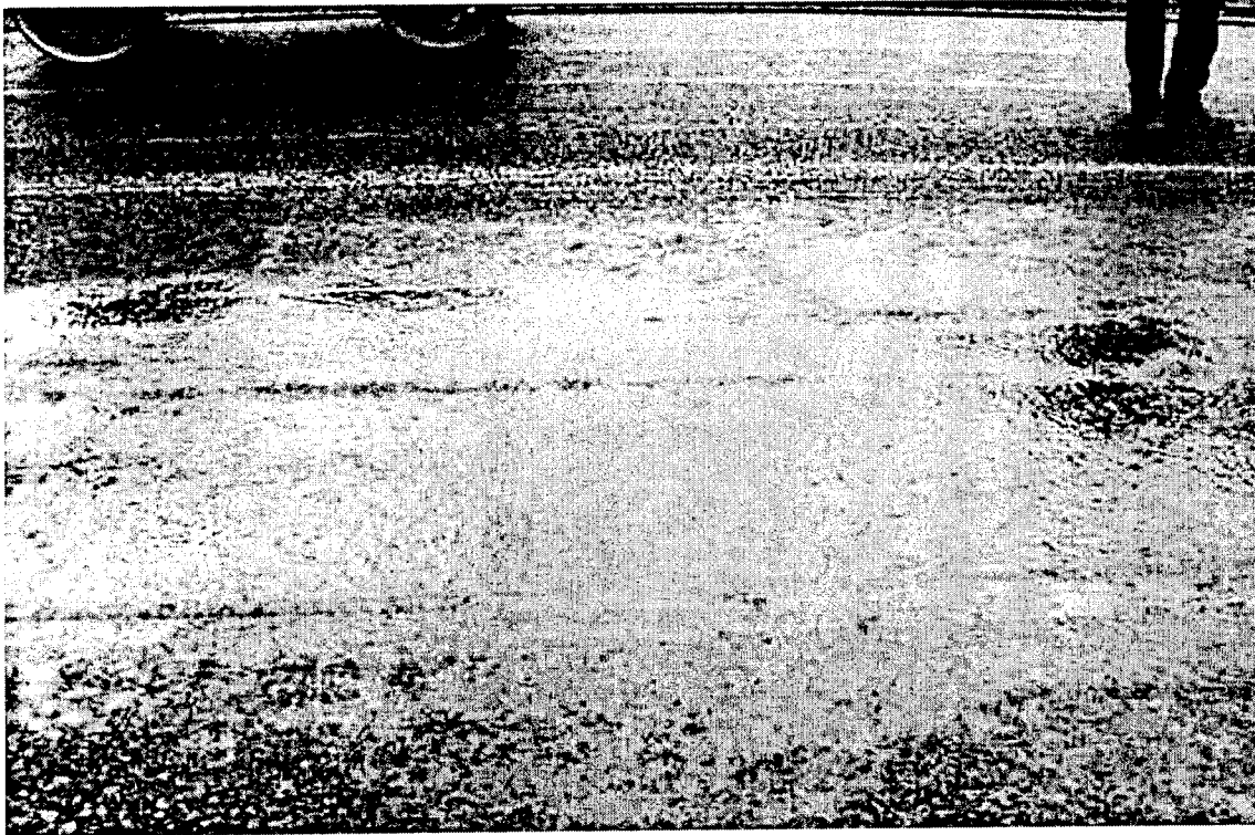
Figure 4.1 Bleeding of Bottom Ash Pavement.
