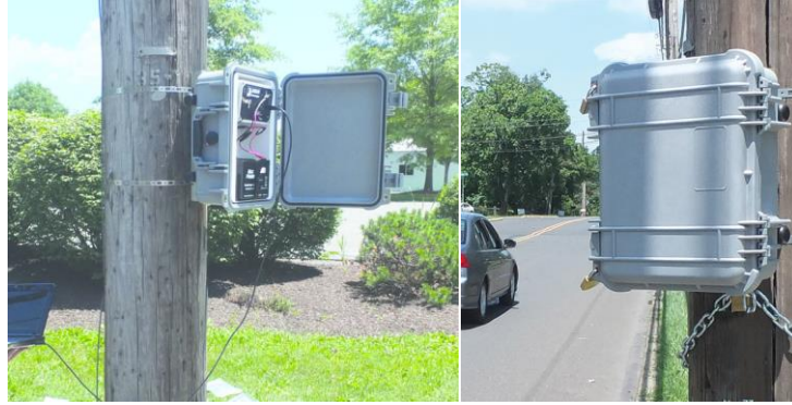
Figure 4.5: Equipment setup including (a) JAMAR radar recorder during setup (b) JAMAR radar recorder in use
