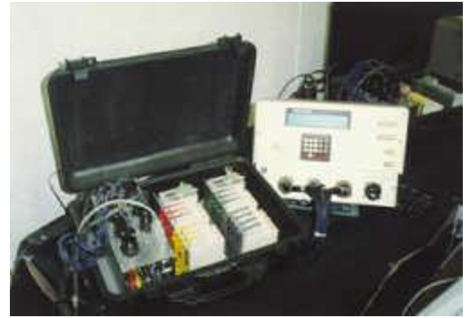
A controller interface device is connected to a NEMA controller.
