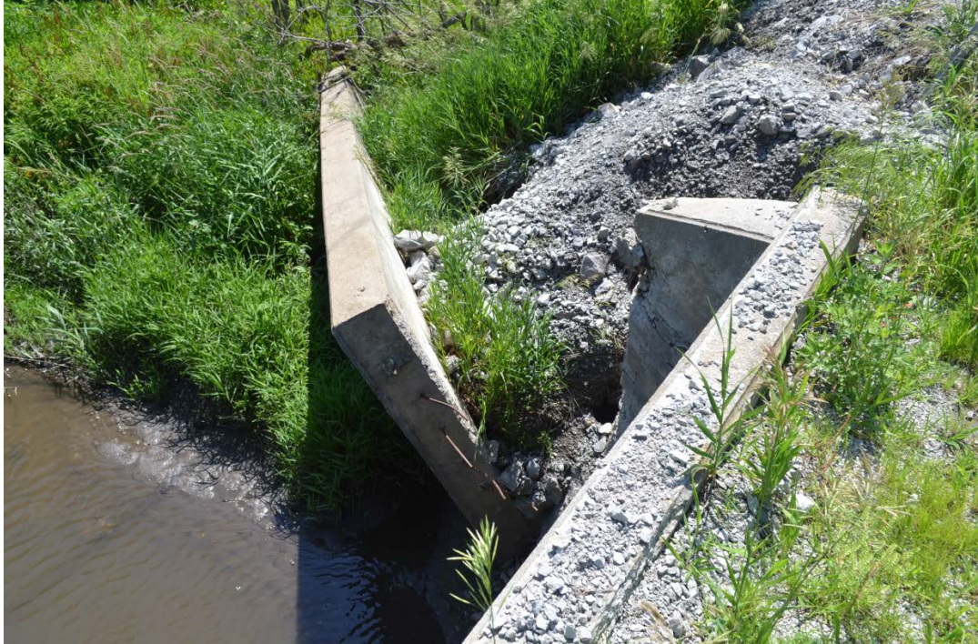
Figure 3.7: RS 25 Bridge Wingwall Failure (2015)
