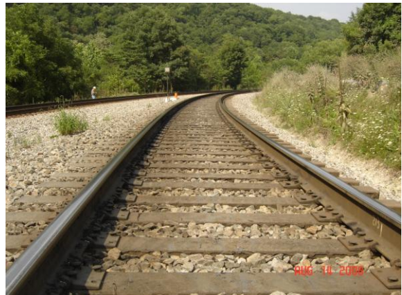
Figure 1. Plastic Composite Tie Test Zone at the NS Revenue Service Mega Site
