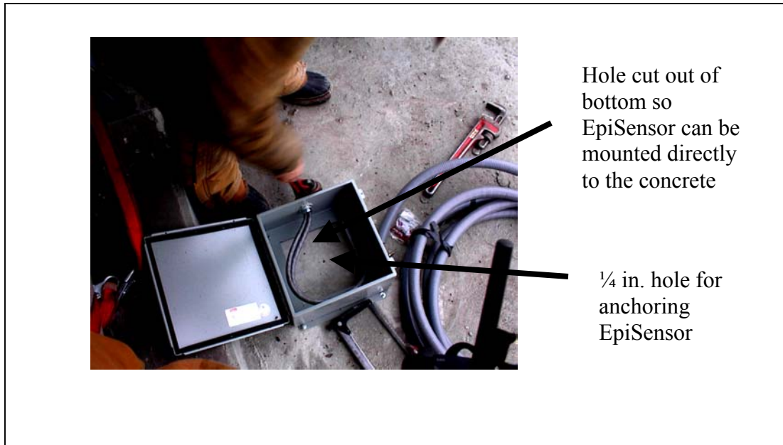
FIGURE 10 Nema 12 enclosure installation
