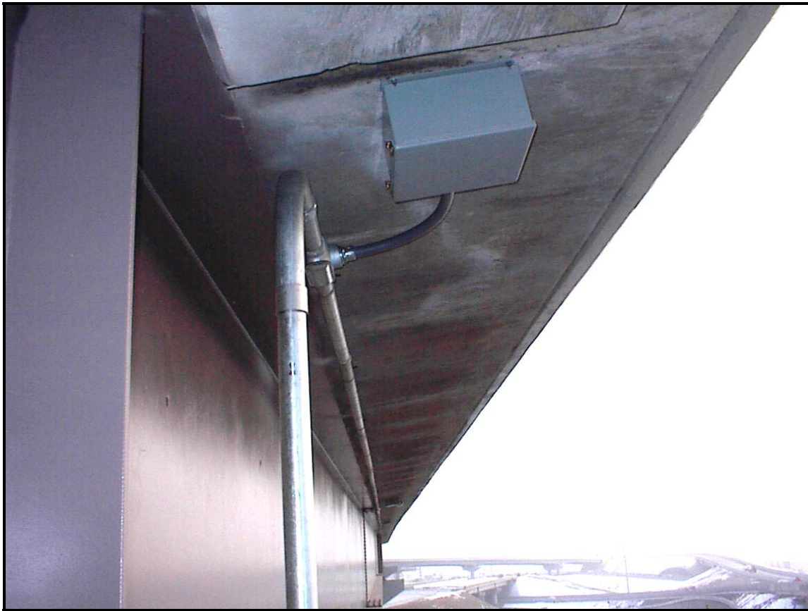
FIGURE 8 Box mounted on bottom of deck
