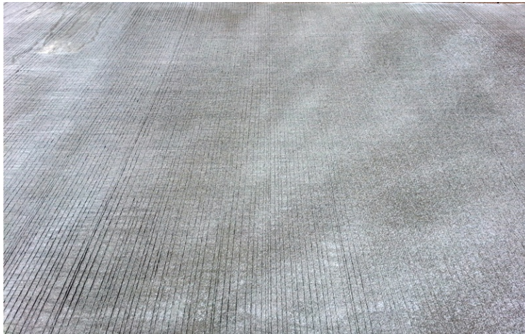
Figure 7.7 The water-wax based curing compound applied by the contractor approximately 30 minutes after paving
