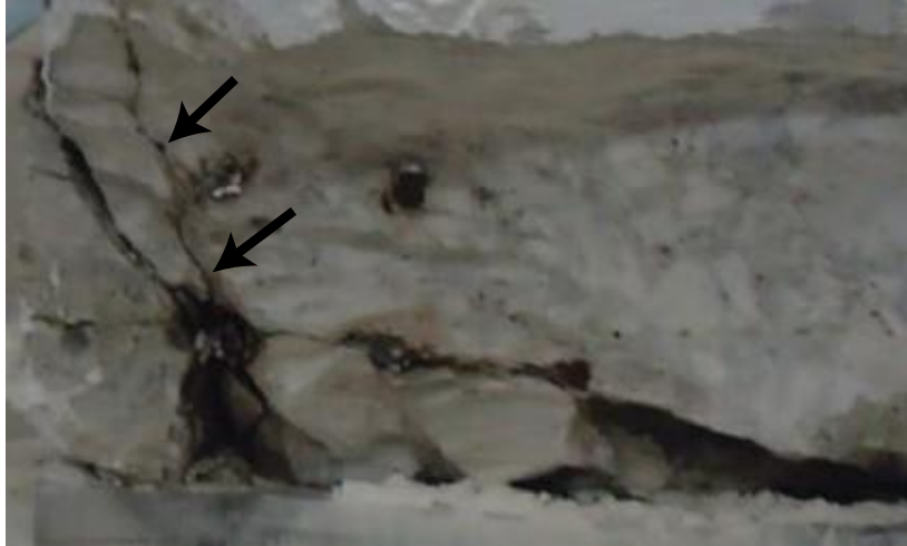
Figure 2.35: Spalling under load initiated by cracking caused by corrosion
