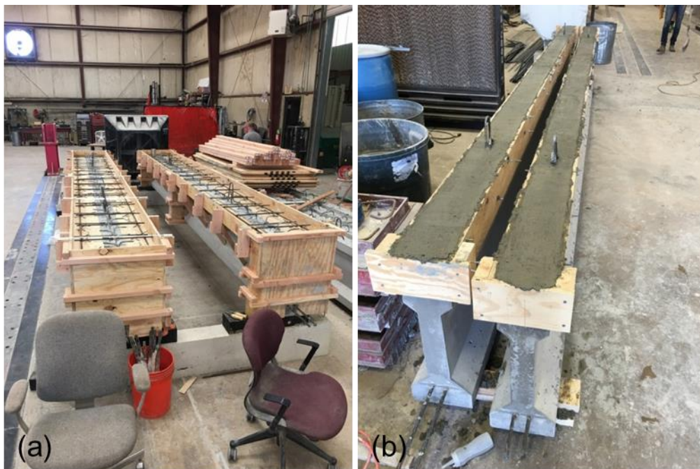
Figure 7.5: (a) Formwork and reinforcing steel for individual girder C sections and (b) formwork and cast concrete for individual scale girder A sections
