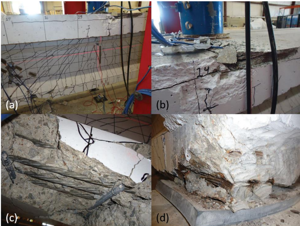
Figure 2.40: Final condition of Girder “C”: (a) shows overall condition, (b) shows crushed deck concrete, (c) shows exposed strands under bottom flange, and (d) shows strand slip of about one inch and corrosion
