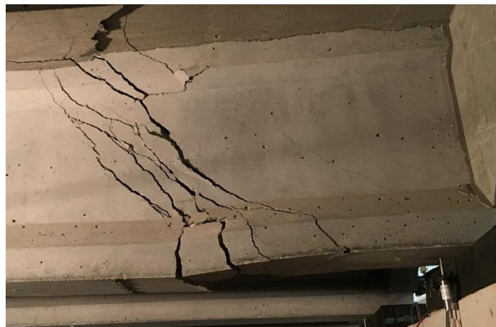
Figure 7.36: Shear cracking of loaded girder at failure
