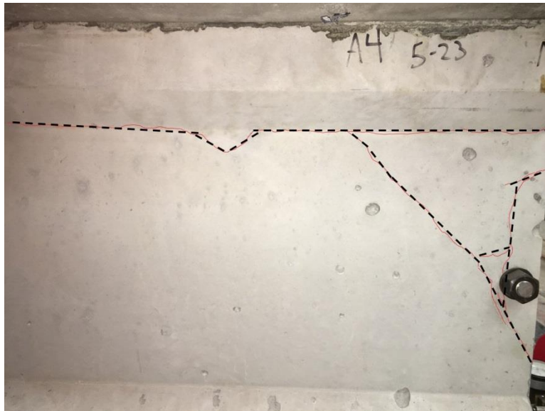
Figure 7.33: Cracking at the diaphragm to girder connection for the exterior girder nearest the load point
