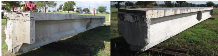
Figure 2.10: Two views of girder C showing details of condition on October 8, 2013
