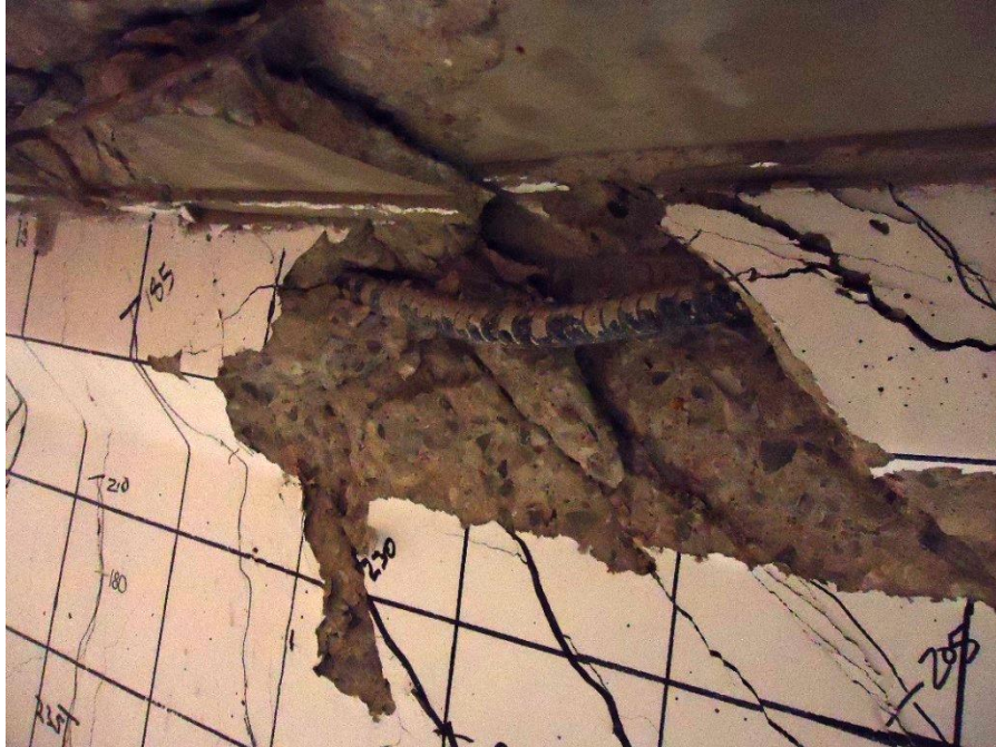
Figure 2.48: Buckled compression steel in girder
