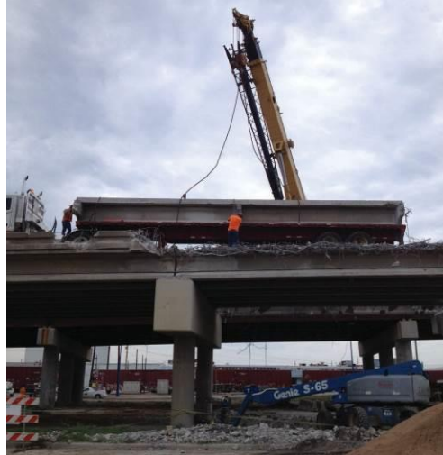
Figure 2.5: Removal of girder C from the I-244 bridge over the Arkansas river in Tulsa, OK on September 4, 2013 (photo courtesy of Gary Quinonez with Manhattan Road & Bridge)
