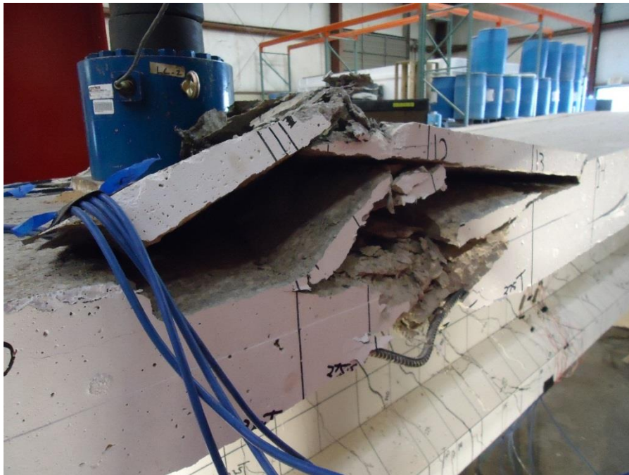
Figure 2.47: Buckled steel and failure along plane of wearing surface
