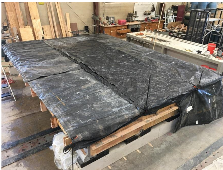
Figure 7.14: Plastic and burlap used for curing concrete deck on scaled bridge section
