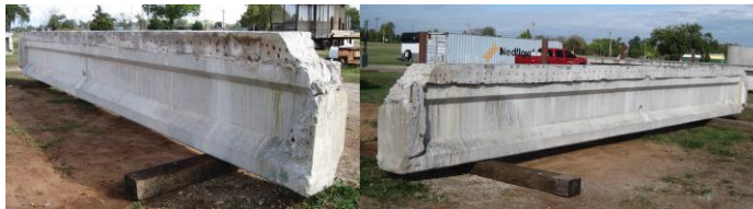
Figure 2.9: Two views of girder A showing details of condition on October 8, 2013
