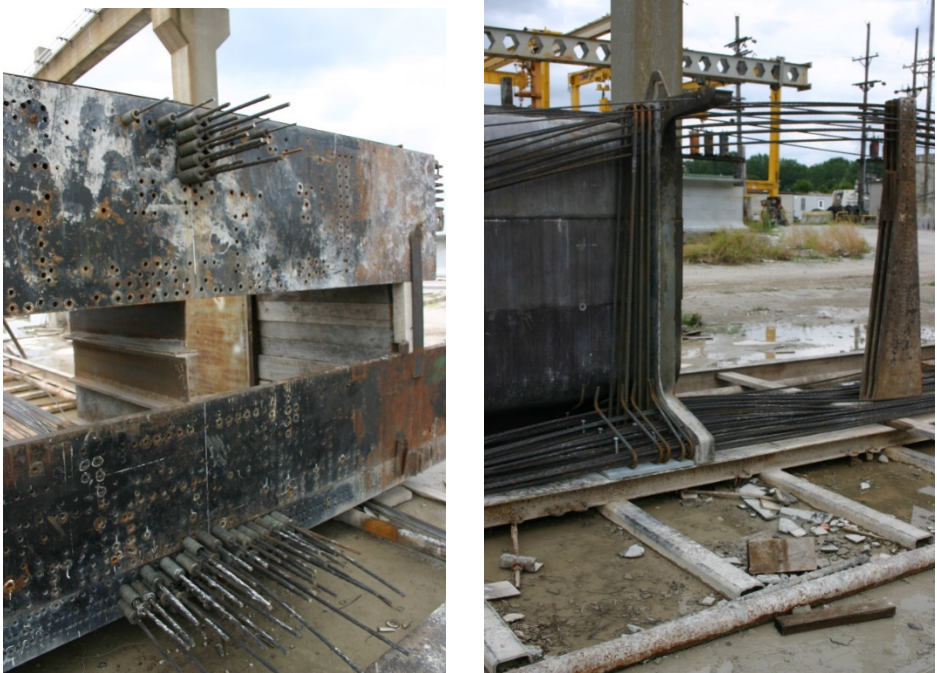
Figure 6.4: Steel Bulkhead for Pretensioned Strand (left) and Placement of Mild Steel Reinforcement at Girder End (right)
