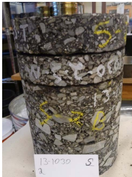
Figure 8. Debonding Shown in a Core From Site S (US 58 in Carroll County)
