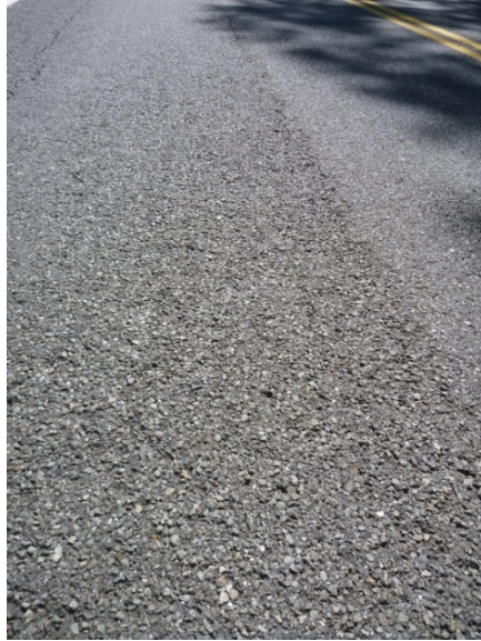
Figure 5. Raveling Observed in Site Q, US 11 in Montgomery County
