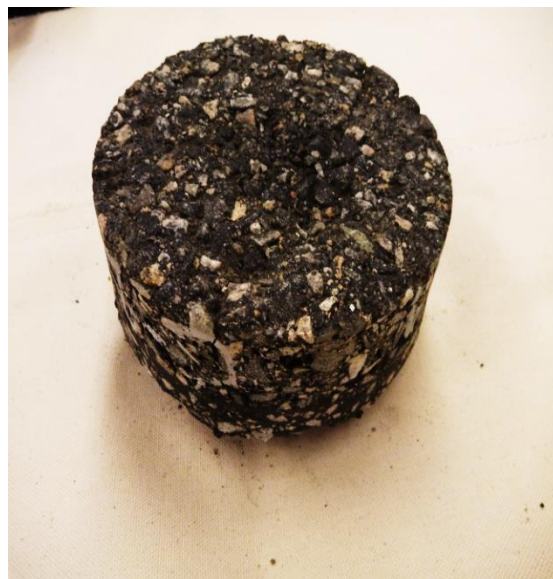
Figure 4. Mixture Raveling in a Core From Site C, CR 703 in Dinwiddie County
