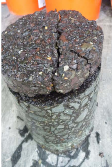
Figure 3. Cores From Sites H and I (SR 211 in Rappahannock County) Showed That Cracking Was Initiating From the Top Down
