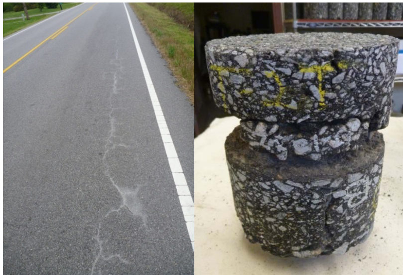
Figure 10. Pumping of Fines and Moisture Damage in a Core From Site T (SR 671 in South Hampton County)
