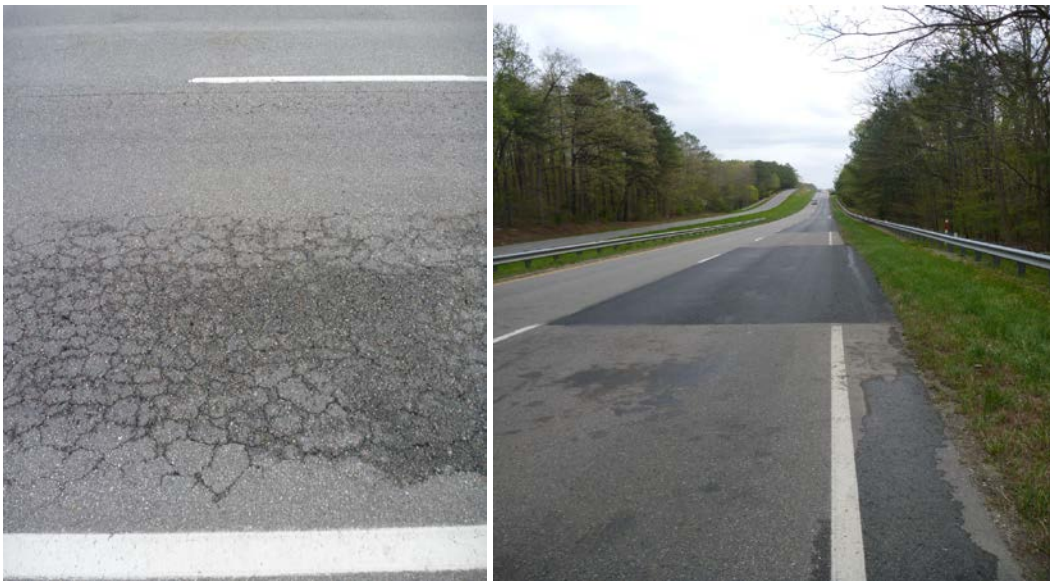
Figure 2. Cracking and Patches on Section A, SR 6 in Goochland County
