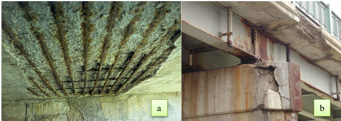
Figure 2.1 (a) Common bridge deterioration caused by corrosion, (b) bridge deterioration with deterioration of the support
