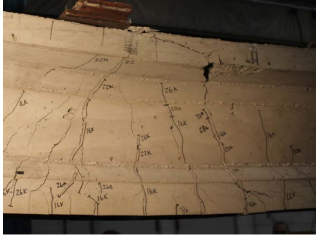
Figure 34. Top Flange Compression Failure of Specimen 1 Typical Steel Reinforcement
