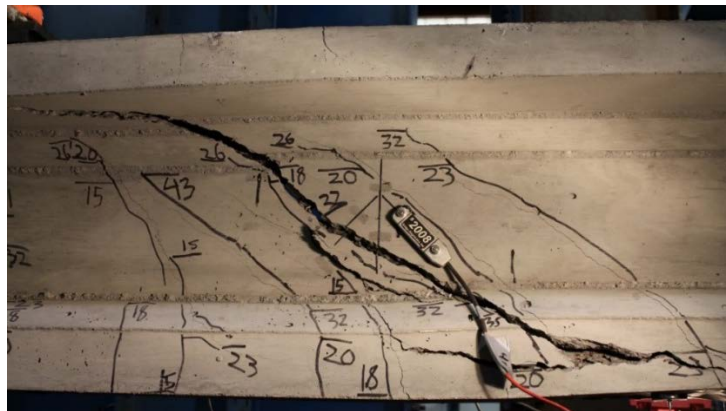
Figure 54. Shear Failure of Specimen 4 with Two Layers of C-Grid Zip Tied Together
