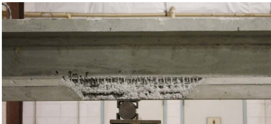
Figure 18. Honeycombing in Three Layers of C-Grid
