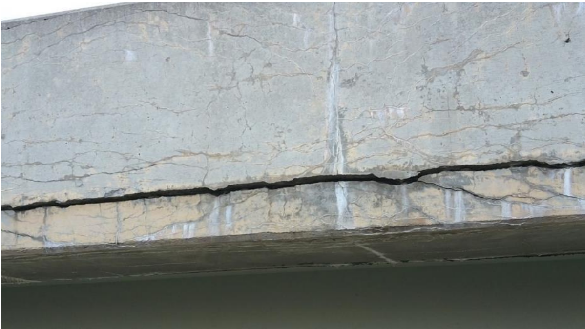
Figure 5.22 Cracks and Possible Delamination on the Southern Barrier, E036
