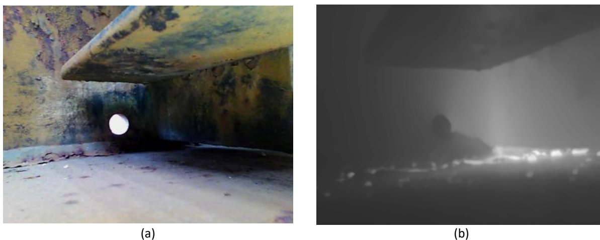
Figure 6.29 (a) A visually undetectable fatigue crack, and (b) fatigue crack detection using active thermography
