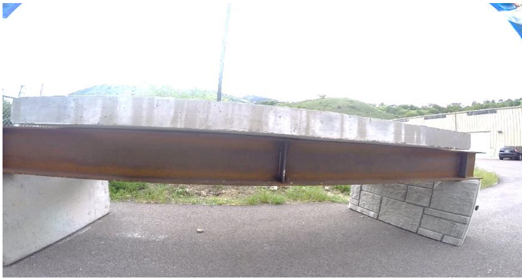
Figure 3.7 Steel Girder Surface Corrosion and Rust in the Image Acquired by UAS, E004
