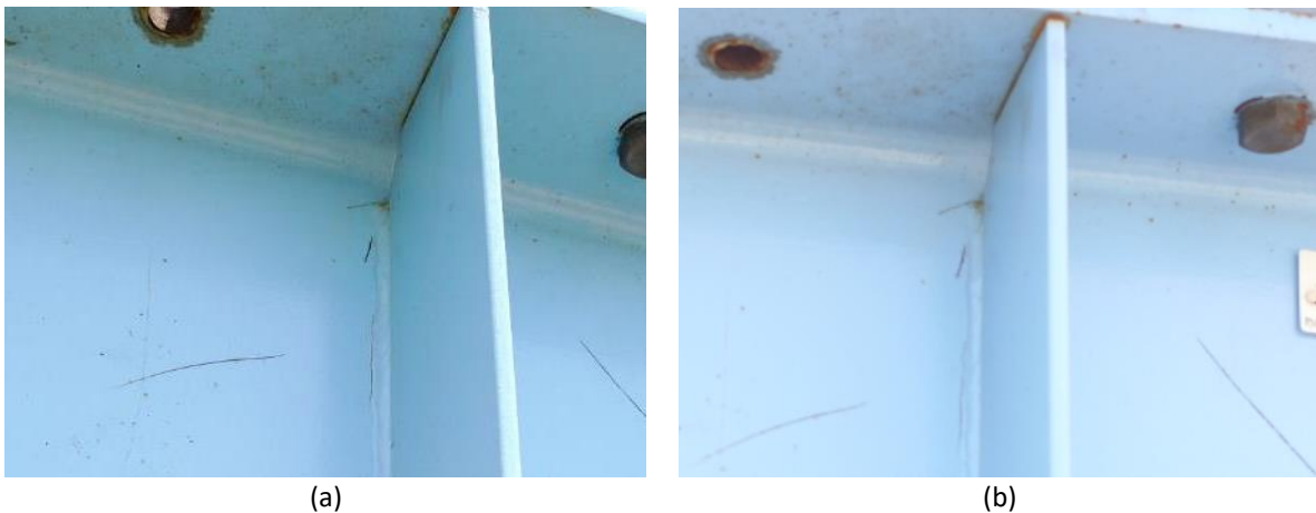
Figure 6.23: (a) 1 fatigue crack reported on top-left in the DJI Mavic images and (b) 2 fatigue cracks reported on top-left in the DJI Inspire images
