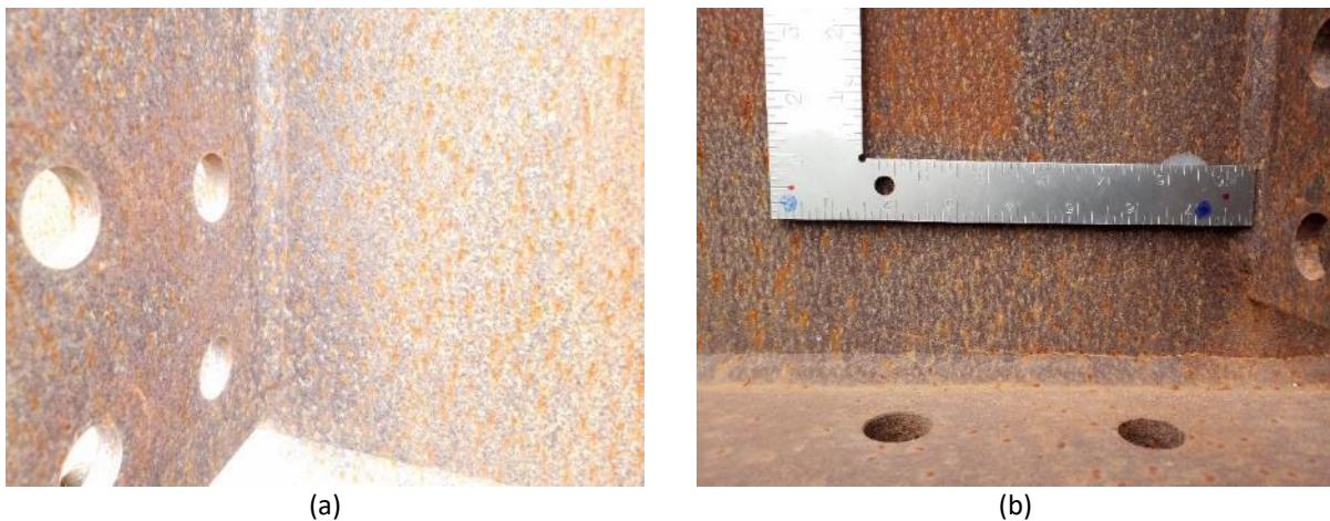
Figure 6.30 Known manufactured fatigue cracks which were (a) small and undetectable visually and (b) large and detectable visually
