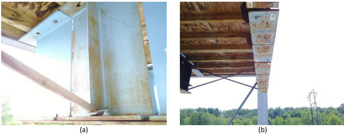
Figure 6.8 DJI Mavic images: (a) a girder in the POD frame with possible fatigue crack and (b) bottom flange cover plates
