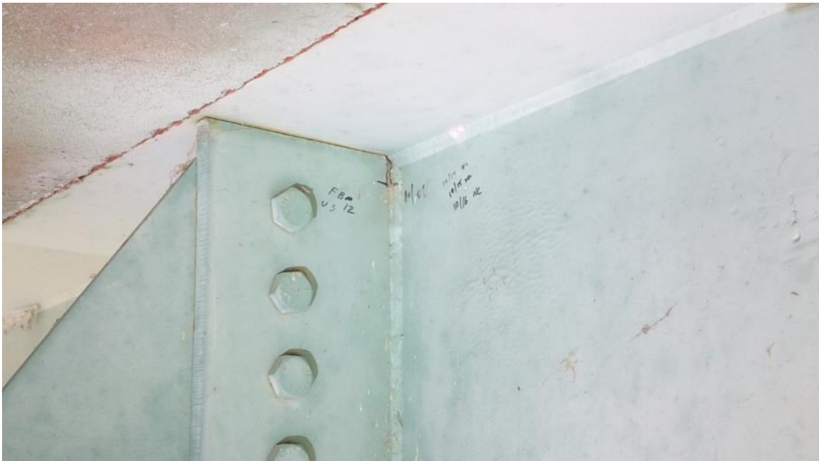
Figure 5.14 Defect (Crack) on the Fourth Floor Beam, E031
