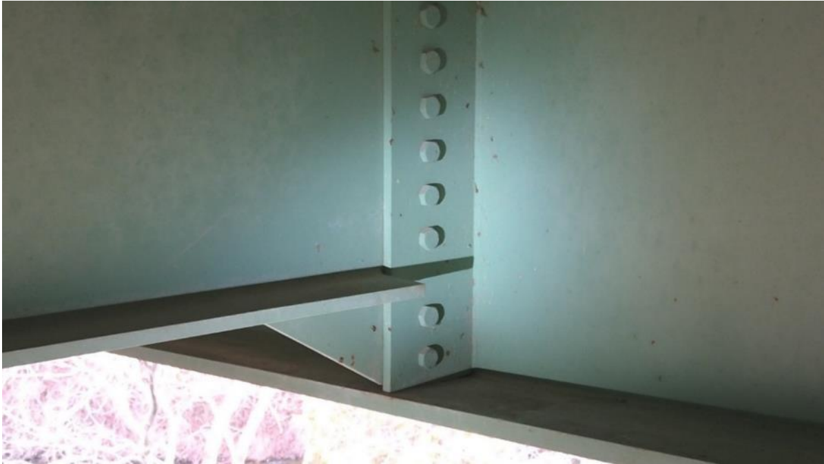
Figure 5.11 No Cracks on Second Floor Beam on East, Southern Corner, E023
