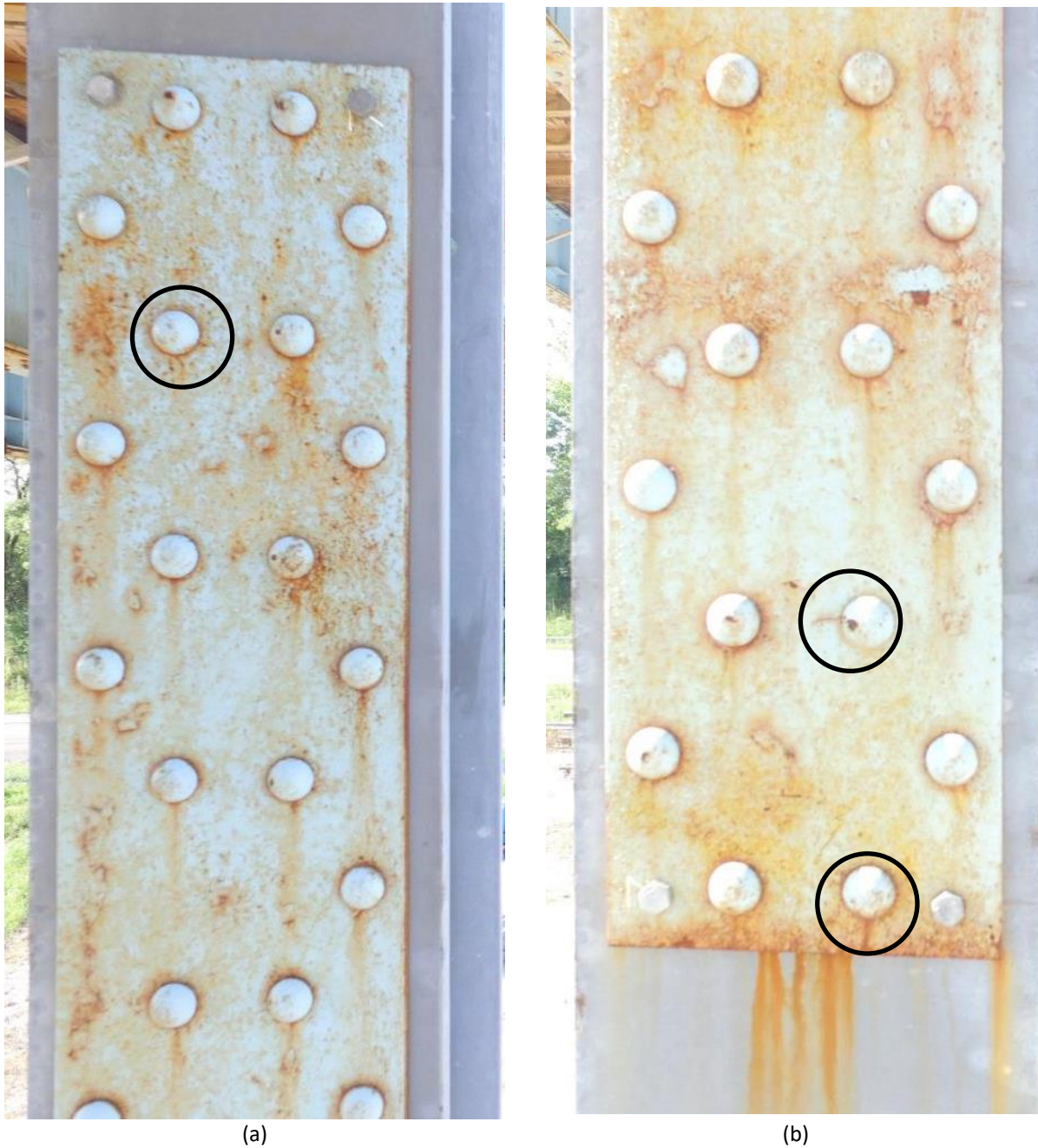
Figure 6.26 Images of the riveted cover plate specimen (a) reported crack on row 3 and (b) reported cracks on row 25 and 27
