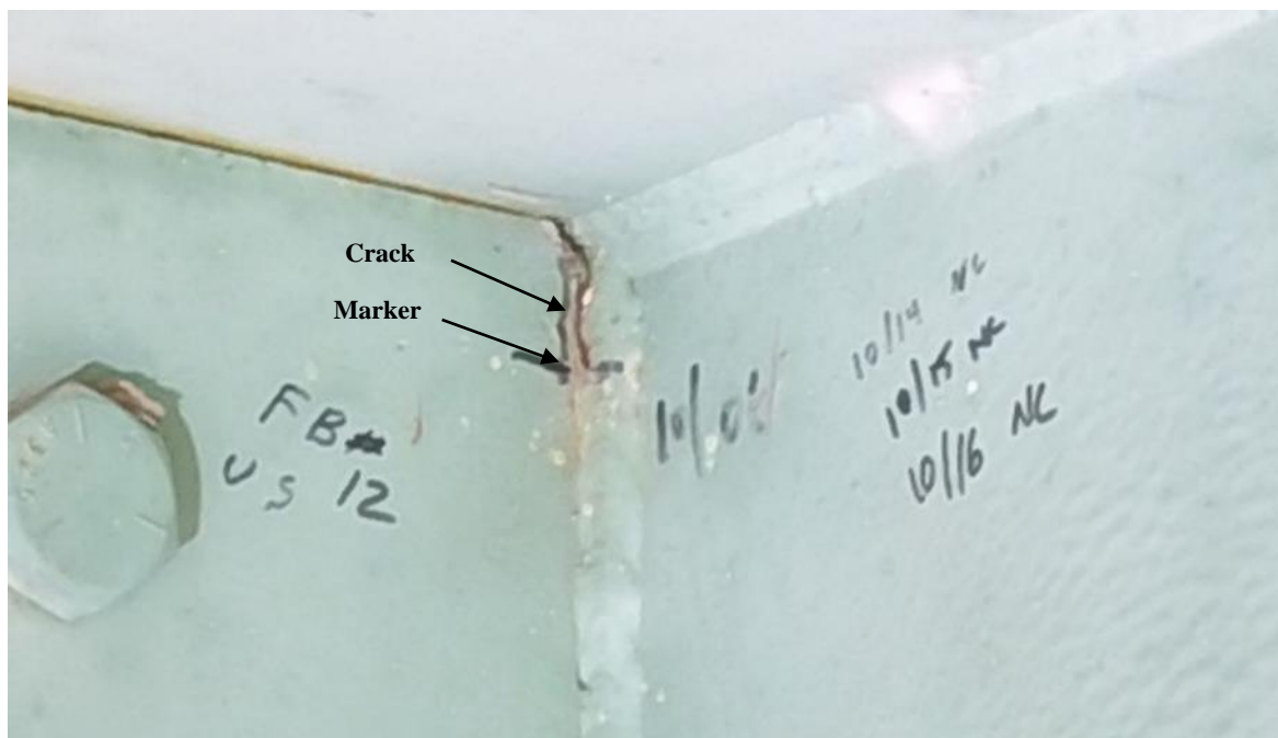
Figure 5.15 Zoomed Image from the Fatigue Crack, E031
