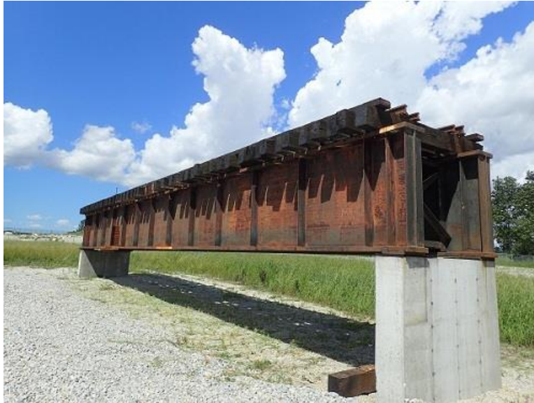
Figure 6.3 Railroad bridge with known fatigue cracks
