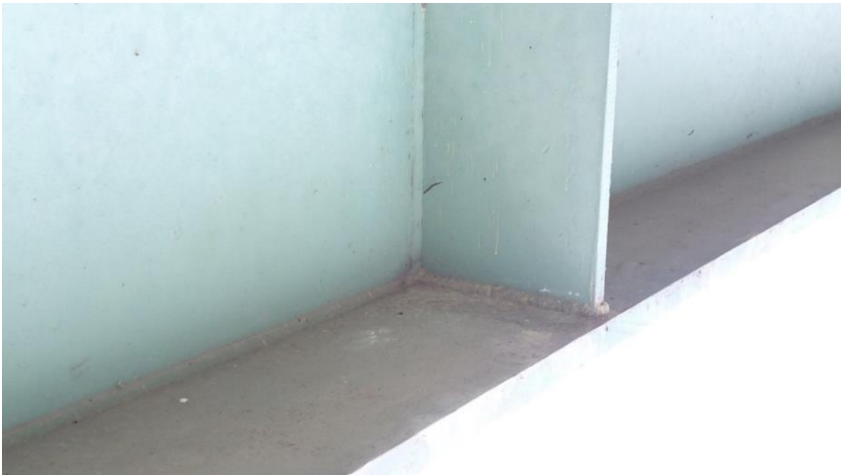
Figure 5.18 No Defects (Crack) on the Fourth Floor Beam, Southern Corner, Bottom Flange Weld, E032
