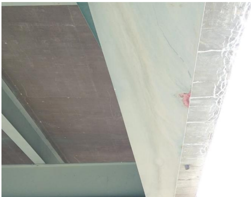
Figure 5.23 Minor Corrosion on Bottom Flange of the Southern Girder, E035 and E036
