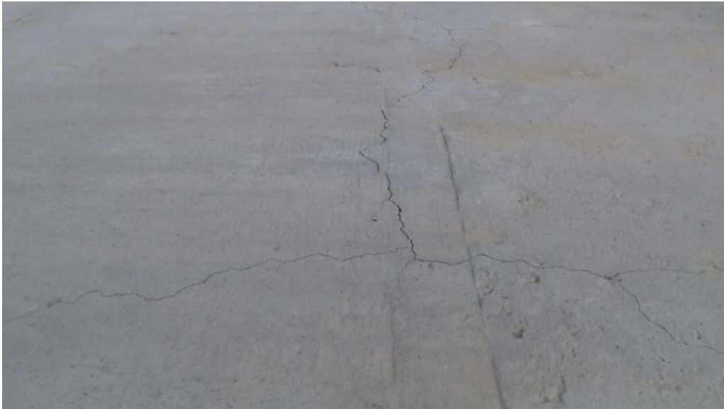
Figure 3.2 Example of Top Cracks in the Color Image Acquired by the UAS, E001
