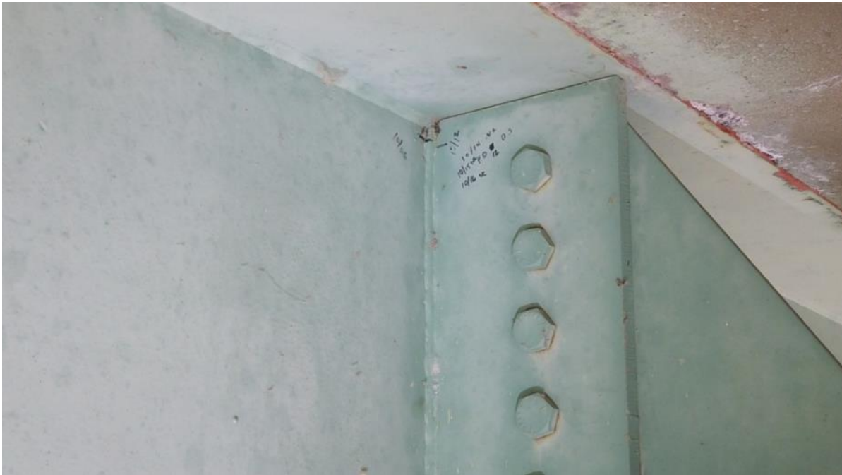
Figure 5.16 Defect (Crack) on the Fourth Floor Beam, Southern Corner, E032
