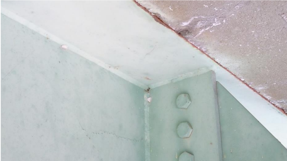
Figure 5.13 Third Floor Beam on East, Mild Rust, Northern Corner, E027
