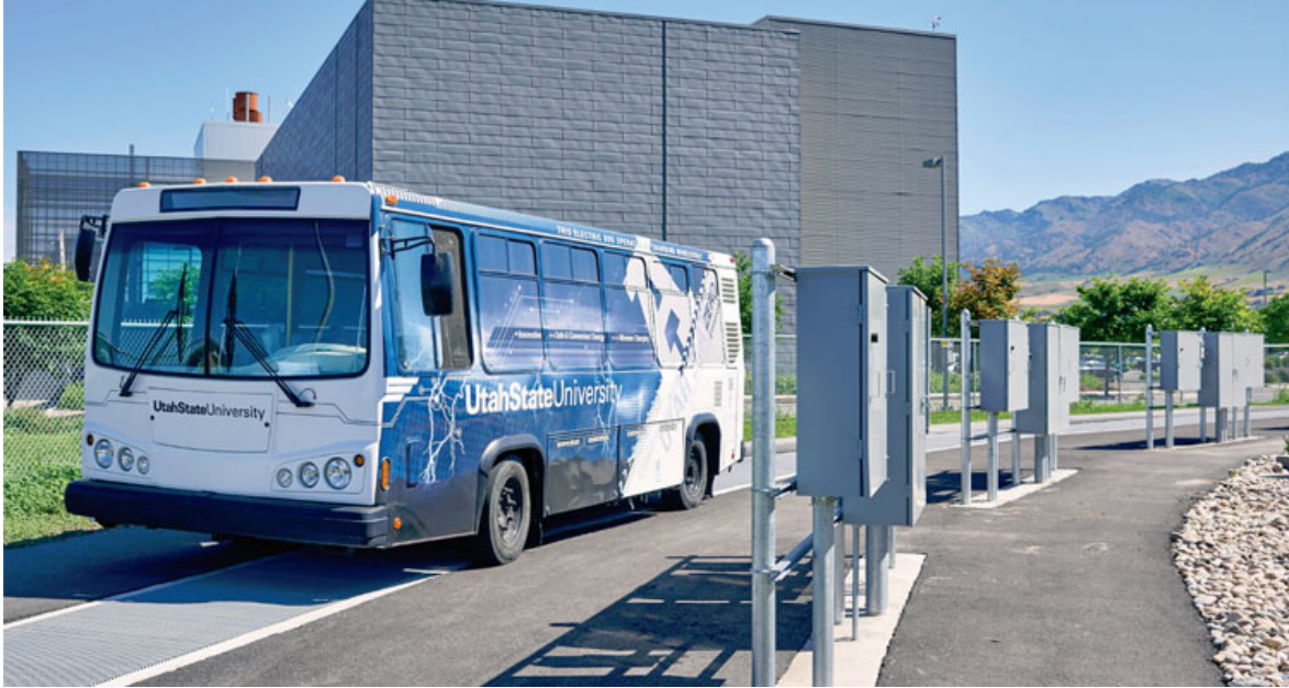
Figure 2.2 EVR Test track and Power Panels
