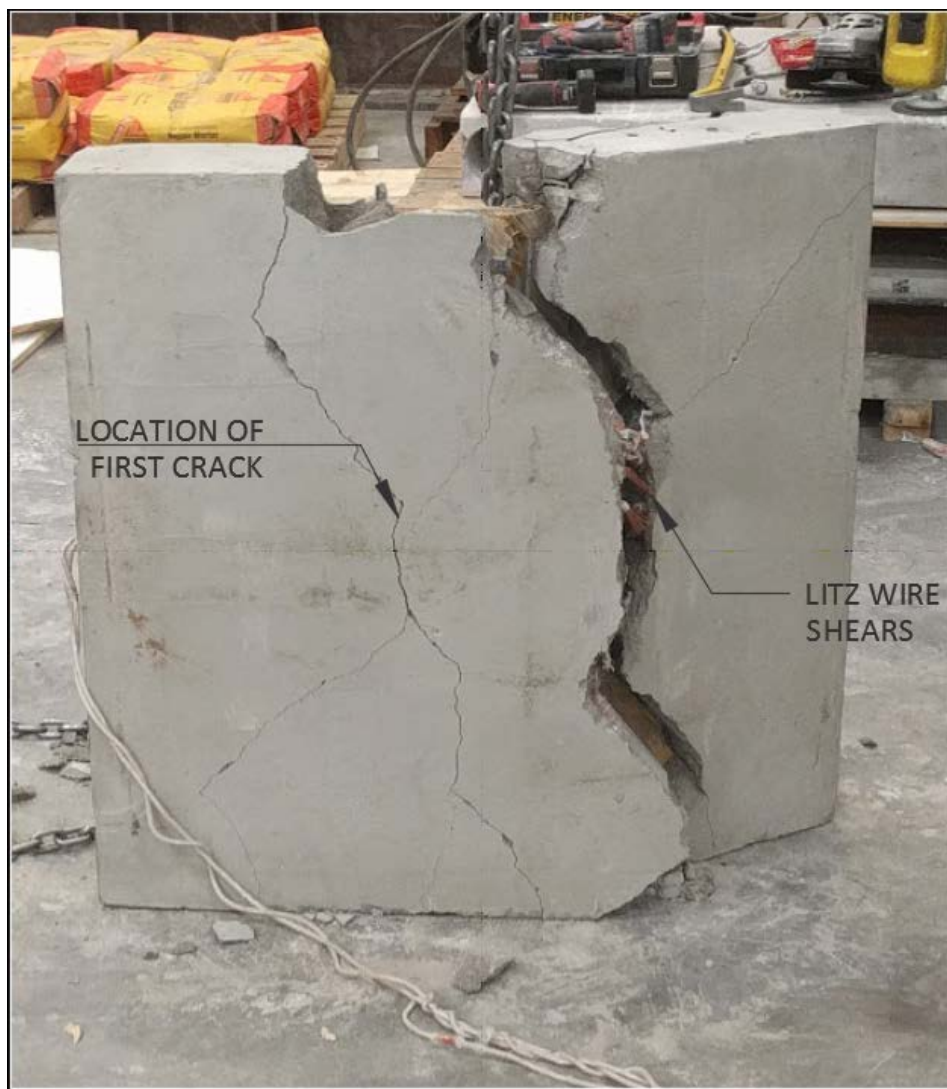
Figure 4.9 First pad post failure
