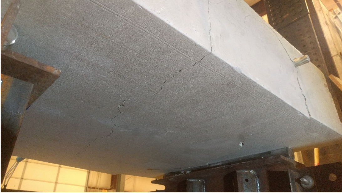
Figure 4.25 Crack 1/2 inch wide
