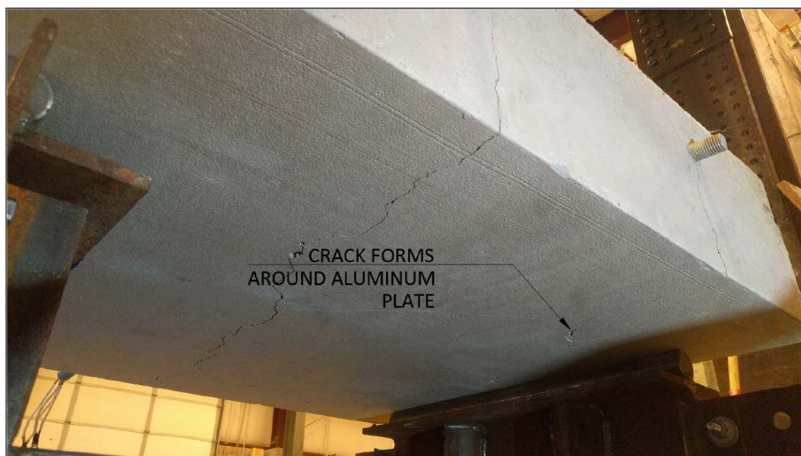
Figure 4.24 Crack 1/4 inch wide
