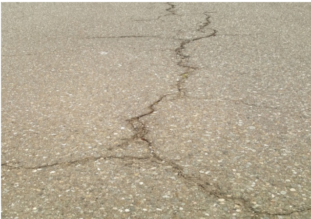
Figure 125. OR3a, SR101, Poor category, age 62 months. No maintenance as of the 2017 inspection.
