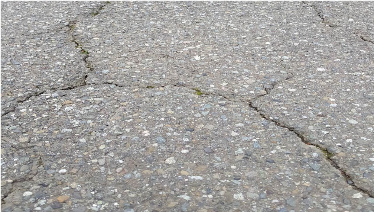
Figure 132. OR3a, SR101, three years after the other section were treated. Cracks are wide but not spalling.
