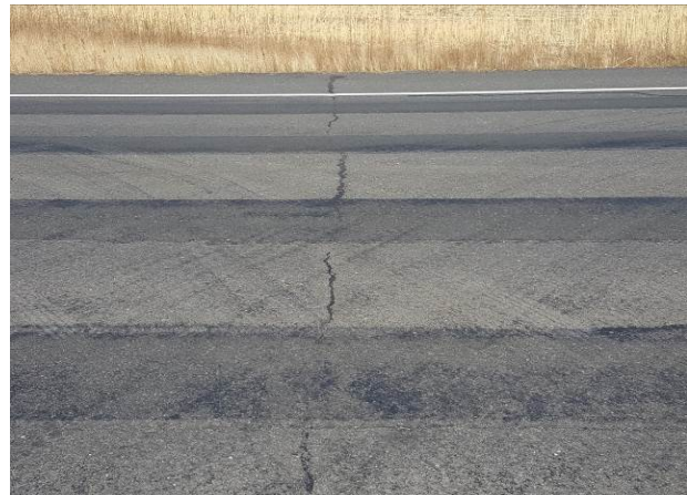
Figure 39. ER10, US2, Good, age 36 months. Cracking noted at 12 months. Loss of aggregate in both wheel paths.
