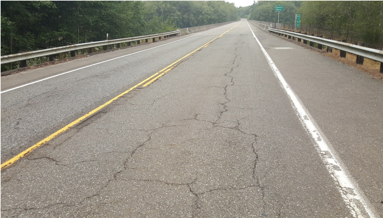
Figure 134. OR3a, SR101, five years after the other sections were treated. Cracks are wide and beginning to spall.
