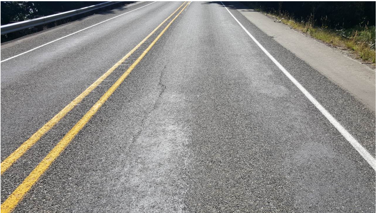
Figure 29. OR1b, SR101, five years after installation. Longitudinal crack condition is about the same, slight rutting and flushing in the wheel paths.
