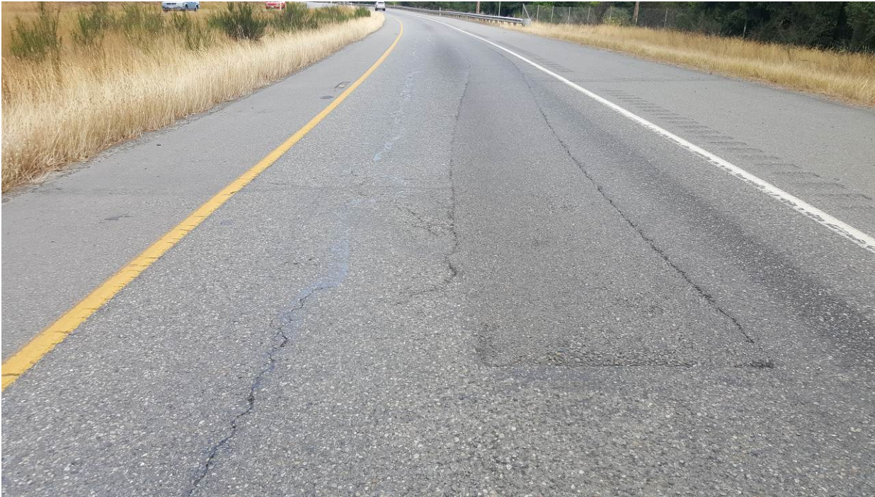
Figure 99. OR4, SR3, four years after installation. No change in dig out patch or crack sealing.
