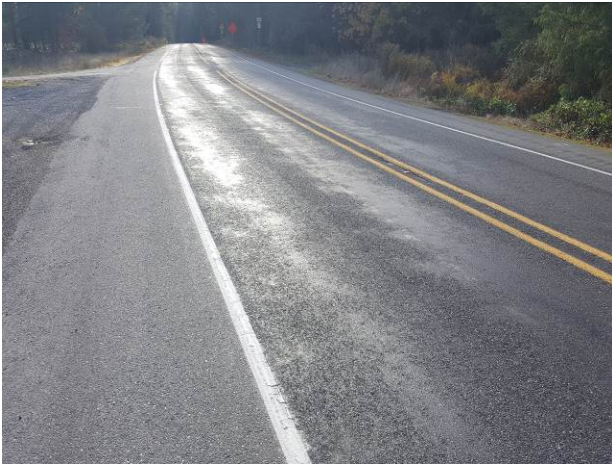
Figure 104. OR14, SR7, Good, age 51 months. Dig out patches flushing through the chip seal at 27 months.
