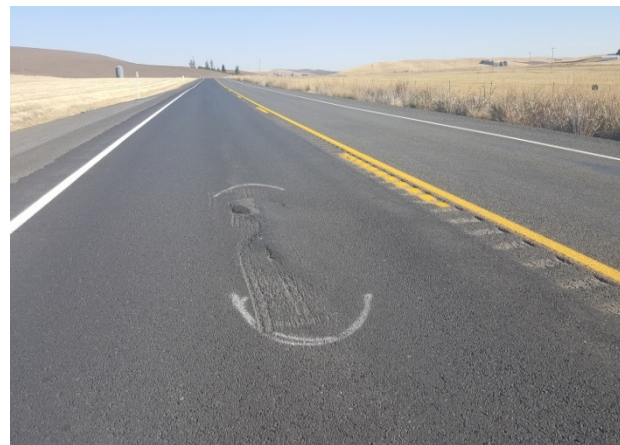
Figure 115. ER26, SR127, Good, age 26 months. Pot hole formed in 2016. Flushing in wheel paths noted in 2017.
