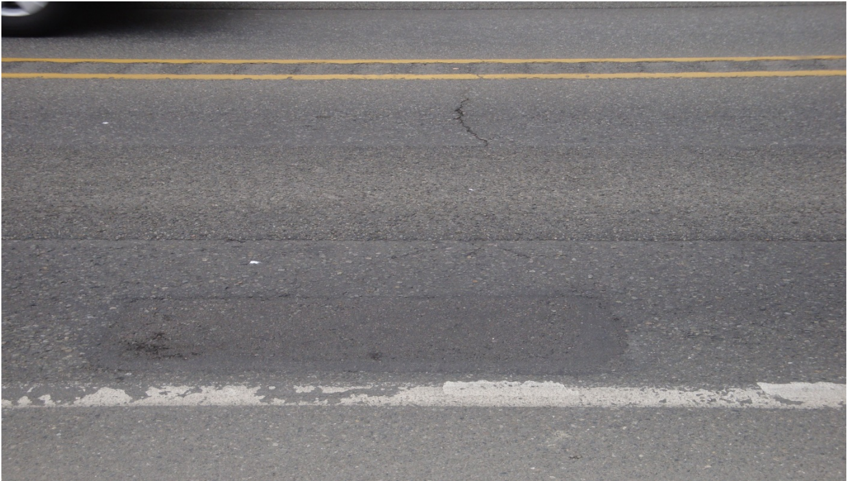
Figure 36. OR12, SR20, three years after installation. Some loss of aggregate but no reflection cracking.
