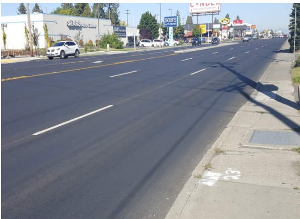
Figure 127. ER2a, US2, Poor category, age 62 months. Dig outs, crack sealing and patching were necessary to preserve the roadway. HMA grind/inlay in 2017, C9063.
