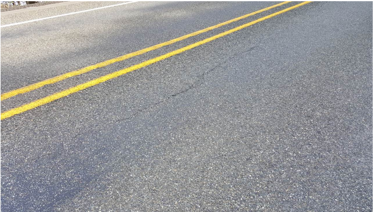
Figure 27. OR1b, SR101, three years after installation. Longitudinal crack is getting longer and wider. Flushing in the wheel paths is about the same.
