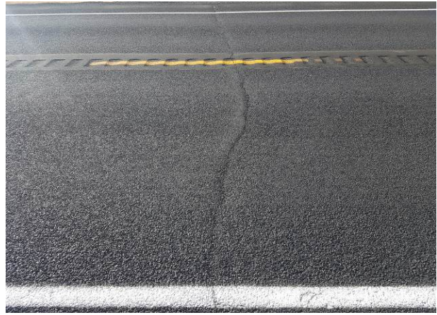
Figure 49. NC1, SR155, Good, age 38 months. Transverse crack locations are depressed and very thin cracks are present.
