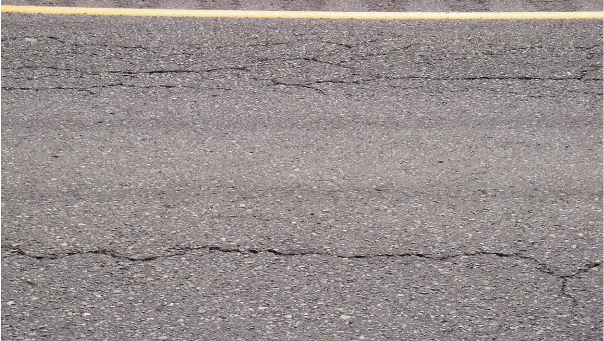
Figure 14. OR1, SR101, prior to treatment. Cracks exceed 1/4 inch in width in places.
