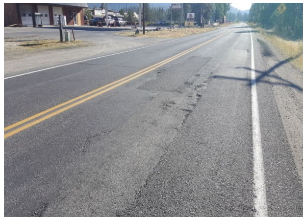
Figure 128. ER3a, SR291, Fair category, 62 months. Dig outs, crack sealing and patching were necessary to preserve the roadway. HMA grind/inlay scheduled in 2018, C9223
