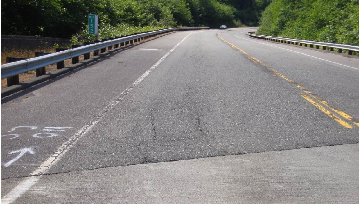
Figure 129. OR3a, SR101, condition in 2012, the year that the other sections were treated.
