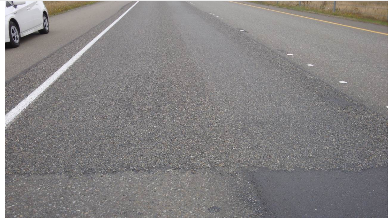
Figure 107. OR2a, SR8, one year after installation. Slight flushing in the wheel paths over the dig out patches.
