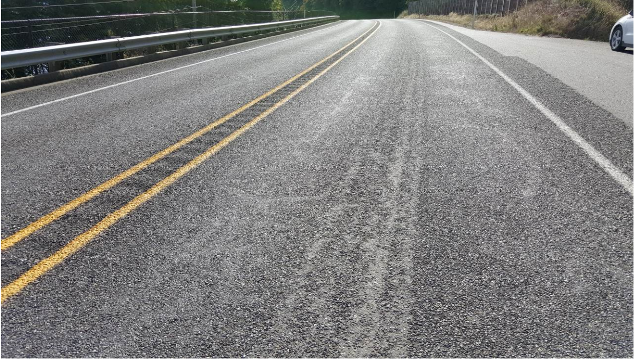
Figure 53. OR1a, SR101, three years after installation. Very slight flushing and shadowing of the sealed cracks.
