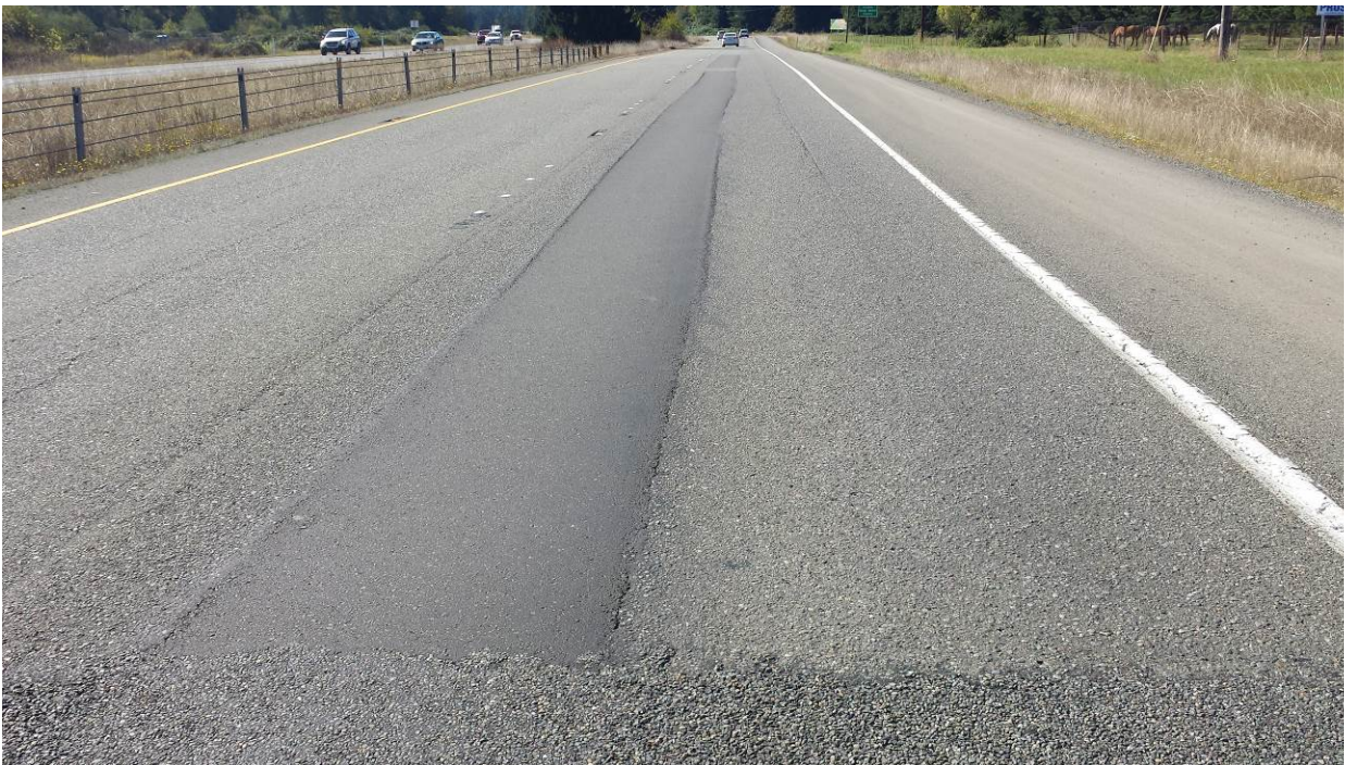
Figure 80. OR2, SR8, two years after installation. No change in condition of patch.
