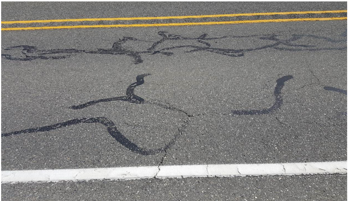
Figure 19. OR1, SR101, five years after installation. The cracks are beginning to appear through the sealant where the original sealant was minimal.
