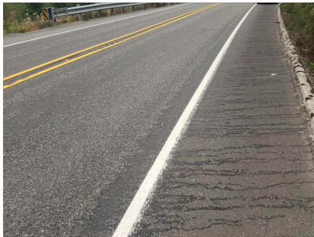
Figure 23. OR22, SR101, Good, age 26 months. Loss of aggregate at bottom of super elevation.
