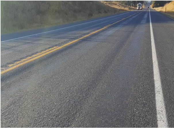
Figure 40. ER15, SR395, Good, age 24 months. Flushing noted in 2017. Transverse reflection cracking noted.
