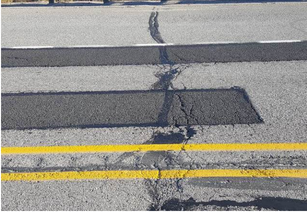
Figure 66. ER9, SR395, Good, age 37 months. Additional dig outs installed in 2015. Transverse reflection cracking noted in 2017.
