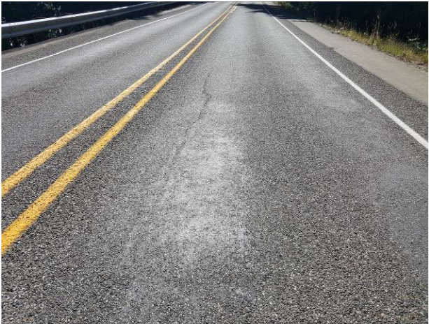
Figure 20. OR1b, SR101, Poor, age 62 months. Longitudinal cracking noted at 21 months. Slight flushing in the wheel paths.
