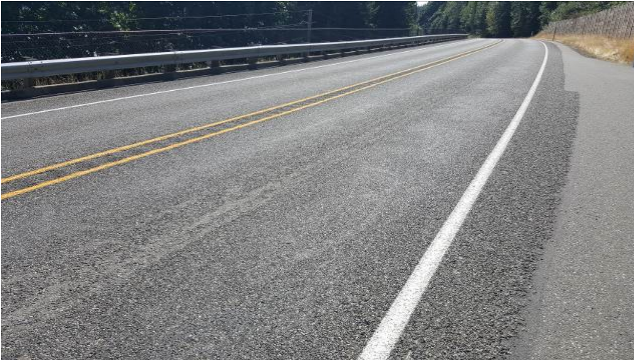
Figure 55. OR1a, SR101, five years after installation. Slight amount of rutting beginning to appear. Flushing not an issue. Shadowing of underlying crack sealant.
