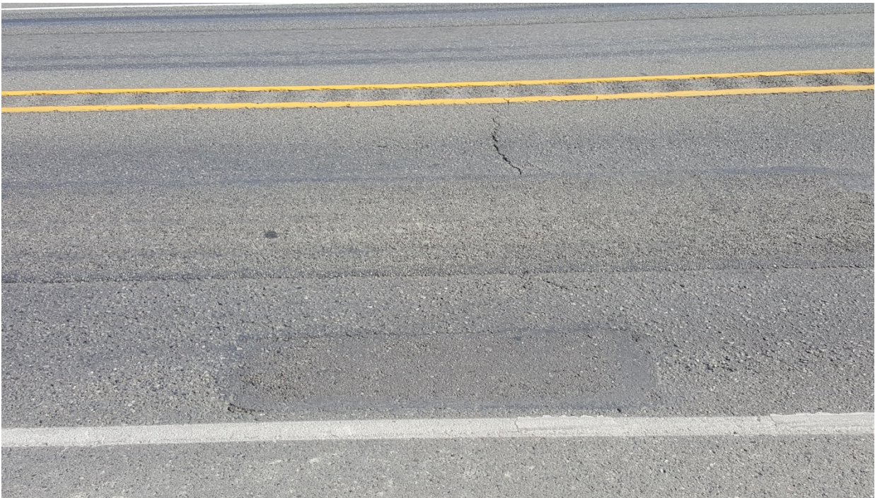
Figure 35. OR12, SR20, two years after installation. Some loss of aggregate but no reflection cracking.
