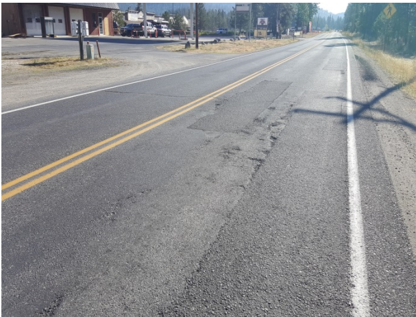
Figure 58. ER3, SR291, Fair, age 62 months. Additional dig outs added in 2015. Transverse reflection crack noted at 10 months after treatment. More dig outs are scheduled for installation in 2017 and a HMA grind/inlay in 2018, C9223.
