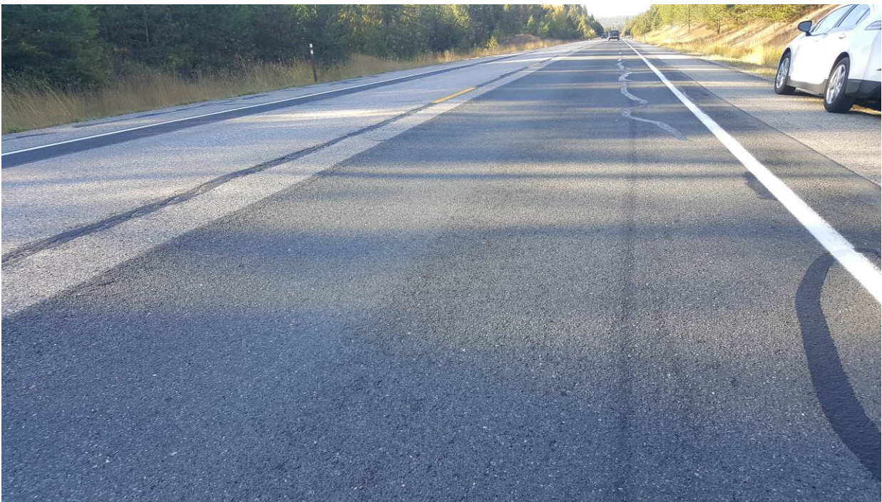
Figure 123. ER9a, SR395, two years after installation. Longitudinal reflection cracking has been sealed. Note slight flushing in the left wheel path.
