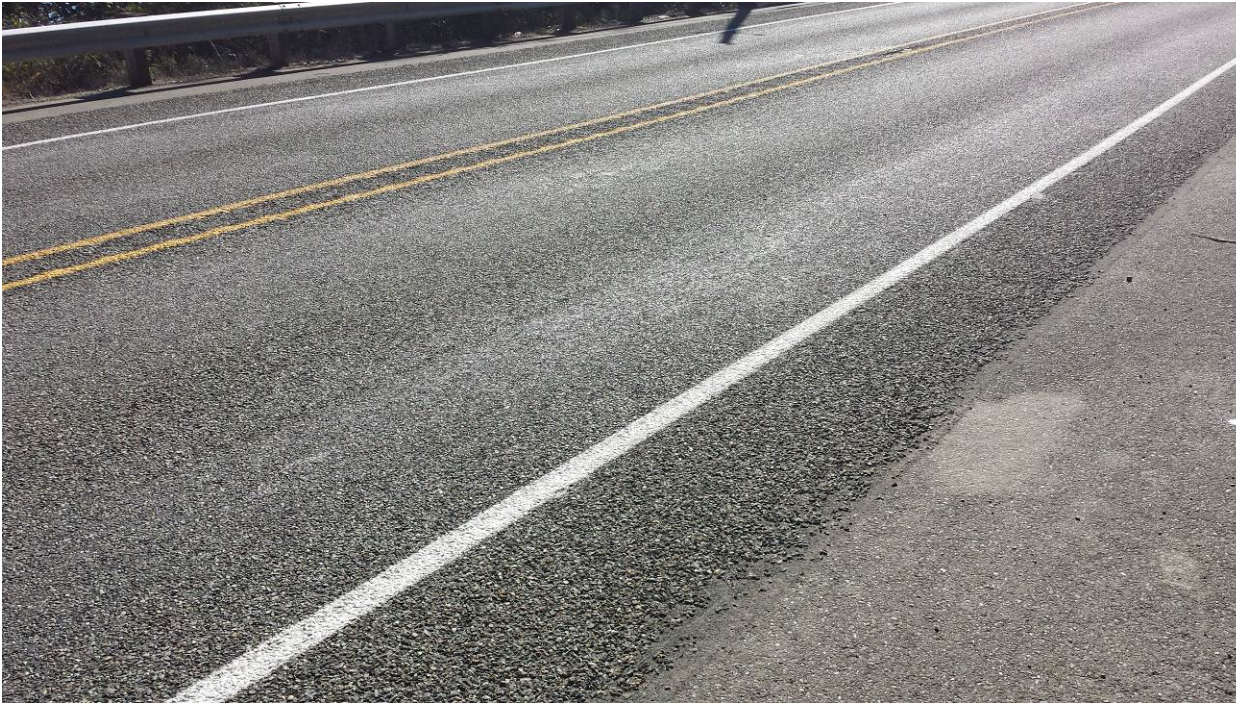
Figure 26. OR1b, SR101, two years after installation. Longitudinal crack appears to have “healed”. Slight flushing in the wheel paths.
