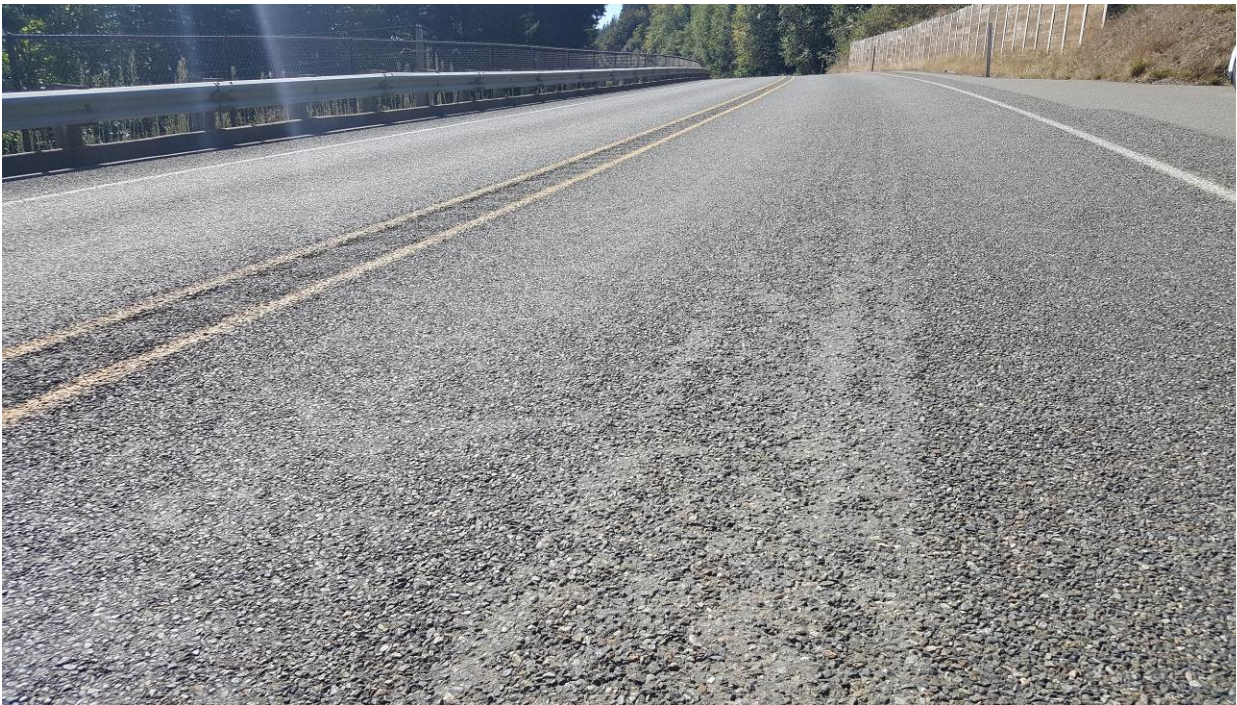
Figure 54. OR1a, SR101, four years after installation. Slight amount of rutting beginning to appear. Flushing does not seem to be a big issue.
