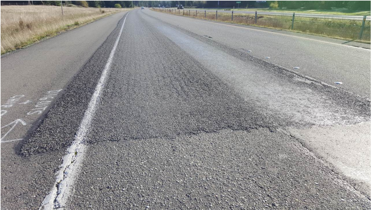
Figure 109. OR2a, SR8, three years after installation. Flushing in the left wheel path throughout the length of the chip seal.
