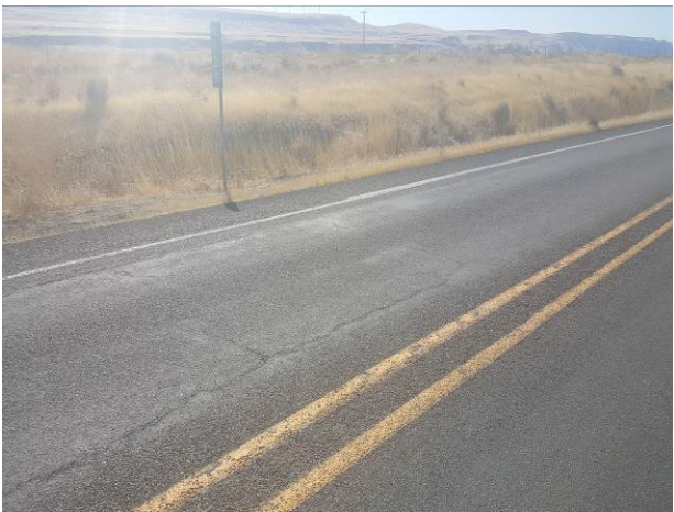
Figure 102. SW1, SR14, Poor, age 62 months. Transverse reflection cracking and flushing noted at 9 months after installation.
