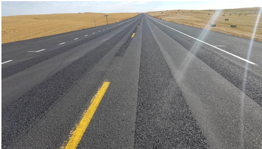
Figure 140. ER10, wheel path chip seal rut filling on US 2. (September 2016)
