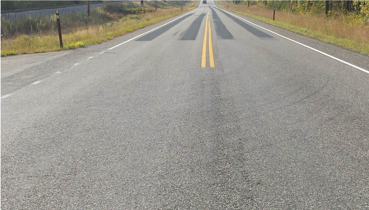
Figure 46. ER7, SR20, two years after installation. No change in chip seal.
