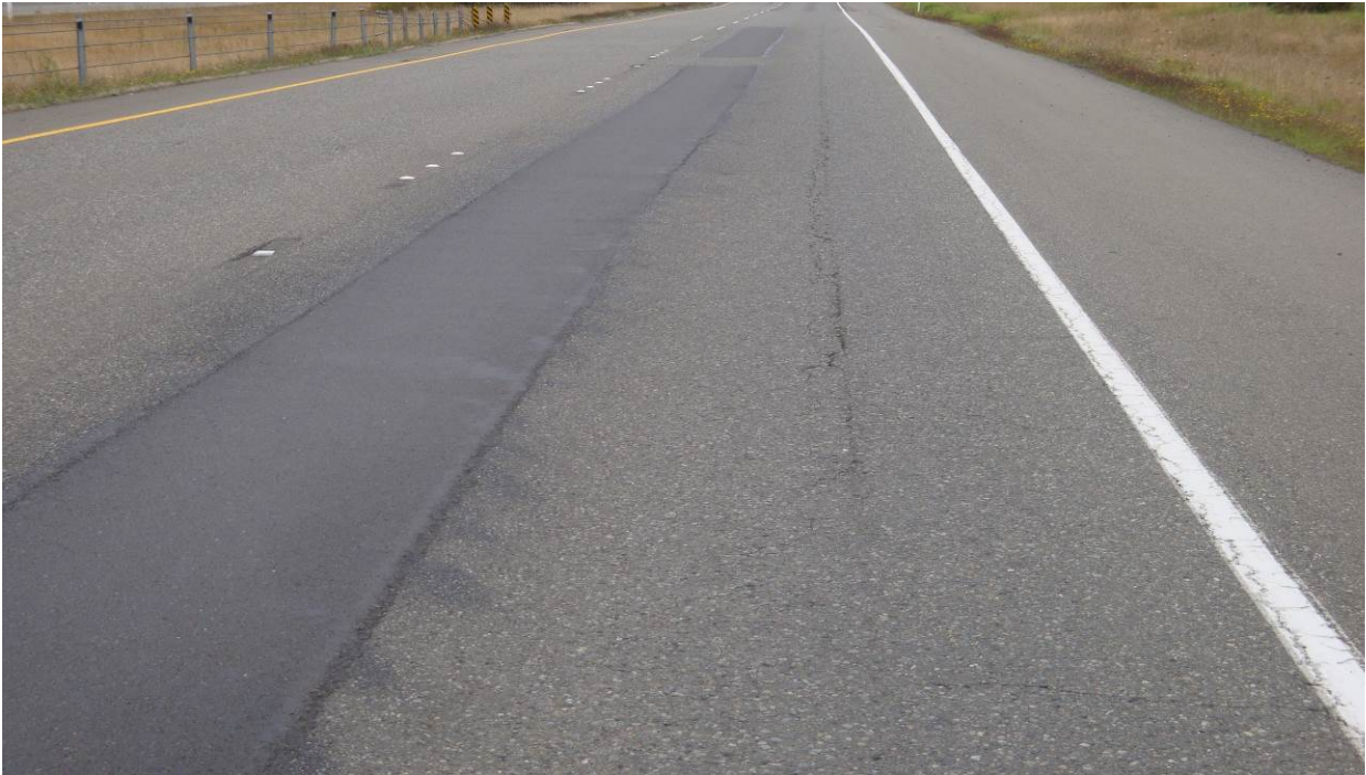
Figure 79. OR2, SR8, one year after installation. Dig out patch looks excellent.
