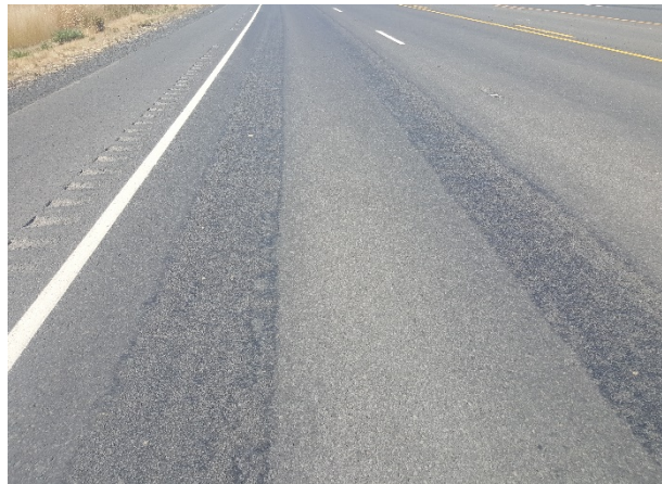
Figure 42. ER40, US270, Good, age 26 months. Loss of chips in both wheel paths.
