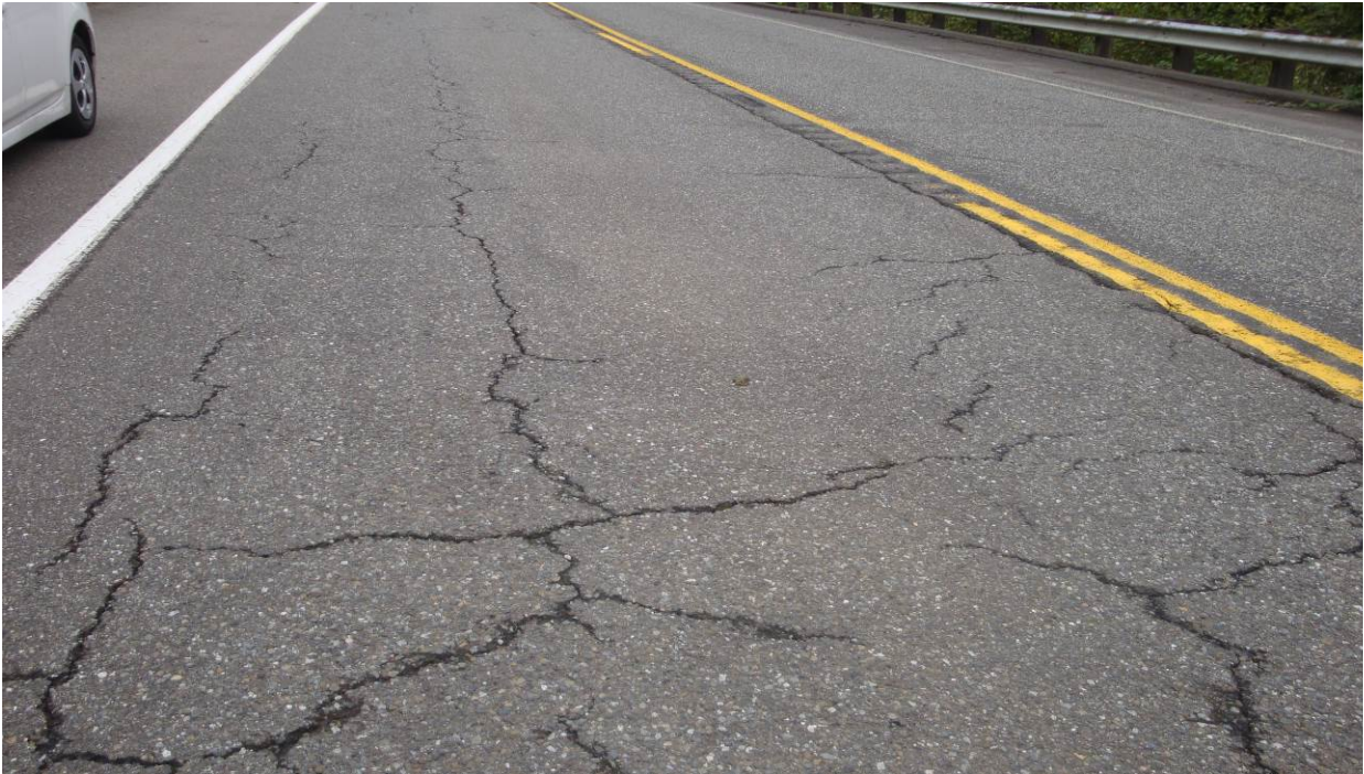
Figure 130. OR3a, SR101, one year after the other sections were treated. Cracking looks severe due to moisture in the cracks.
