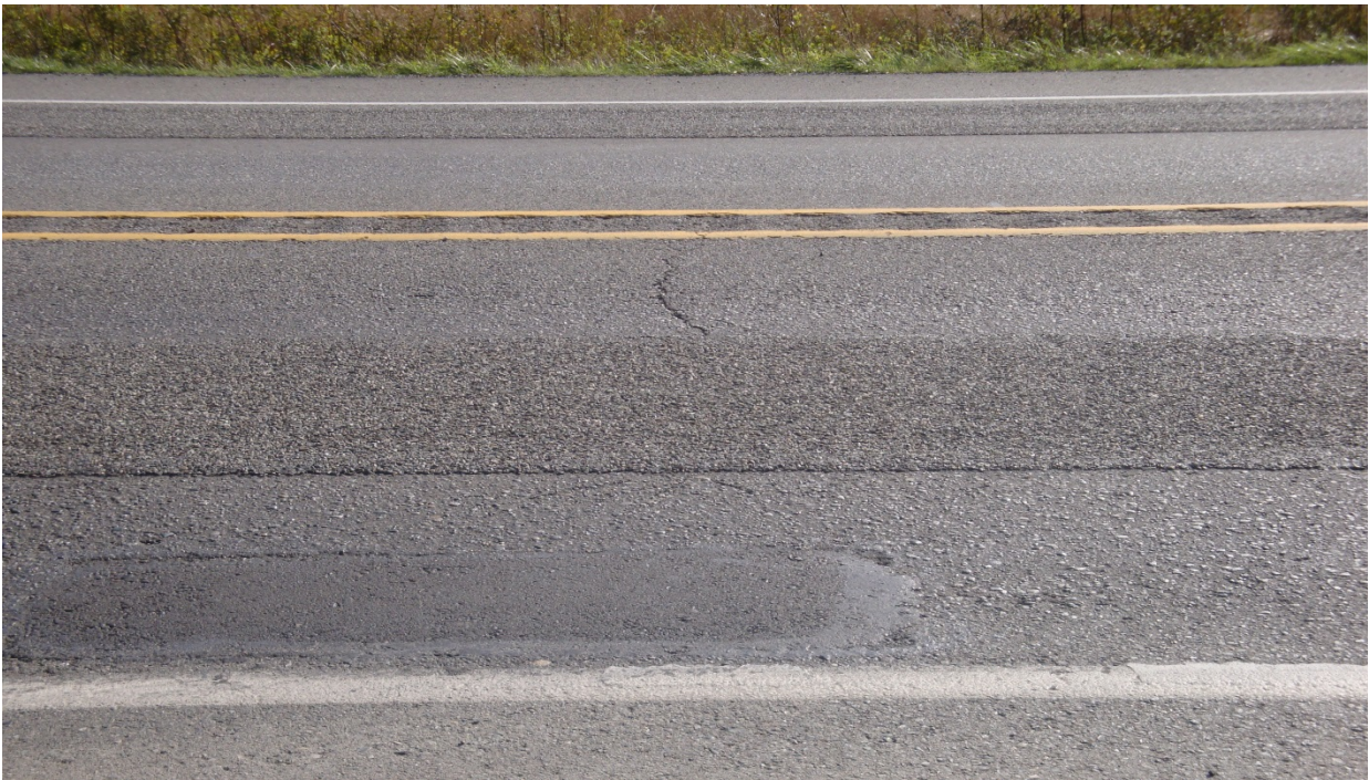
Figure 33. OR12, SR20, immediately after installation. Wheel path chip seal patching was well constructed.
