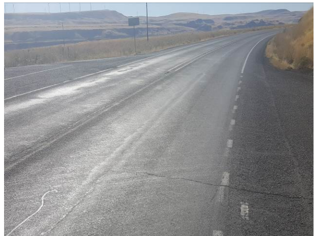
Figure 103. SW1a, SR14, Poor, age 62 months. Transverse and longitudinal reflection cracking and flushing noted at 12 months after installation. Potholes developed at 50 months.
