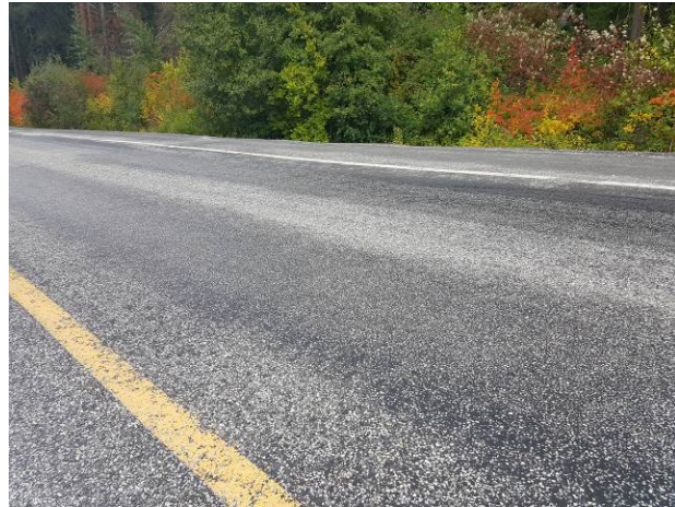
Figure 105. NC3, SR207, Good, age 38 months. Dig out patches flushing through the chip seal after 12 months. This is actually a HBST with 100% embedment in the wheel paths.
