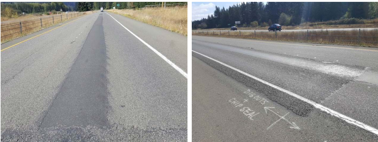
Figure 136. OR2 and OR2a on SR8. OR2 received dig outs and OR2a received dig outs and a chip seal. Photos are from 2016, both sections were milled and filled with HMA in 2017
