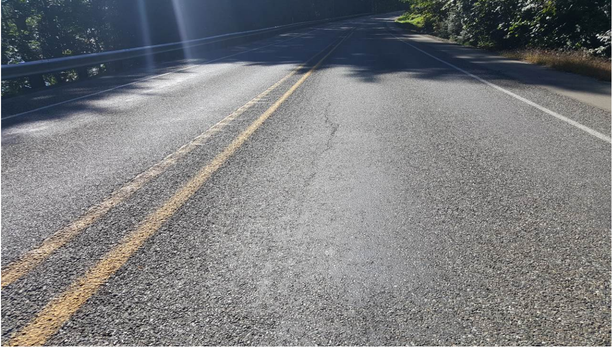
Figure 28. OR1b, SR101, four years after installation. Longitudinal crack condition is about the same, slight rutting and flushing in the wheel paths.
