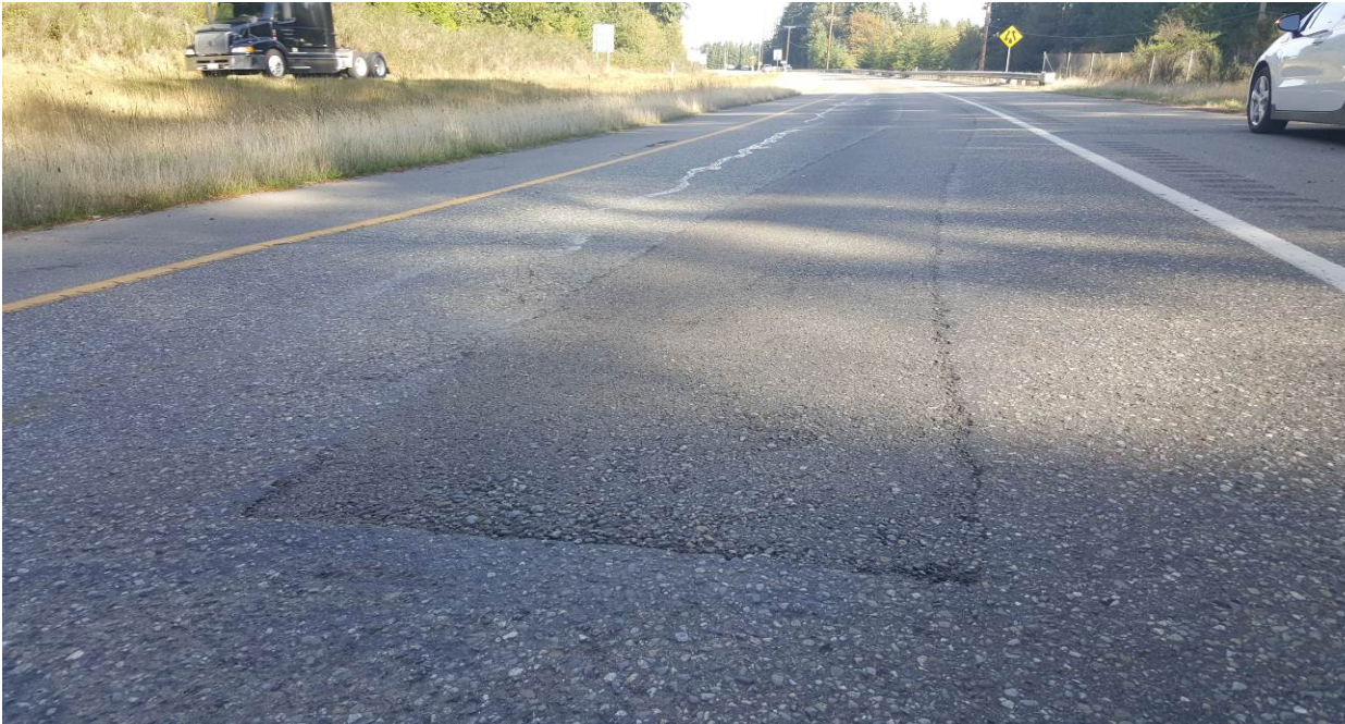
Figure 97. OR4, SR3, two years after installation. No change in dig out patch or crack sealing.
