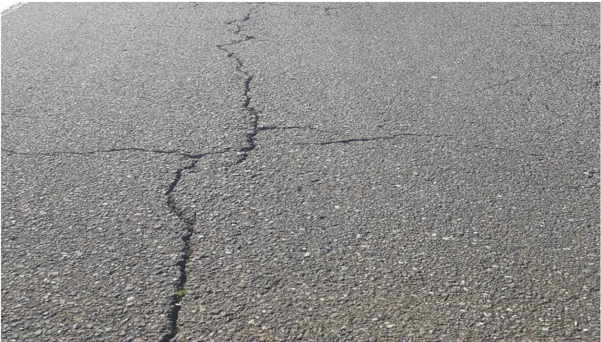
Figure 133. OR3a, SR101, four years after the other sections were treated. Cracks are wide and beginning to spall.
