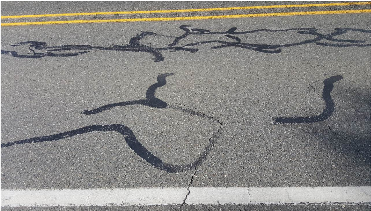
Figure 17. OR1, SR101, three years after installation. There is not much change from year one.
