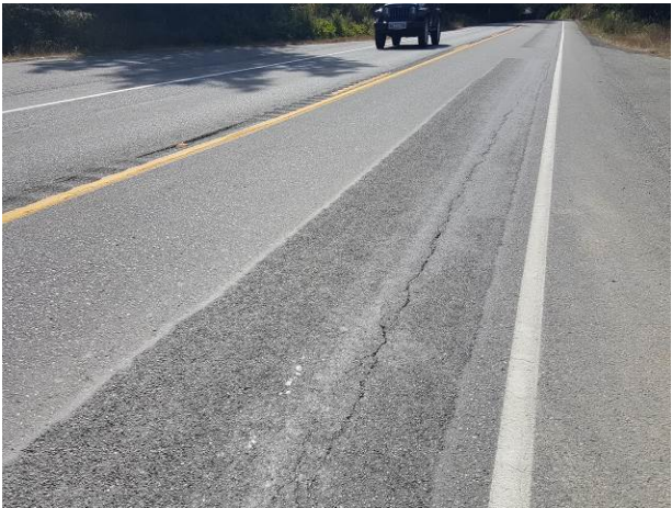
Figure 30. OR12, SR20, Good, age 49 months. Longitudinal reflection crack and flushing noted at 10 months.
