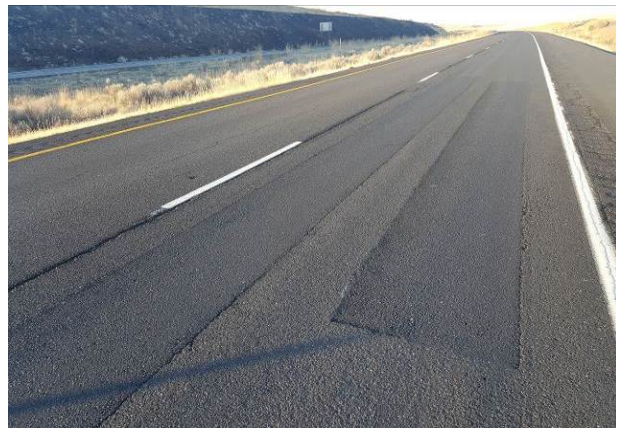
Figure 69. ER17, SR395, Good, age 26 months. Transverse reflection cracking in 2017.
