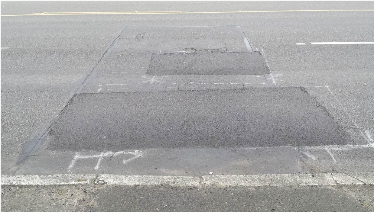
Figure 86. OR5, SR7, one year after installation. No change in the dig out patches.
