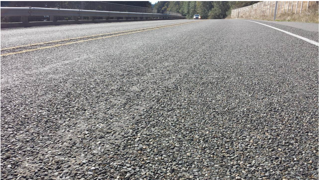
Figure 52. OR1a, SR101, two years after installation. Shadowing of the sealed cracks visible.
