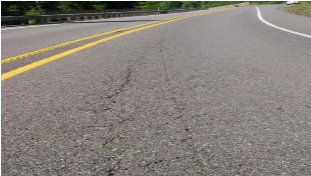
Figure 50. OR1a, SR101, prior to treatment. Alligator and longitudinal cracking noted.
