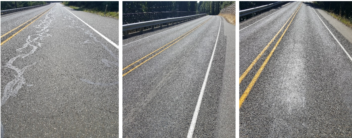
Figure 135. OR1, OR1a and OR1b on SR 101. OR1 has crack sealing, OR1a has crack sealing and chip sealing, and OR1b has a chip seal with no crack sealing. Photos from 2017.
