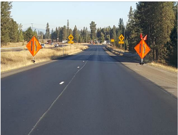
Figure 90. ER1, US2, Poor, 62 months. Additional dig outs and crack sealing done in 2015. HMA grind/inlay in 2017, C9124.
