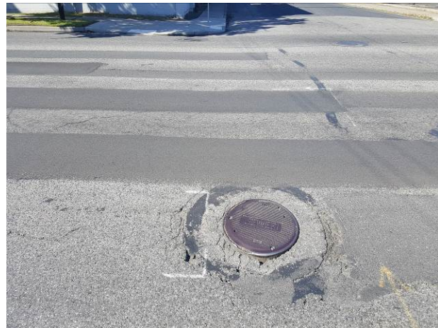
Figure 59. ER4, US2, Fair, age 62 months. Additional dig outs installed in 2013 and 2015. Note different colors of dig out patches done in different years. HMA grind/inlay scheduled in 2018, C9187
