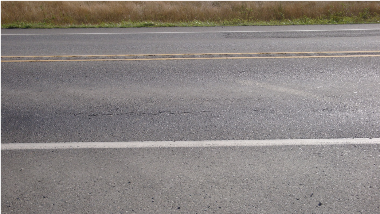
Figure 32. OR12, SR20, prior to treatment. Longitudinal and alligator cracking present in the wheel paths.
