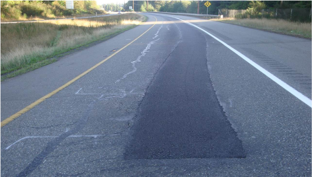
Figure 95. OR4, SR3, a few months after installation. Crack sealing looks good, dig out patches appear under filled in spots.
