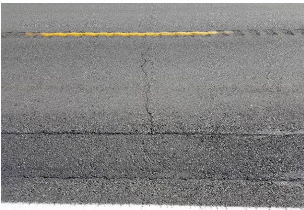
Figure 64. OR11, SR20, Good, age 49 months. Raveling of patch edges noted at 25 months.
