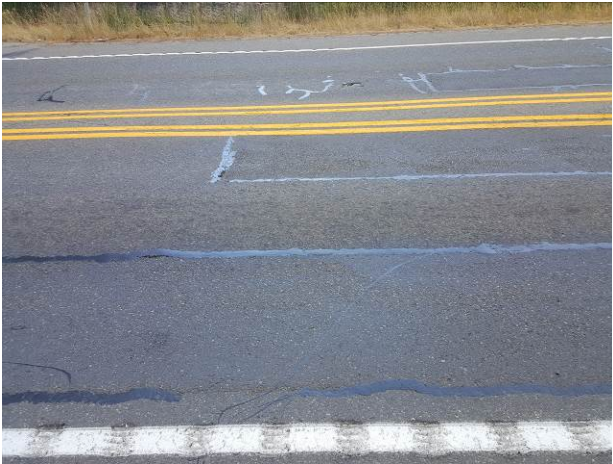
Figure 92. OR27, SR307, Good, age 26 months. Dig out patches and crack sealing in excellent condition.
