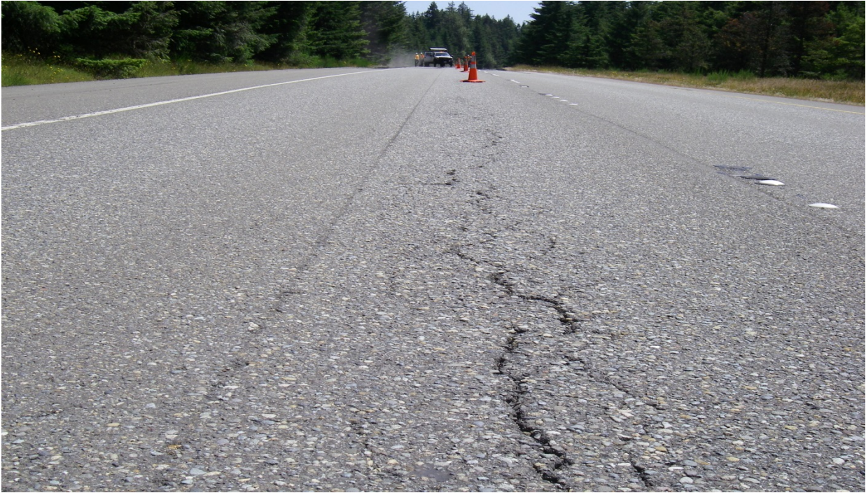
Figure 78. OR2, SR8, prior to treatment. Alligator cracking in the left wheel path. This is not the same location as the following photos which had alligator cracking in both wheel paths.
