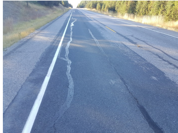
Figure 113. ER9a, SR395, Good, age 37 months. Transverse and longitudinal cracking reflecting through the patch at 13 months.
