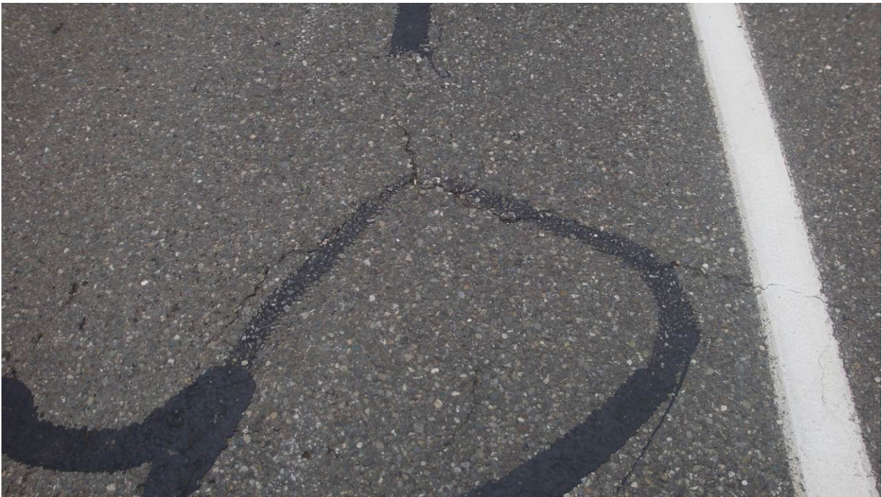
Figure 15. OR1, SR101, one year after installation. Slight wear of sealant over banding.
