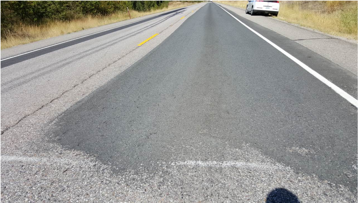
Figure 122. ER9a, SR395, one year after installation in 2014. Some wear of the blade patch at each end. Transverse cracks reflected through the blade patch after only one year.
