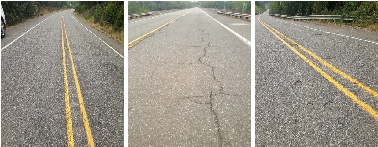
Figure 137. OR3, OR3a and OR3b on SR101. OR3 received dig outs and a chip seal, OR3a no treatment and OR3b a chip seal with no dig outs. Photos from 2017.
