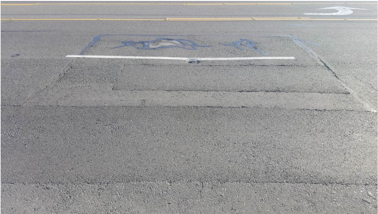
Figure 89. OR5, SR7, four years after installation. No change in the dig out patches. Different location in the same test site.
