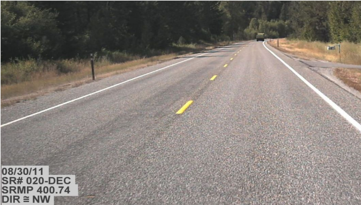
Figure 43. ER7, SR20, prior to treatment. Rutting is visible in the wheel paths.
