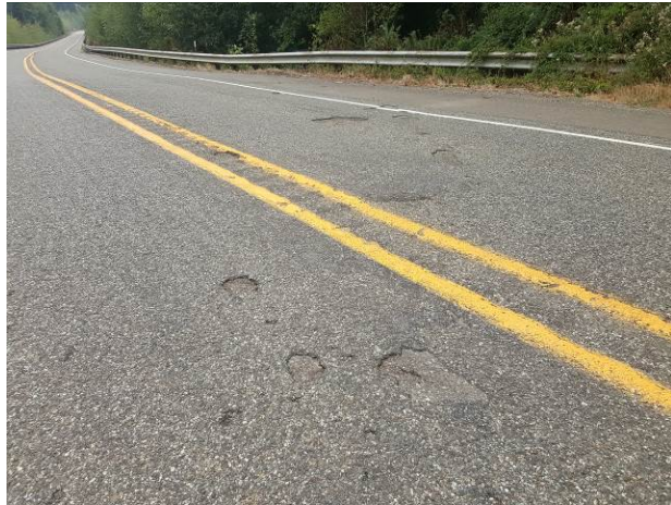
Figure 21. OR3b, SR101, Poor, age 62 months. Delamination and spalling noted.
