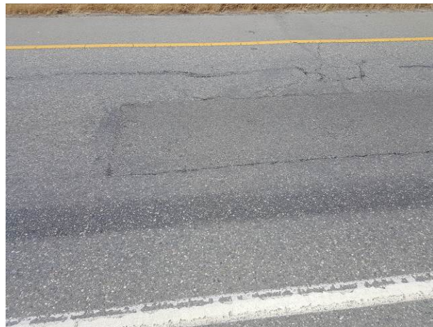
Figure 91. OR4, SR3, Good, age 50 months. Dig out patches and crack sealing in excellent condition.
