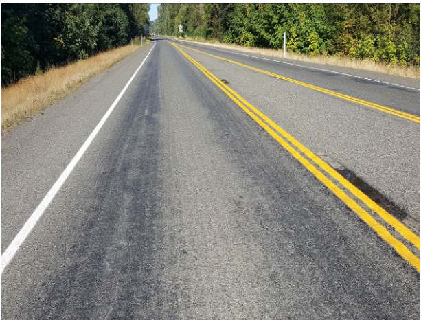
Figure 22. OR16, SR16, Good, age 49 months. Longitudinal cracking and pumping of fines noted at 14 months. Alligator cracking noted at 49 months.
