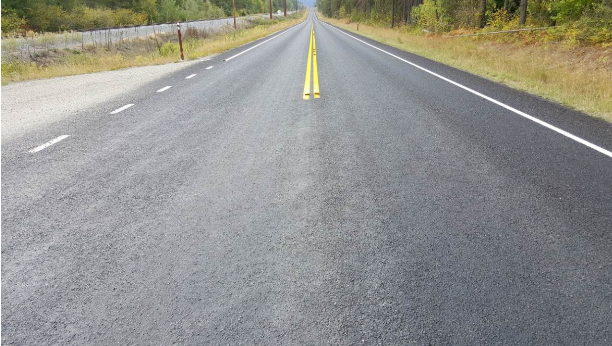
Figure 47. ER7, SR20, three years after installation. Full lane chip seal installed under Contract 8728, US 2 ET AL 2015 Eastern Region Chip Seal.
