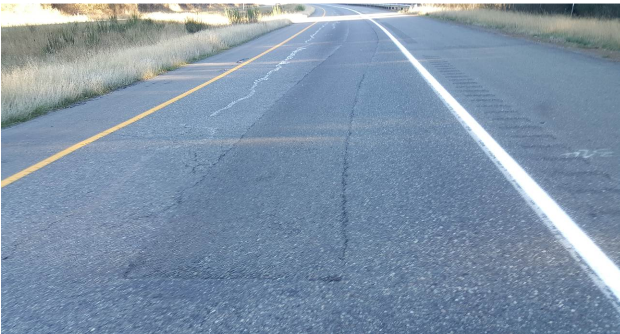
Figure 98. OR4, SR3, three years after installation. No change in dig out patch or crack sealing.
