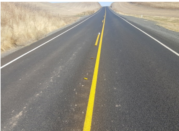
Figure 114. ER20, SR272, Good, age 24 months. Transverse crack reflecting through the patch. HMA grind/inlay in 2017, 9031.
