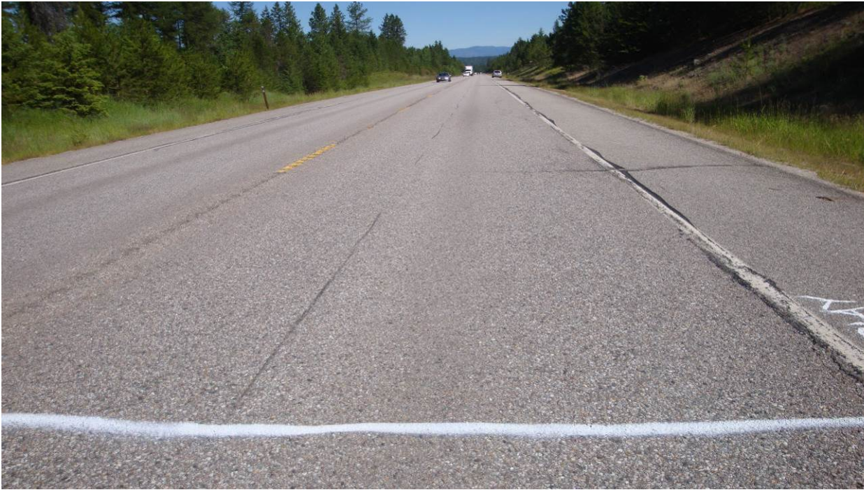
Figure 120. ER9a, SR395, prior to treatment. Longitudinal, transverse and alligator cracking.
