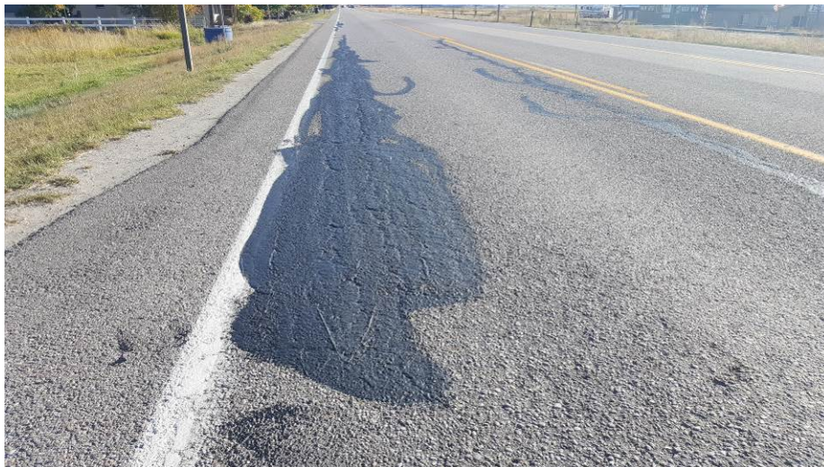
Figure 139. Excessive crack sealant used on alligator cracking on SR 20. (November 2016)
