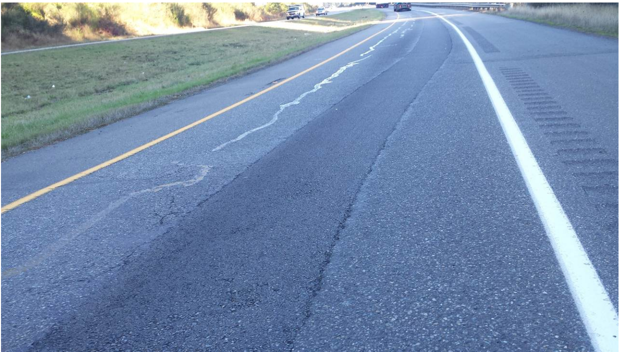
Figure 96. OR4, SR3, one year after installation. Dig out patch and crack sealing look unchanged.
