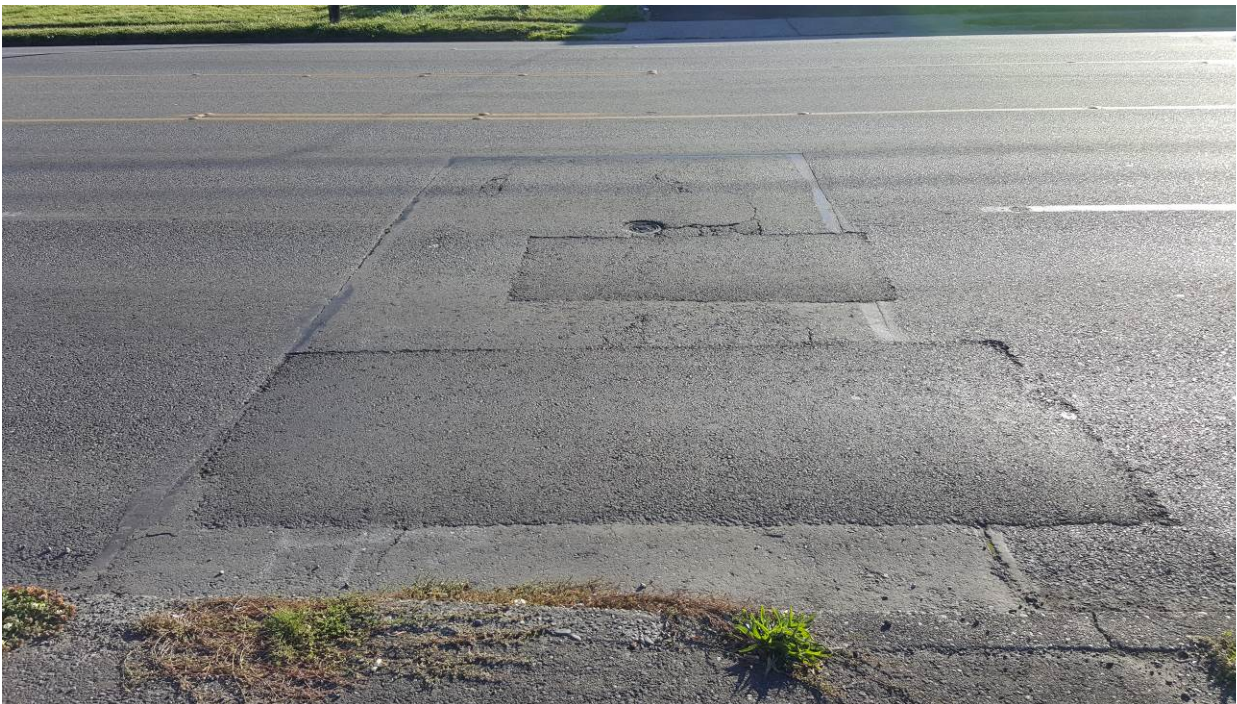
Figure 87. OR5, SR7, two years after installation. No change in the dig out patches.
