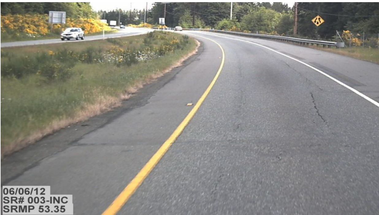
Figure 94. OR4, SR3, prior to treatment. Longitudinal, transverse and alligator cracking.
