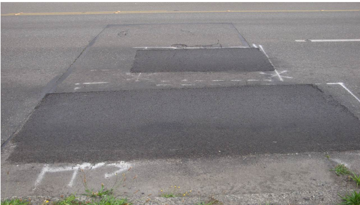
Figure 85. OR5, SR7, immediately after installation in 2013. Dig out patches look good. They appear to be related to utility cuts in original pavement.
