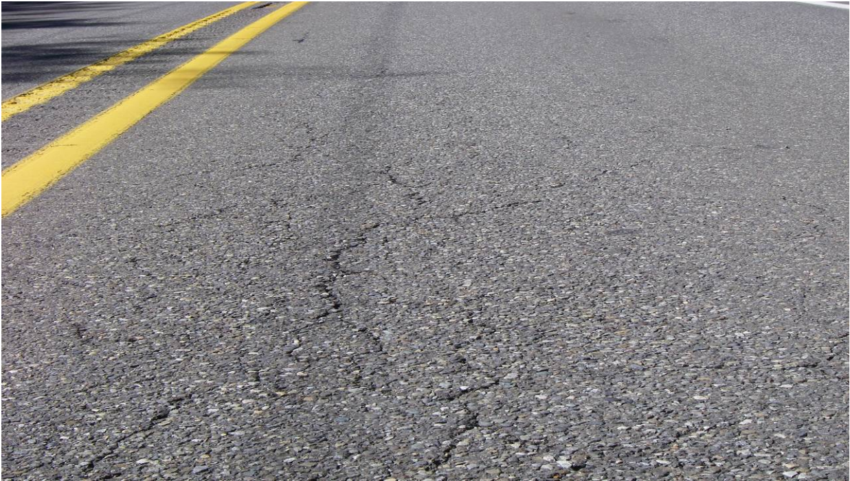
Figure 24. OR1b, SR101, prior to treatment. Alligator cracking was noted over the entire lane, but especially severe in the wheel paths.
