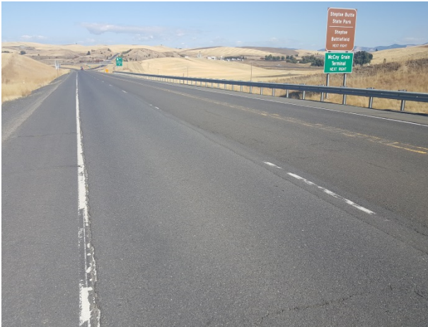
Figure 112. ER8, SR195, Good, are 39 months. Blade patch used to fill wheel path ruts. Additional patches placed in 2017.
