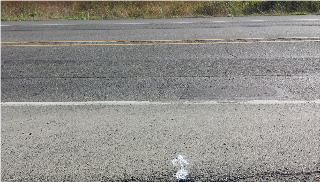
Figure 34. OR12, SR20, one year after installation. No change in the condition of the wheel path chip sealing.
