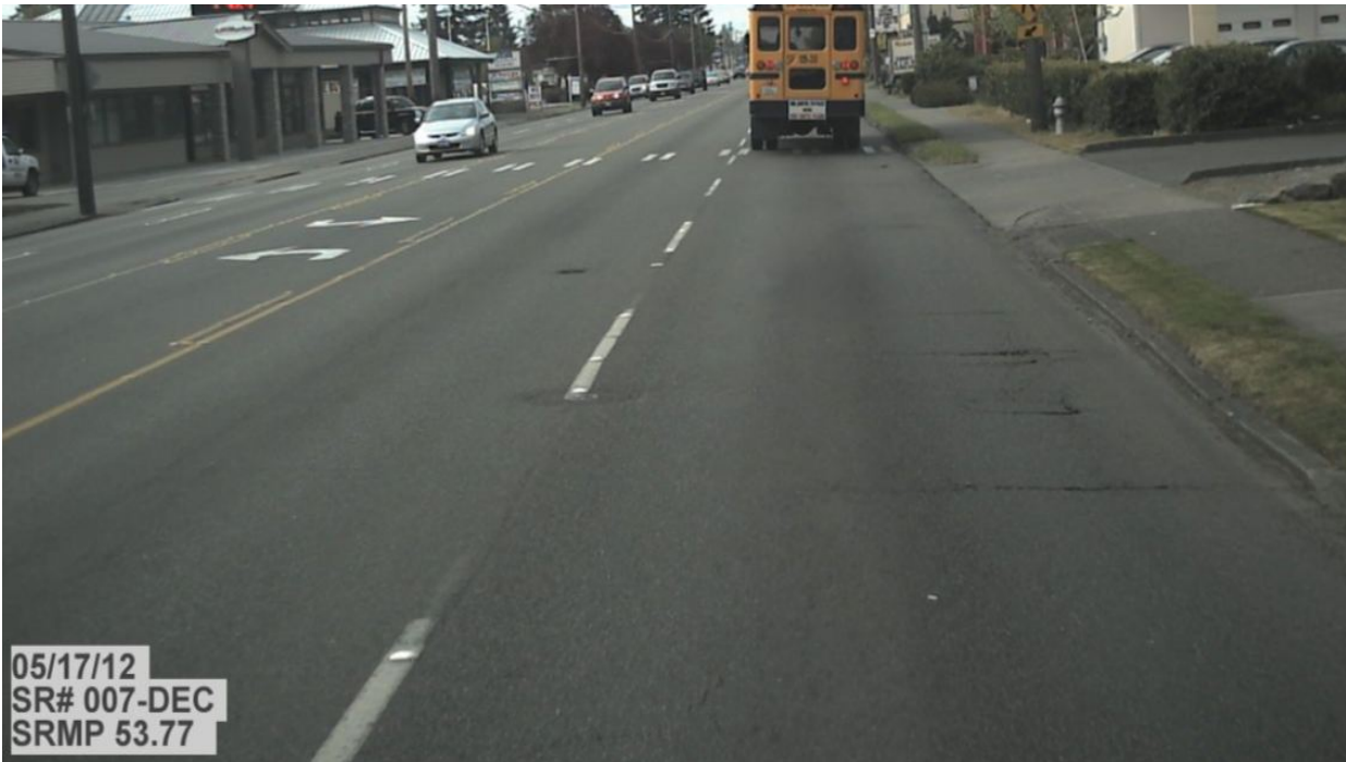
Figure 84. OR5, SR7, prior to treatment. Not at same location as following photos.
