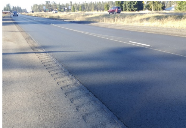
Figure 126. ER1a, US2, Poor category, age 62 months. Dig outs, crack sealing and patching were necessary to preserve the roadway. HMA grind/inlay in 2017, C9124.
