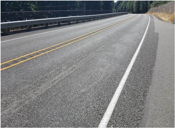
Figure 48. OR1a, SR101, Poor, age 62 months. Underlying crack sealant can be seen as shadowing.
