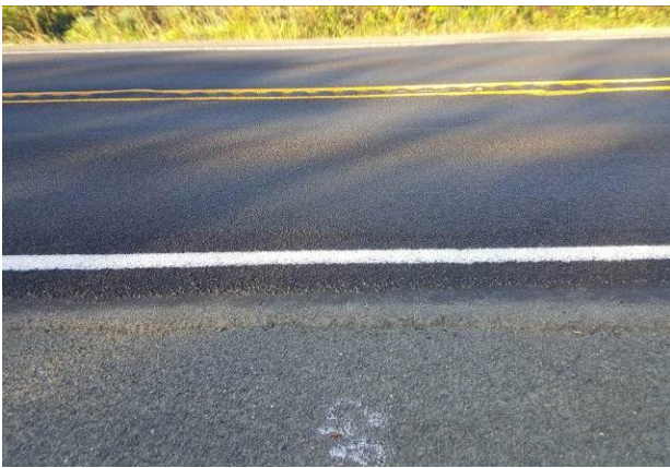
Figure 68. SW5, SR6, Good, are 38 months. More dig outs added in 2015. HMA grind/inlay in 2017, C9087.
