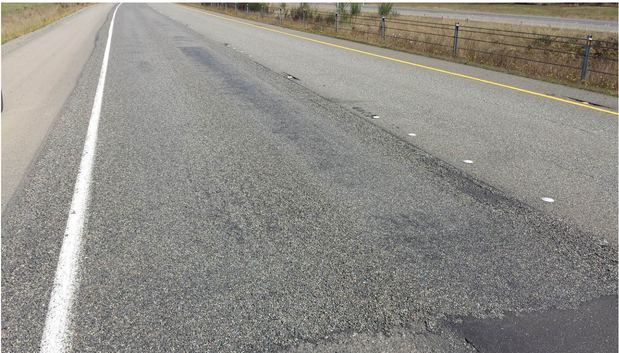
Figure 108. OR2a, SR8, two years after installation. Increased flushing in the wheel paths over the dig out patches.
