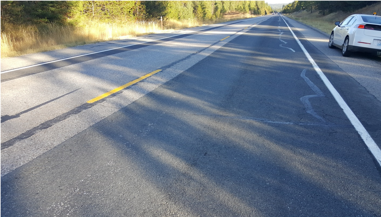
Figure 124. ER9a, SR395, three years after installation. Longitudinal reflection cracking has been sealed. Note slight flushing in the left wheel path.
