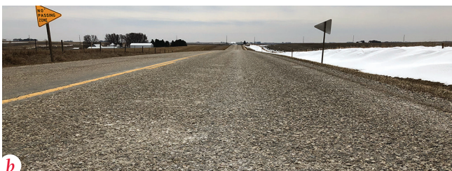
Otta seal surface appearance: (a) one day and (b) six months after construction
